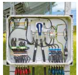
String Combiner Box
