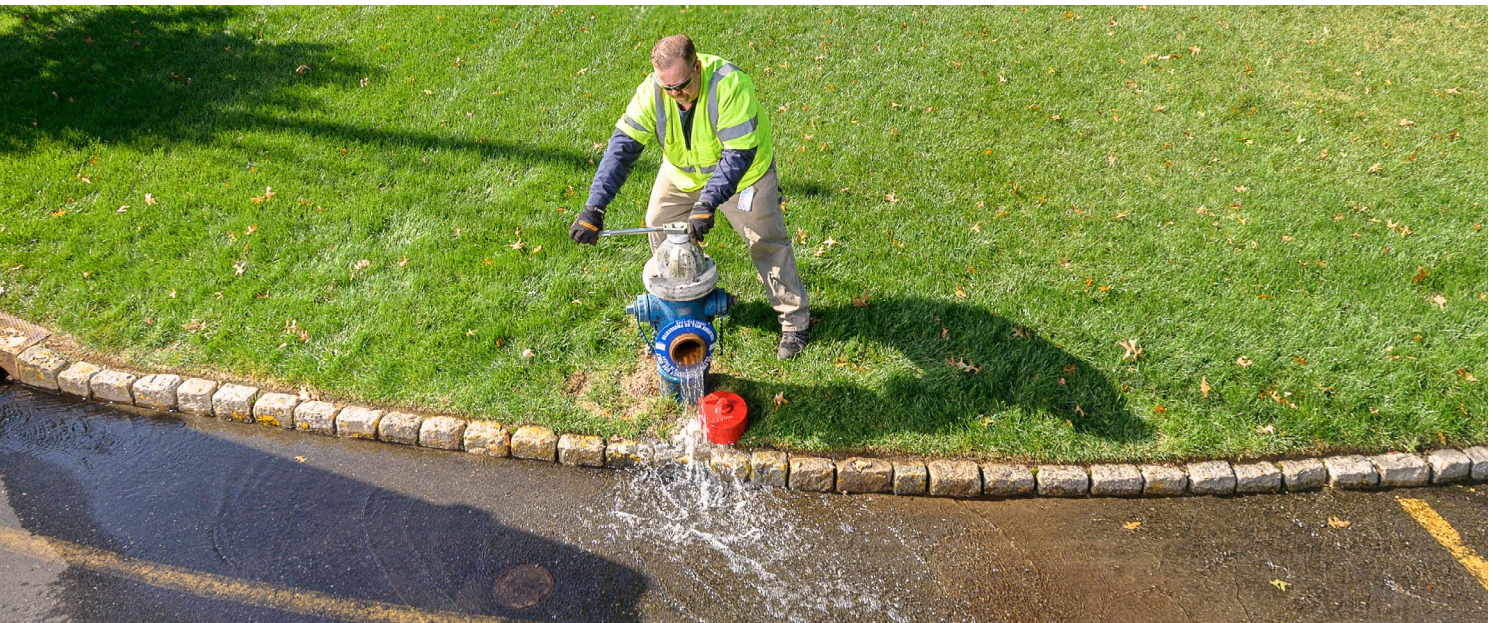
Flushing hydrants contributes to maintenance efficiencies in our service territories.
