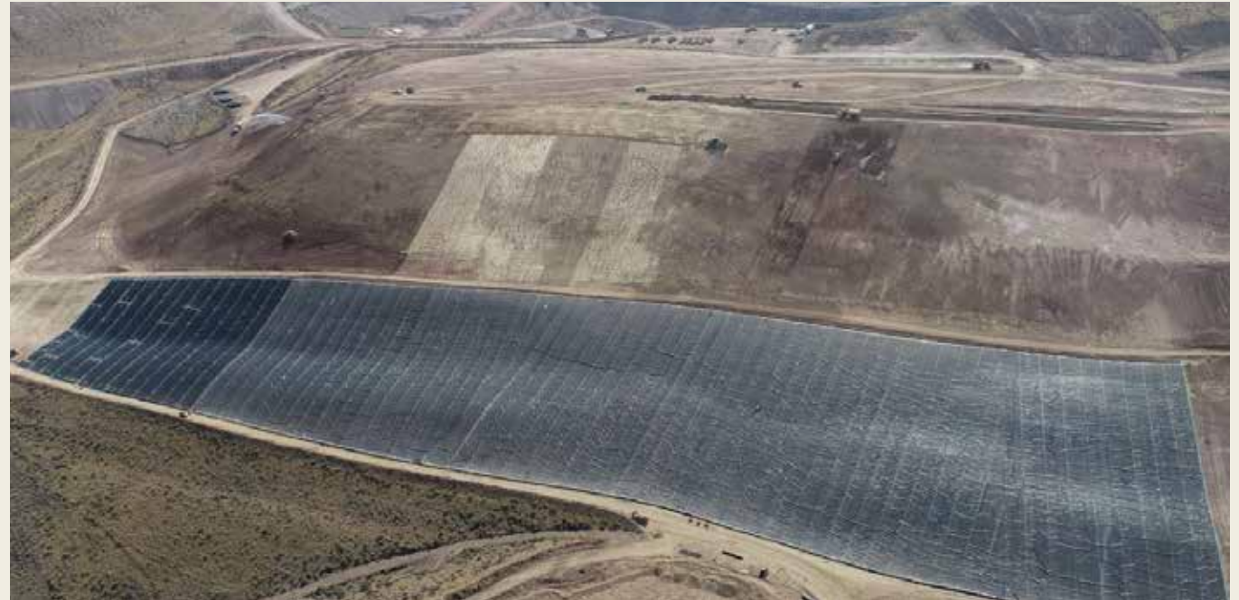
Rehabilitation activities at Rain, including the laying of the HDPE liner before the geotextile, cover material and topsoil deployment - NGM, USA.
