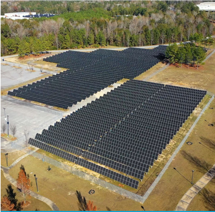
Aflac U.S.'s expanded solar array visual is available here .
