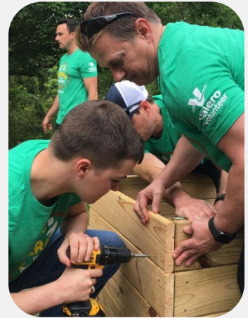
Texas City, Texas – As part of Earth Day activities, Valero volunteers helped build raised garden beds.
