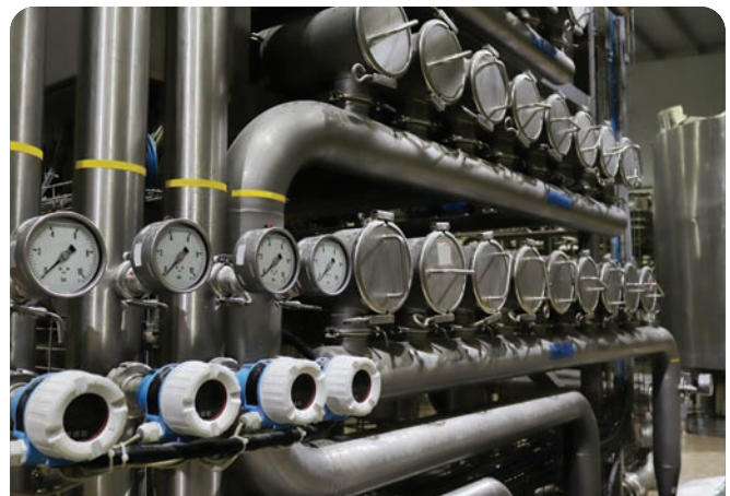
Our Penang, Malaysia facility uses water-efficient cooling systems and domestic water systems designed for reduced water consumption.
