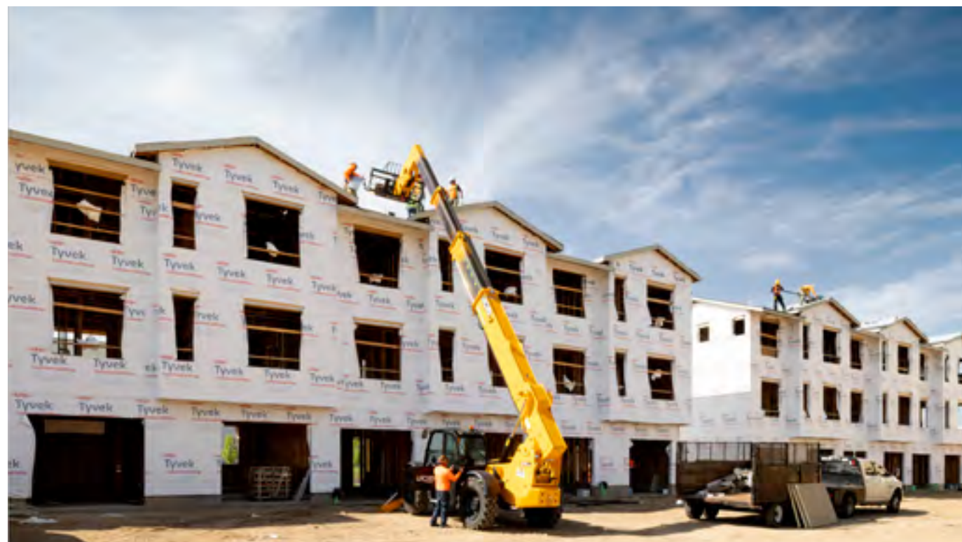
MAA Milepost 35 | Denver, CO | Construction started in 2022 on this garden style project built on a former airstrip in Denver, Colorado. Residents will enjoy access to an adjacent community park, additional amenities that support healthy lifestyles, and resource-efficient features in units and common areas.
