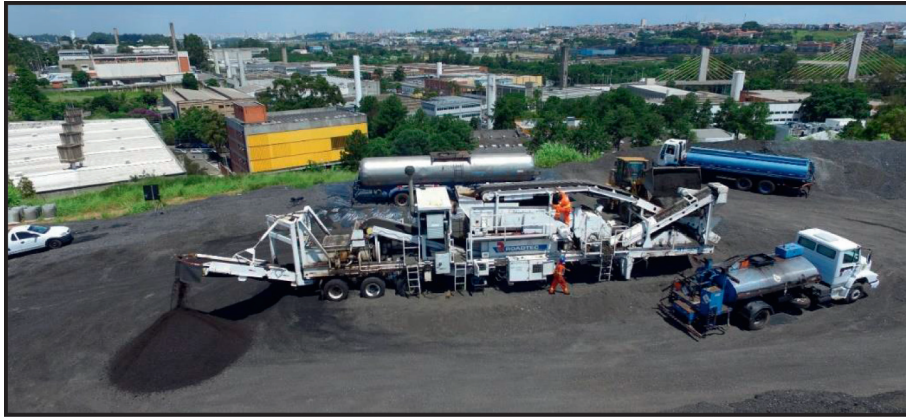
FIGURE 2: Cold in-place recycling train set up as a stationary cold central plant recycling.
