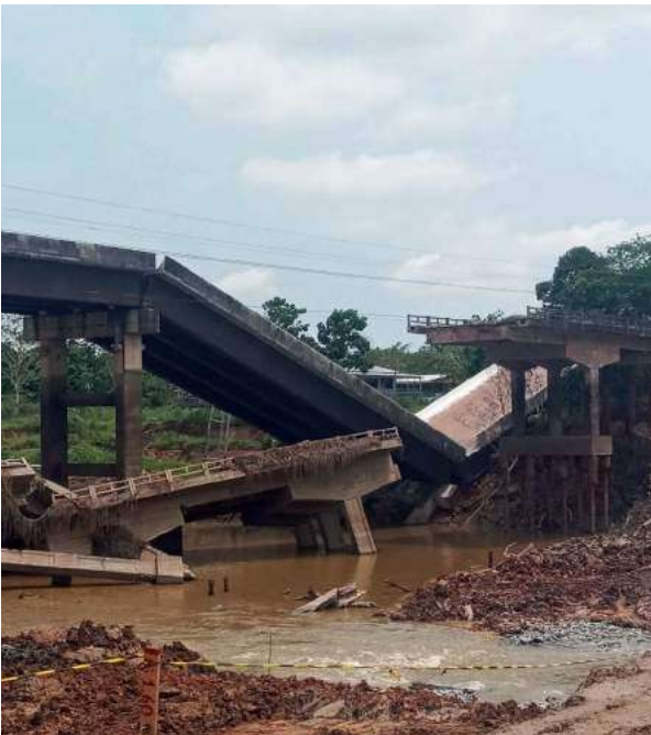
Figure 26. Bridge collapsed and lives lost due to lack of respect for the forest code and maintenance of Permanent Preservation Areas (APP).
