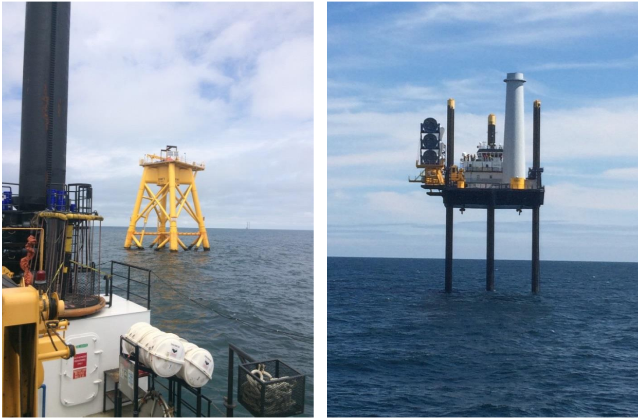
Figure 2. (L) Photo of a foundation base prior to WTG erection. (R) Photo of L/B Paul with tower section and blades.
