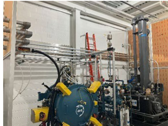
BWXT CVI Furnace Installed
