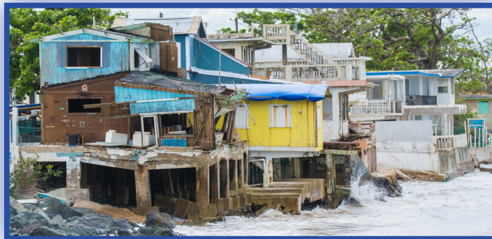
Seaside scene in Rincon, Puerto Rico after Hurricane
