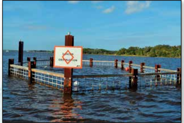
Jacksonville Electric Authority District II outfall manatee exclusion barrier. Photo Credit: T. Calleson, USFWS
