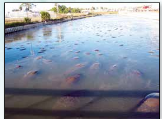
FPL Cape Canaveral Energy Center temporary heating system. Photo Credit: J. Lorne
