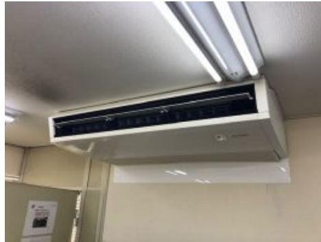
Update air-conditioning system
