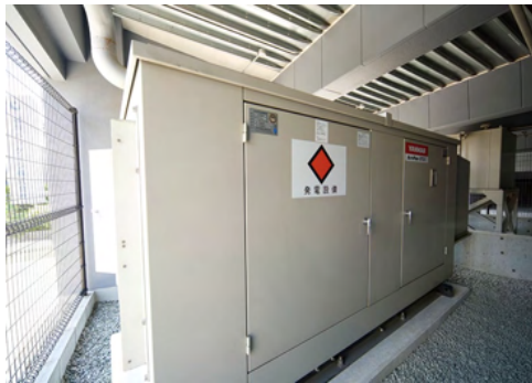
Installment of private power generators
