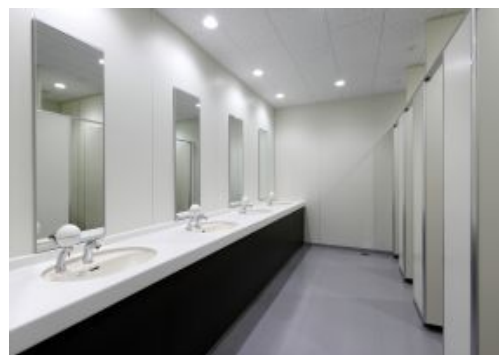
Installment of motion detected sensor
