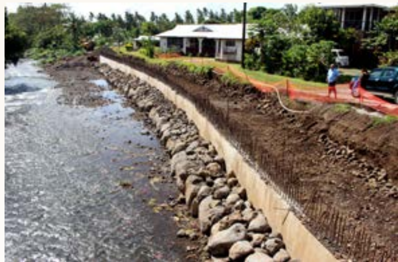
Vaisigano river wall. Photo: R.Setu
