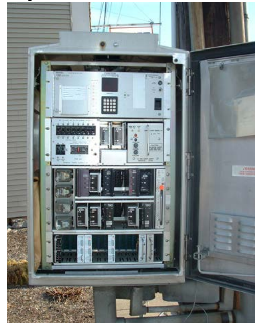
Figure 9-2: Computerized Signal Controller Cabinet at Intersection of Dixie Highway and Commonwealth in Kenton County
