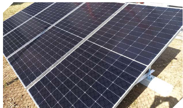
Photovoltaic panels producing electricity directly from sunlight to power our mobile base stations.
