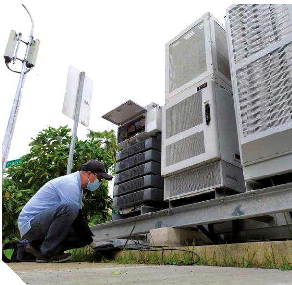
Engineer maintaining a mobile base station.
