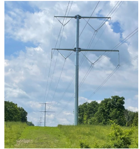
Figure 2-17. A double circuit rebuild for the New Your Energy Solution project with the 115 kV circuit on the left side of the tower and the 345 kV circuit on the right side of the tower.
