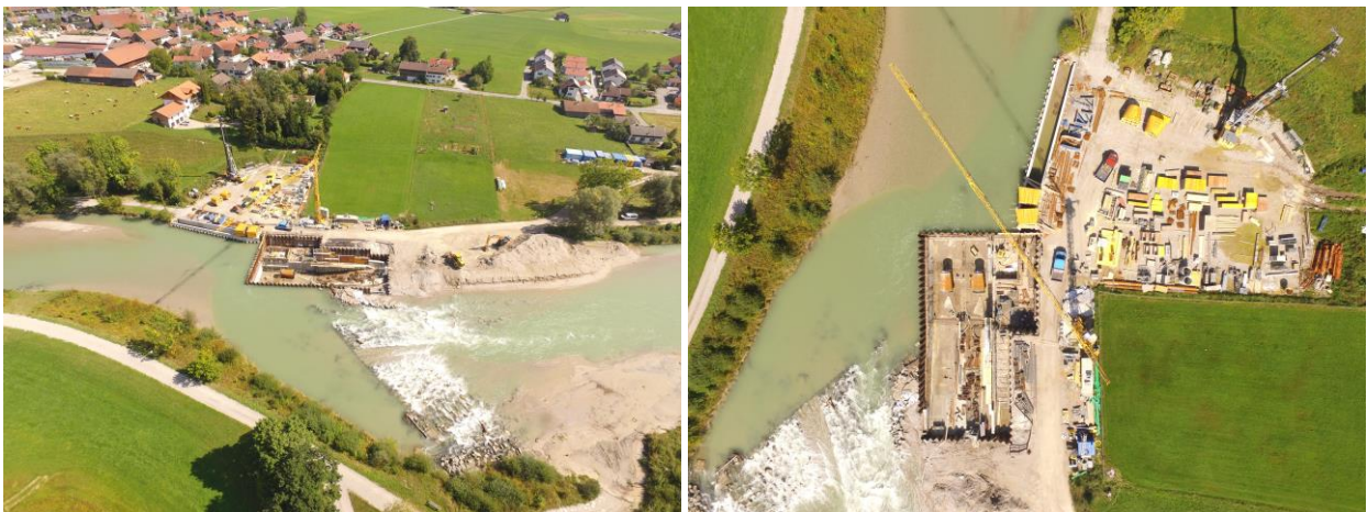
Figure 5: Construction pit at the orographically left bank. Suction pipes and parts of the vertical slot path are visible. (Ch. Bäck/TUM)
