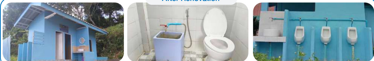
Pictures of bathrooms of a school in Galyani Vadhana District in Chiang Mai Province
