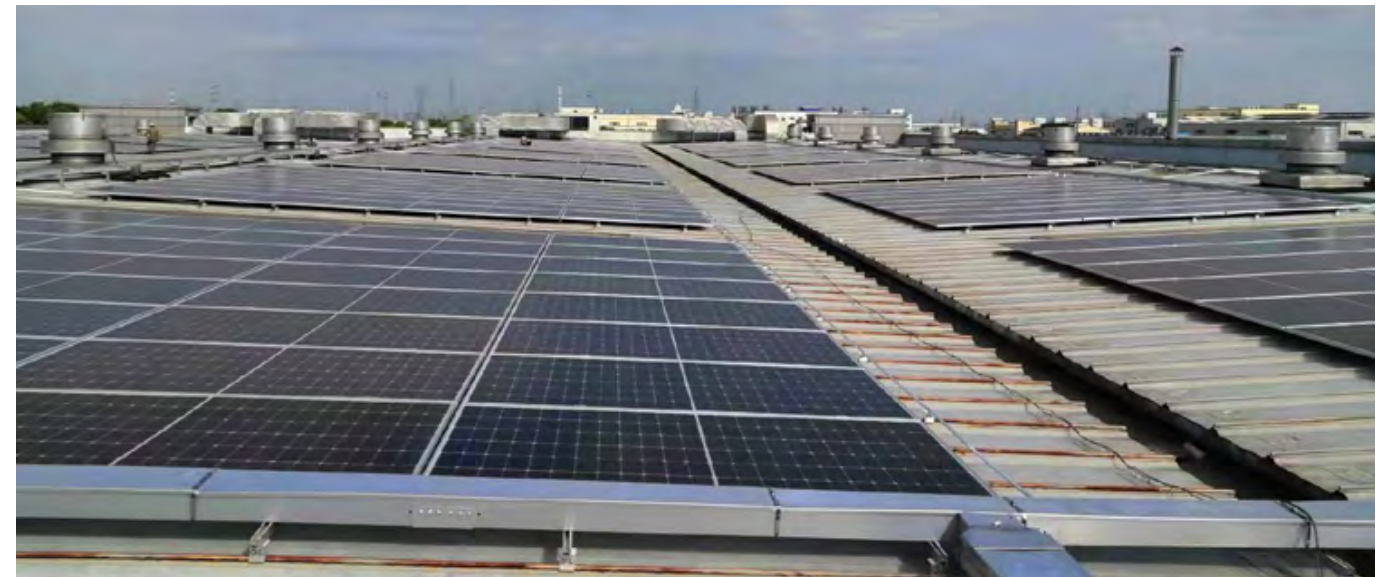
Photo from solar panel install at a Mold-Masters facility in Kunshan City, China.
