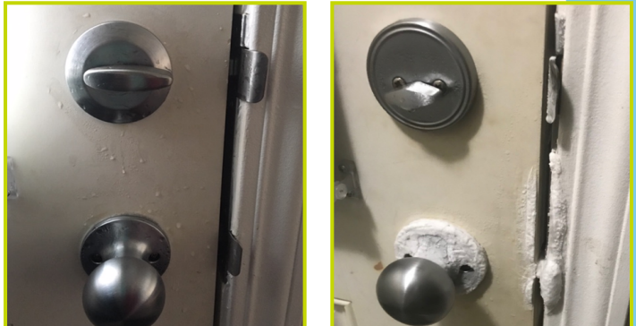
Ice inside your home can lead to material damage and mold. It can be an indicator of heat loss and high humidity.
