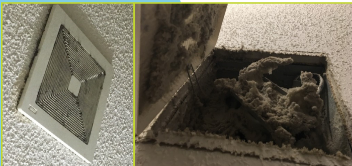
Do not let your vents look like these. This is a fire hazard and does not allow for proper ventilation.
