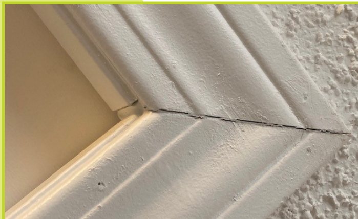
Photo of attic framing that needs latex caulk to avoid potential air leaks. Apply latex, paintable caulk to cracks.
