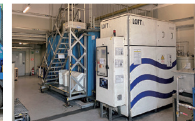
Liquid waste evaporation system
