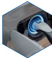
EV Charging Stations
