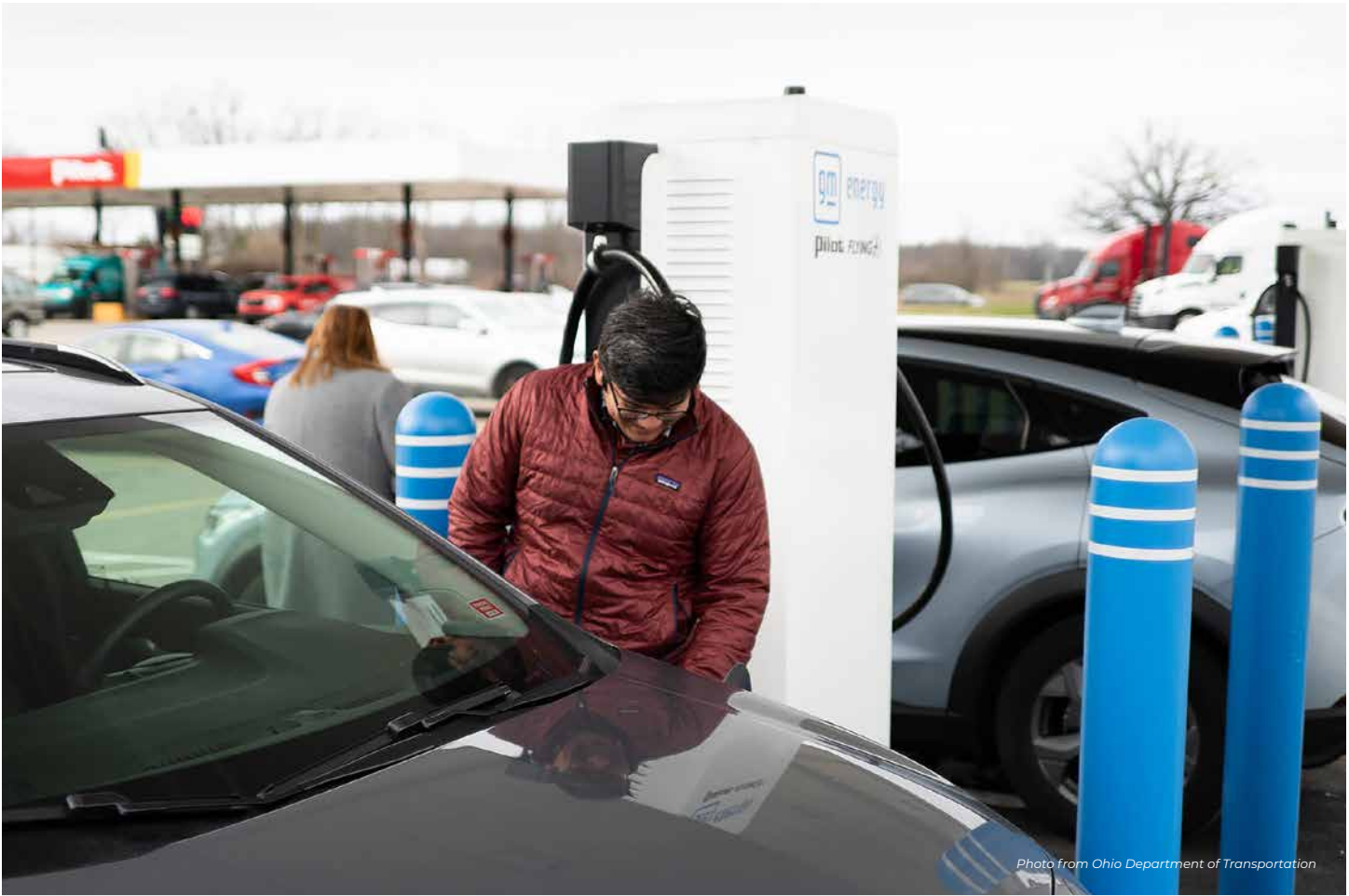
Concrete-filled bollards to help prevent vehicles from hitting charging equipment.
