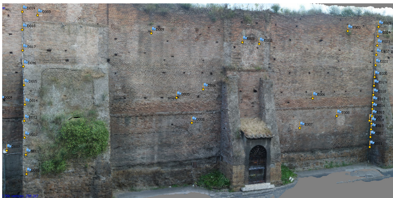
Figure 2. Topographic and Photogrammetric survey: portion of 3D model. The triangulated surface with topographic control points and colour information.
