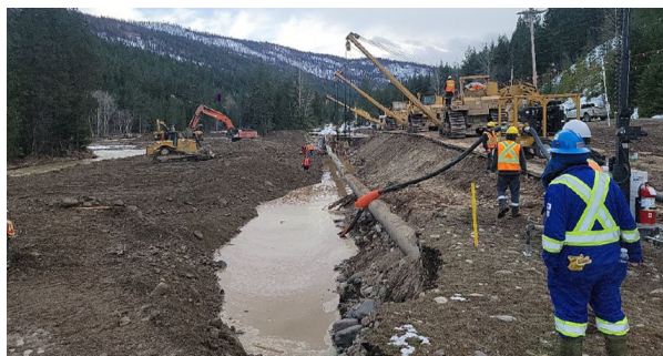
BELOW: Equipment supports the pipeline to allow crews to access the pipe after flooding in the Coldwater area and conduct inspection and repair.
