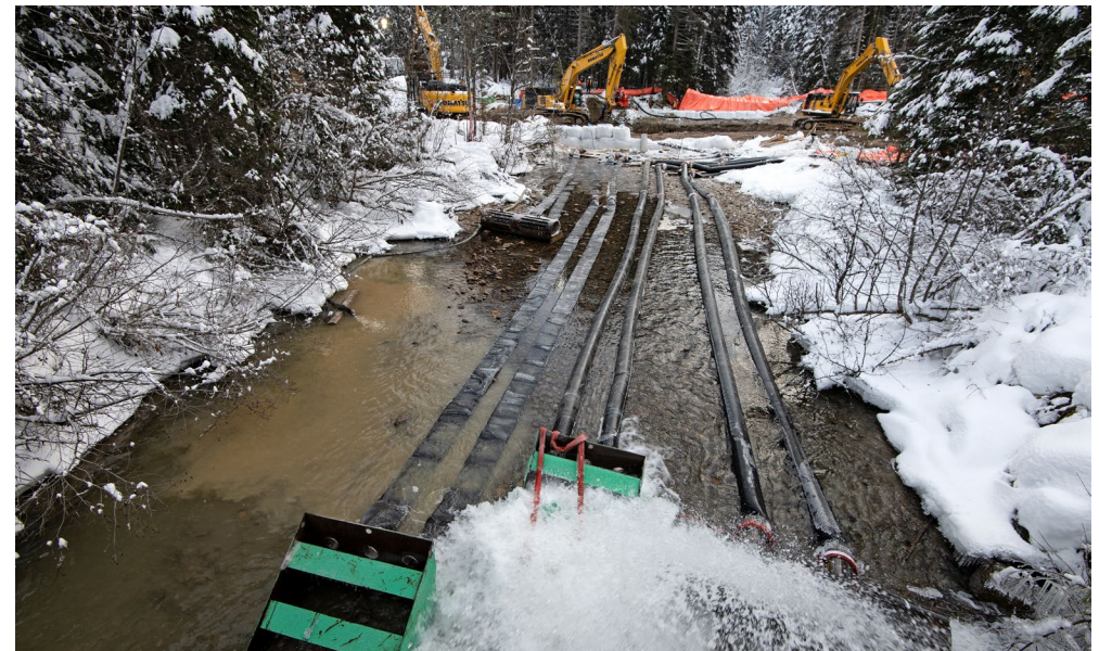
RIGHT: We inspect and monitor pipeline segments under bodies of water and conduct preventative replacements when needed. We carefully select appropriate construction methods given the sensitivity of the environment surrounding the pipe.
