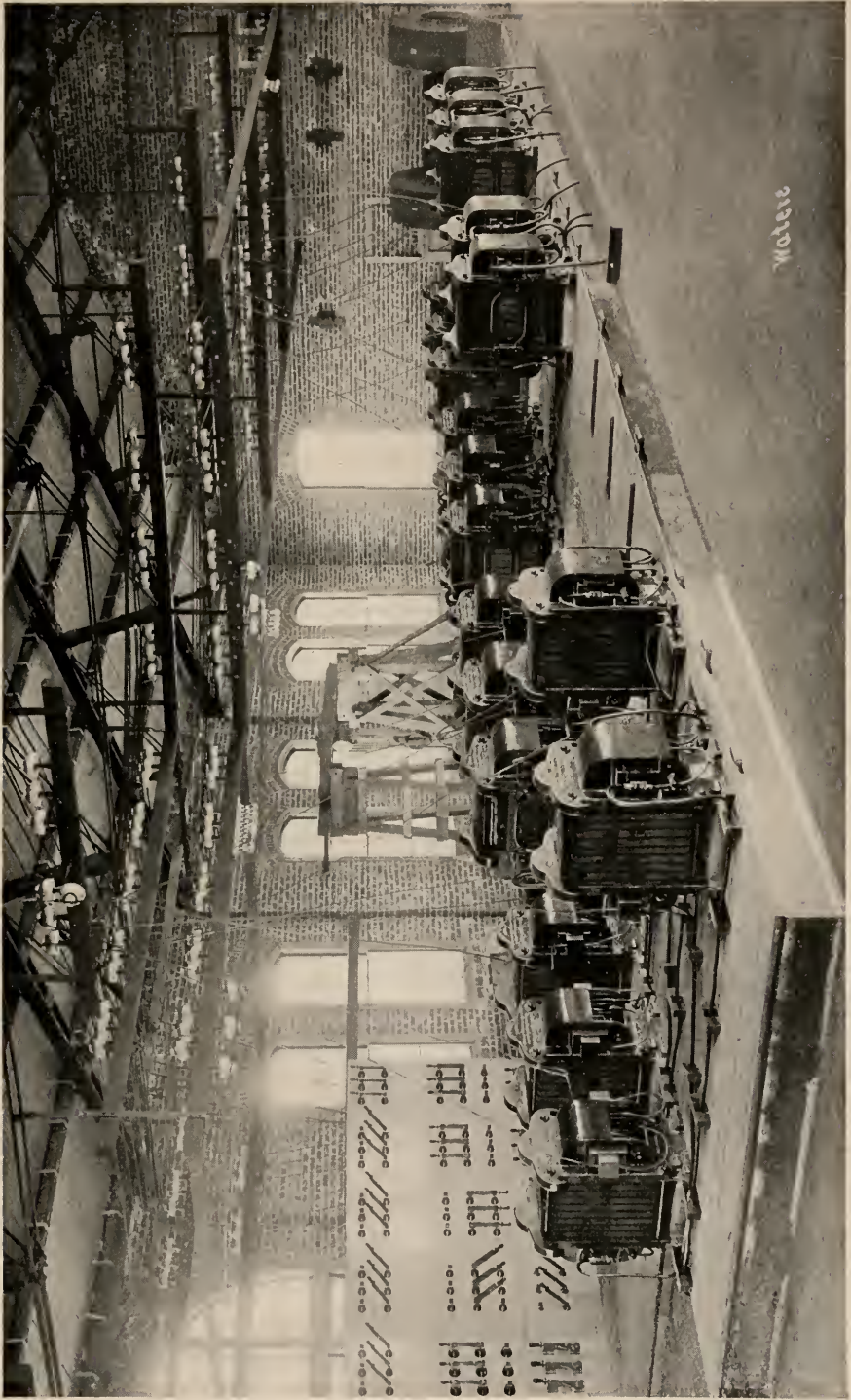
STEP-DOWN TRANSFORMERS IN SUBSTATION. FOLSOM-SACRAMENTO TRANSMISSION.
