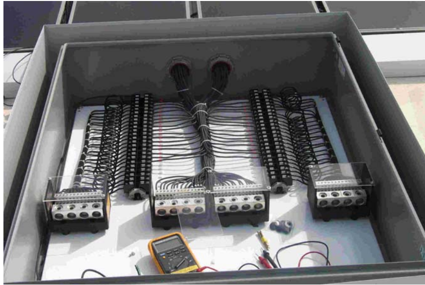
Figure 17. Photo of a wiring ‘combiner box’ housing the terminations for 17 high-voltage module-strings in a large array. In this case, each module string had twelve 150- W_p crystalline silicon modules connected in series.
