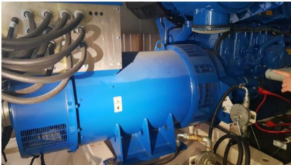
Water level, generator set – emergency power system. Photo: DNV
