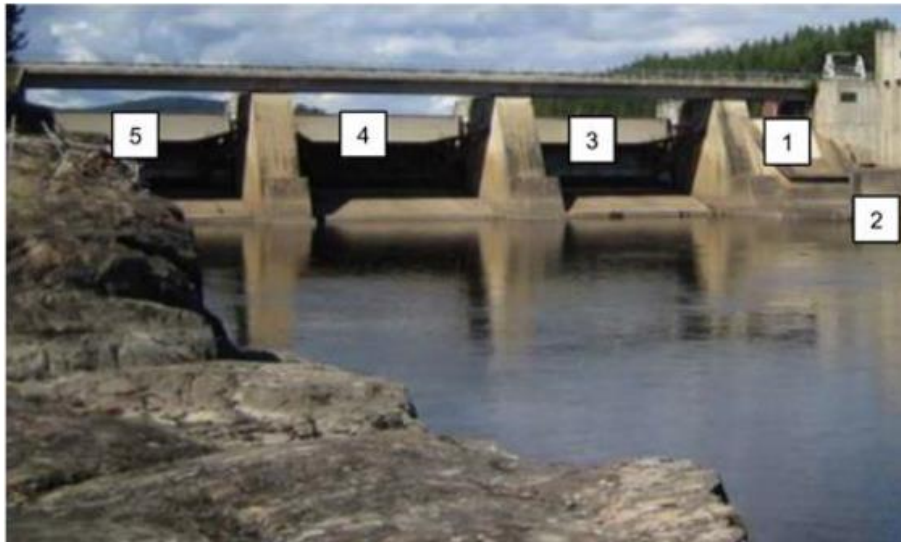
Numbering of gates according to the control system. Illustration photo: SWECO (does not match reassessment and inspection reports)
