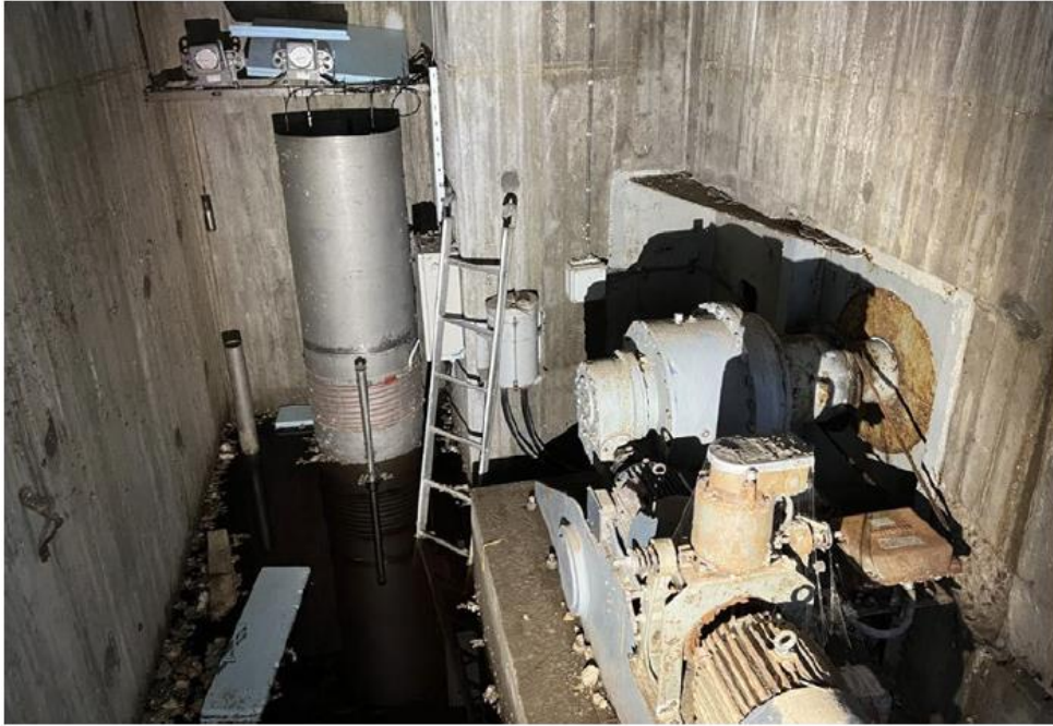
Photo 15: Gatehouse in pillar, with submerged machinery. The photo was taken after most of the water had been drained. Water can still be seen at the bottom of the gatehouse (Photo: DNV)
