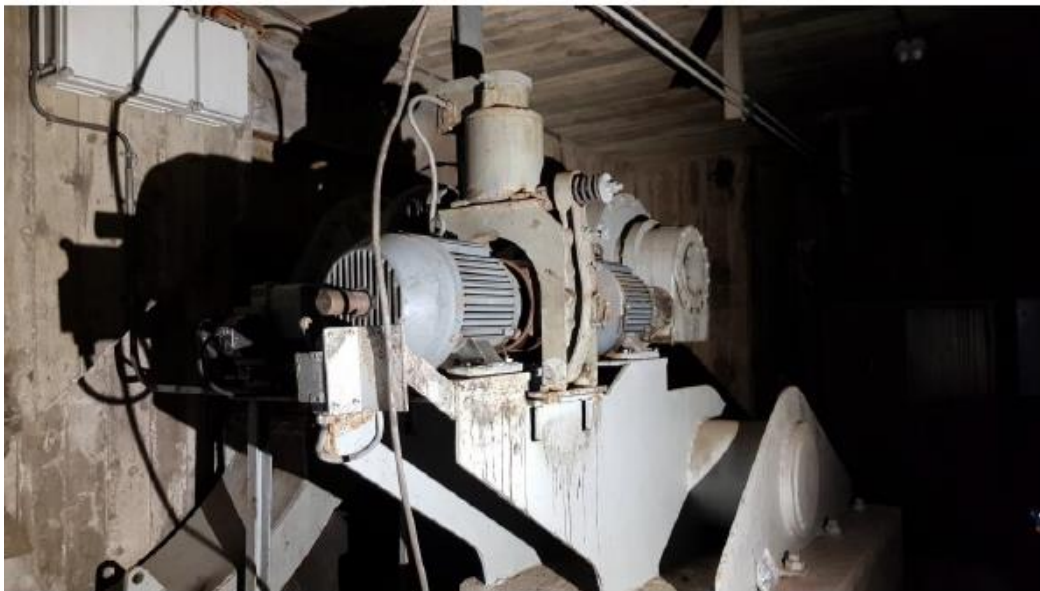
Chain works – floodgates. Photo: DNV
