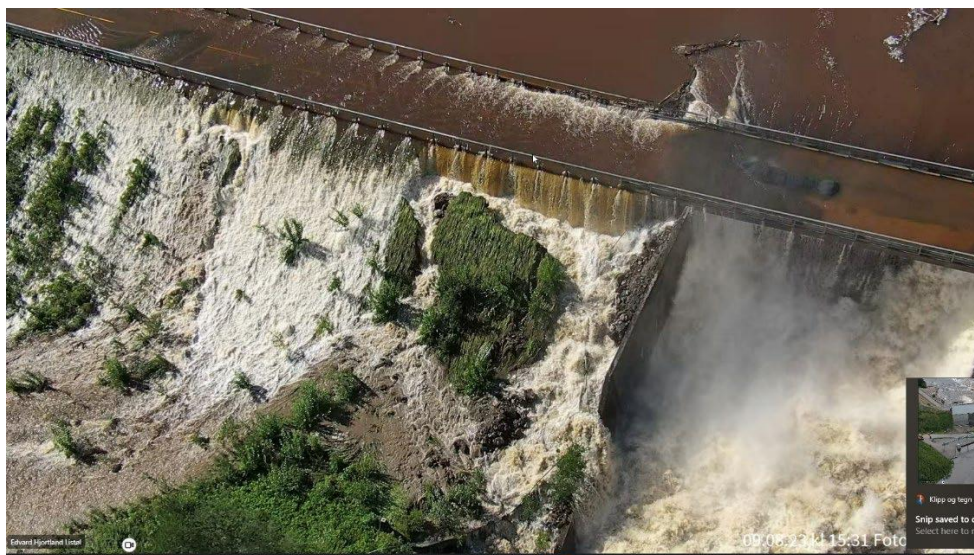
Photo 12: Overtopping of road bridge, embankment dam and gated dam at 15:31 (Photo: Police/Source NVE)
