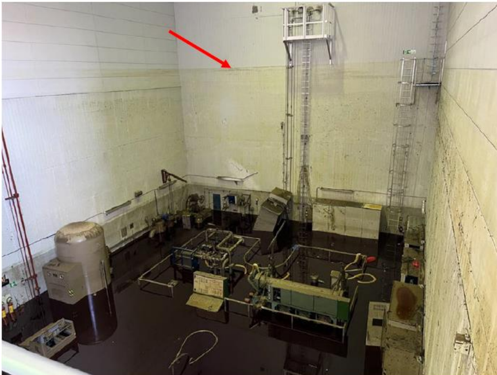
Photo 16: Generator 1 submerged. The photo was taken after most of the water had been pumped out. At the top of the photo you can see the line where the water reached at its peak, marked with a red arrow (Photo DNV)
