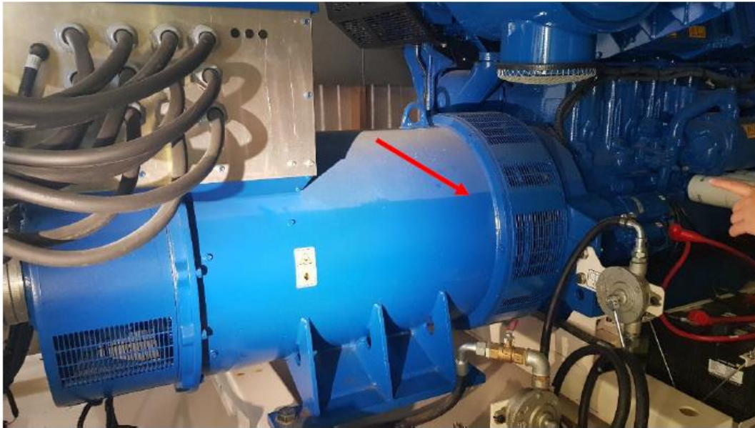
Photo 17: Submerged emergency generator. The line near the top of the generator cover shows where the water reached at its peak, marked with a red arrow (Photo DNV)
