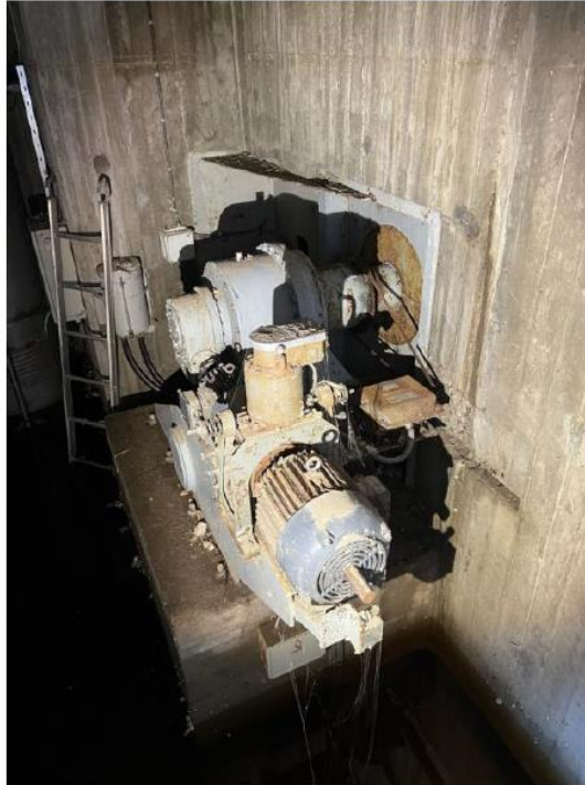
Gate works and motors that have been submerged.
