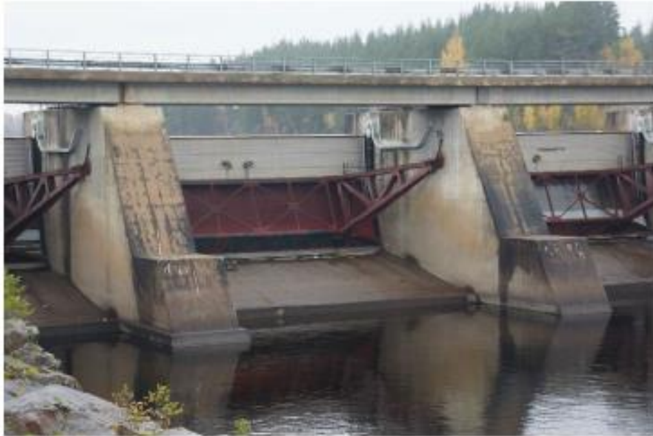
Photo 5: Floodgate 4 in closed position (Photo: Sweco)
