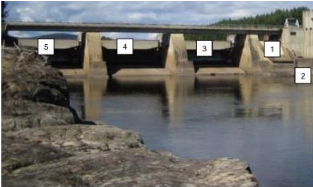
Photo 4: Overview of the gates at Braskereidfoss, as seen from downstream (Photo: Sweco)
