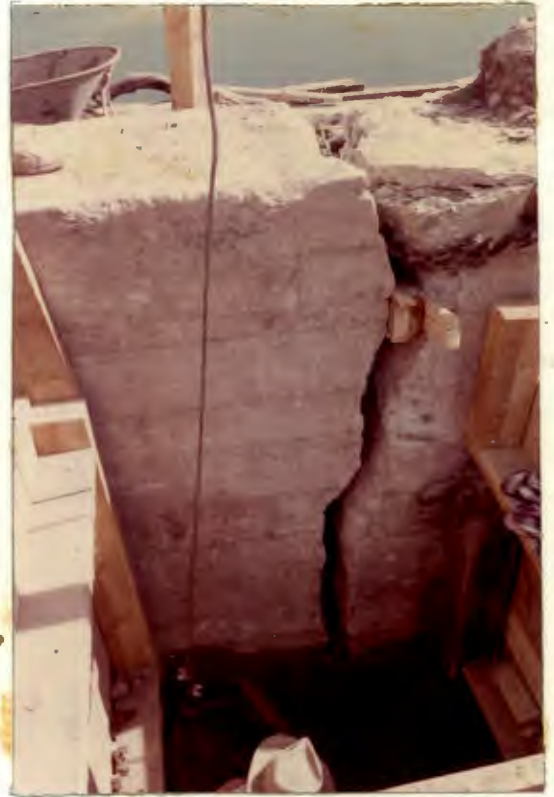
Fig. 9 CRACK IN CORE WALL
