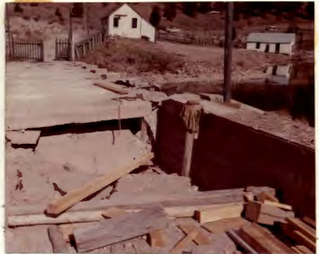
Fig. 8 CREST SETTLEMENT ADJACENT TO SPILLWAY
