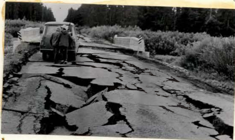
Fig. 13 TYPICAL DAMAGE TO STATE HIGHWAY 287 AT SMALL BRIDGE (M. P. Co. Photo)
