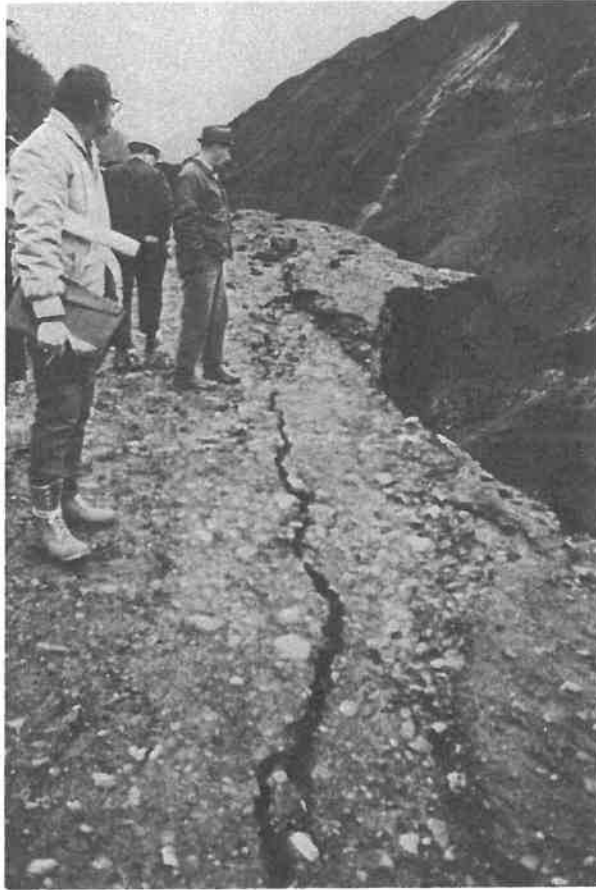
FIGURE 14 Looking Upstream at Edge of Waste Pile.
