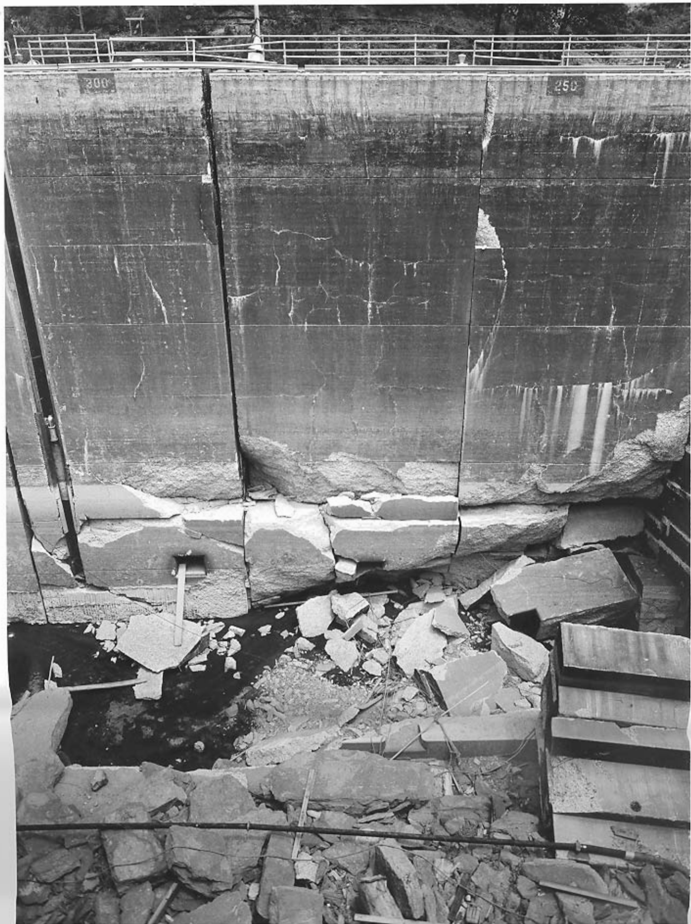
Auxiliary lock, blocks 9, 8, and 7.
