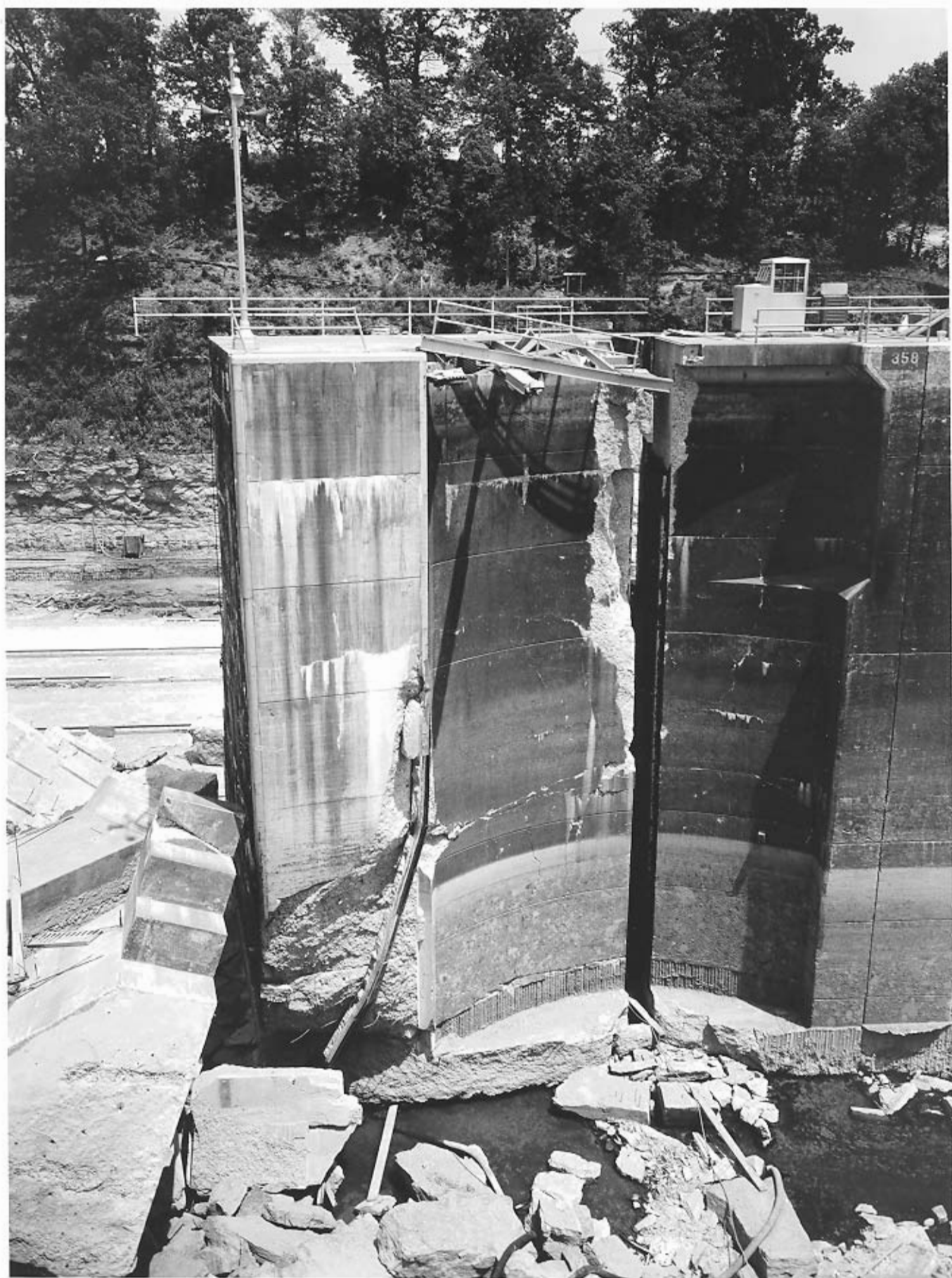
Auxiliary lock, blocks 12 and 11.
