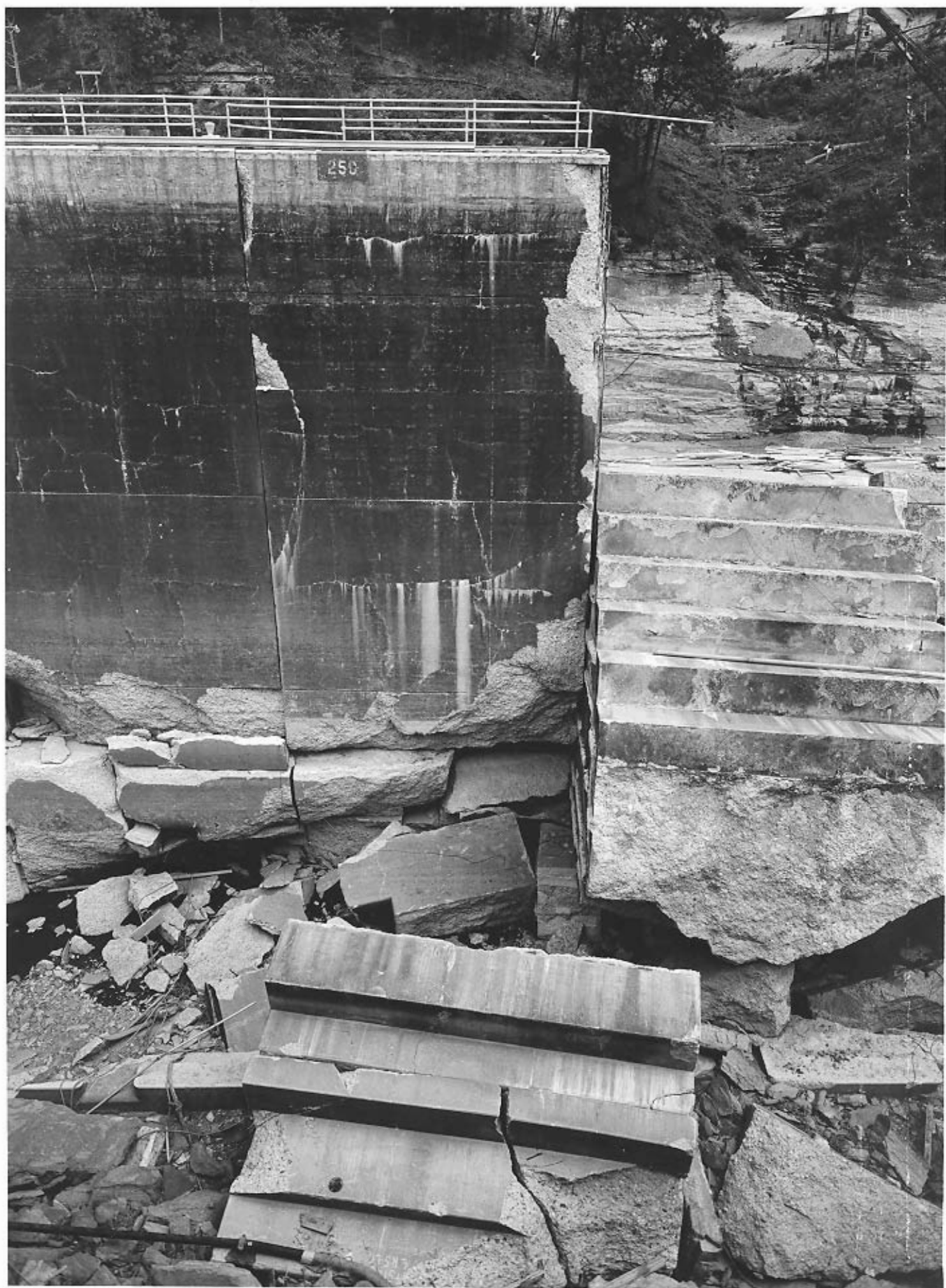
Auxiliary lock, blocks 8, 7, and 6.
