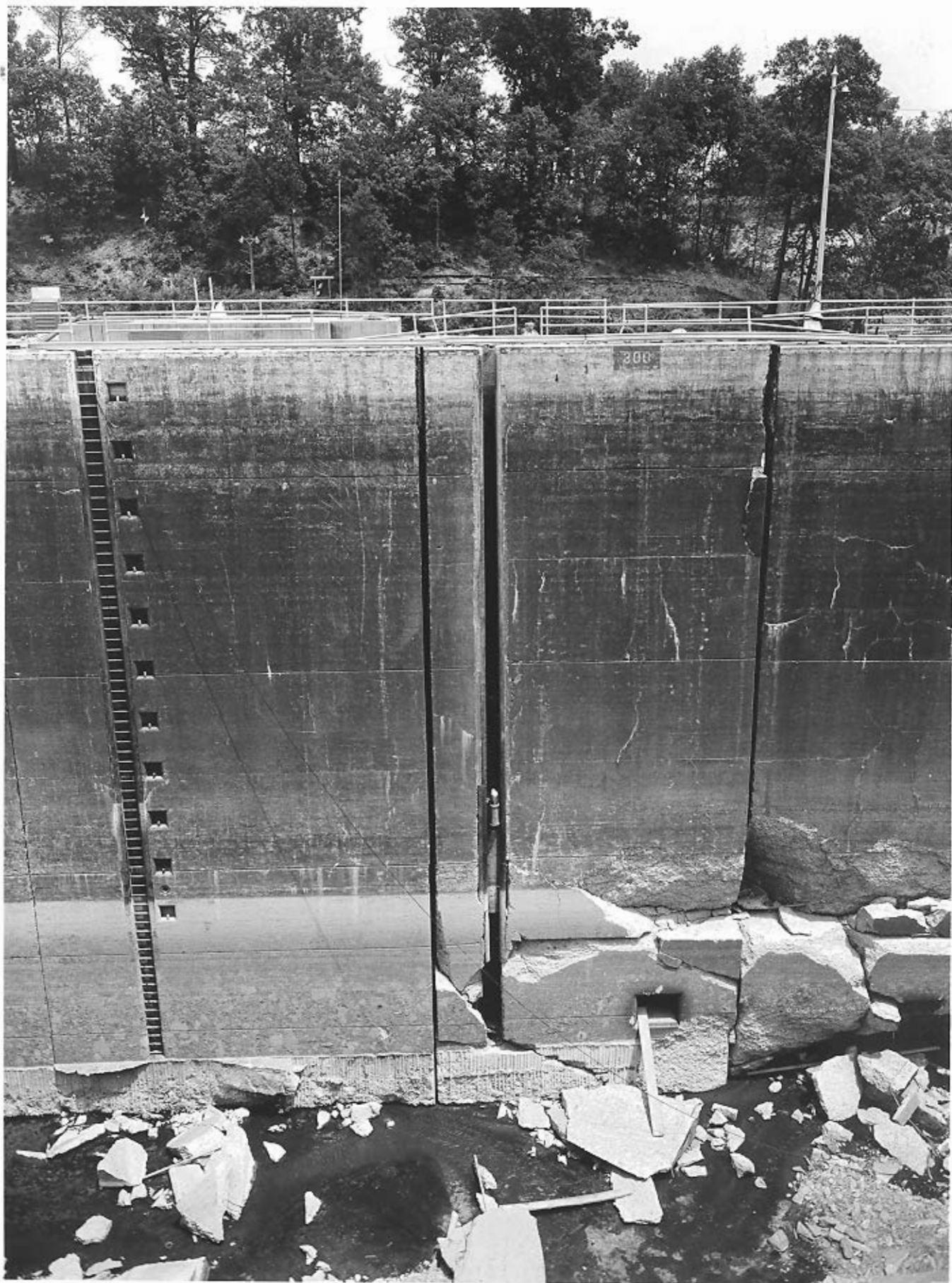
Auxiliary lock, blocks 10, 9, and 8.
