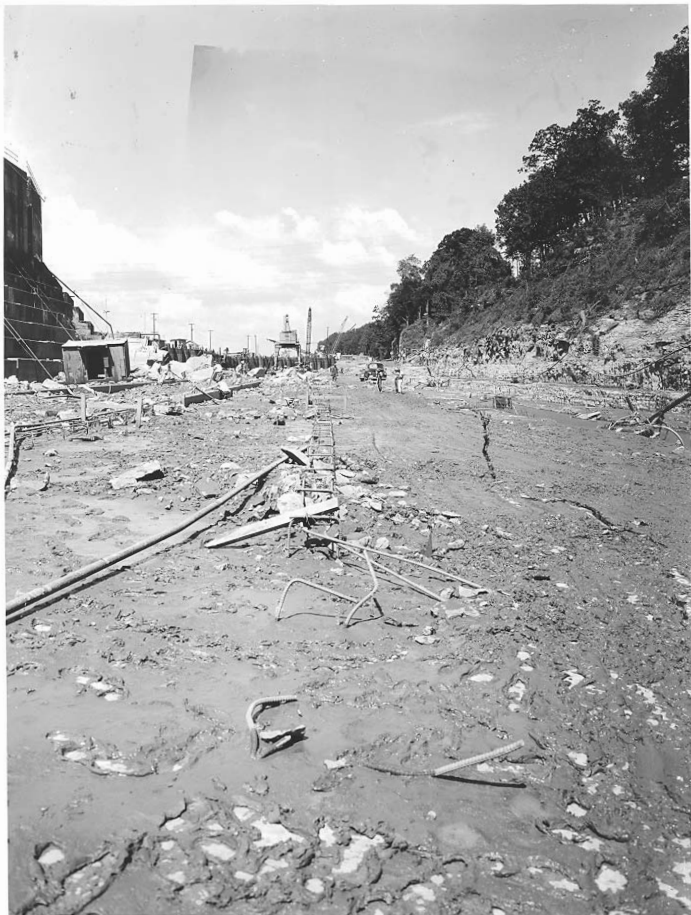
Looking downstream at crack in rock. Note crane runway reinforcing.
