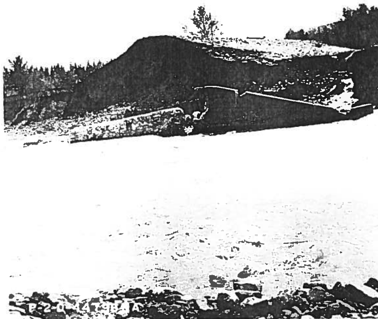
Photograph No. 4 Two Medicine Dam - View of right embankment showing remains of spillway retaining wall. 6-11-64
