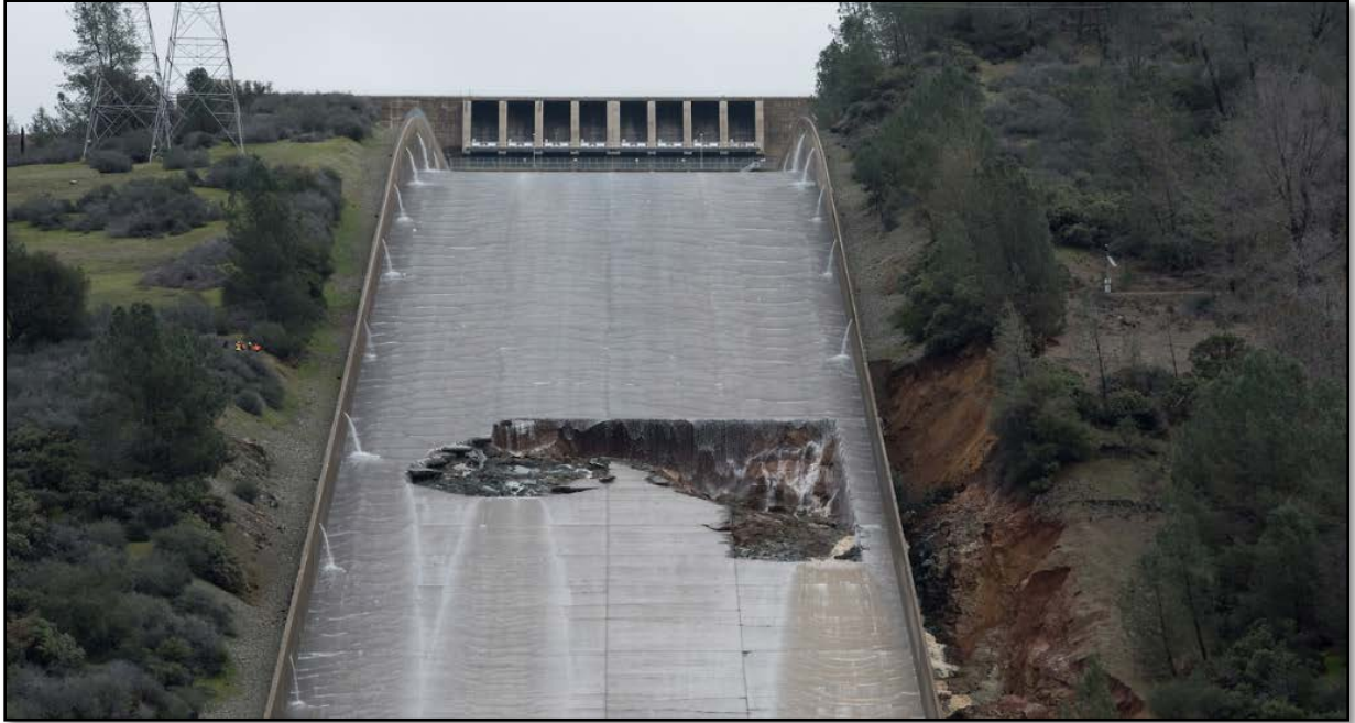
Figure 1-2. A large hole was discovered in the Oroville Dam service spillway chute on February 6, 2017 (Photo courtesy of California DWR).
