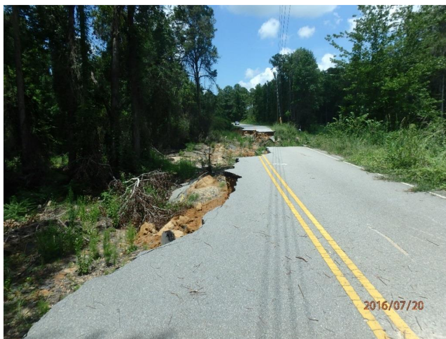
Figure 12: Head-Cutting of the Embankment at SCNONAME 14008 (Source: FEMA 2016)
