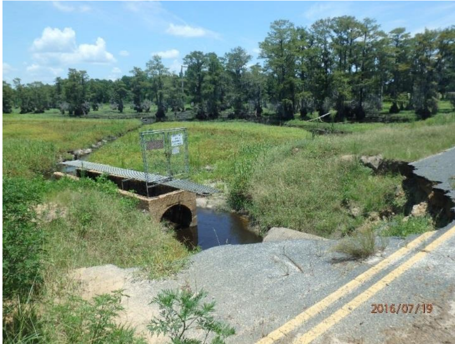
Figure 14: Piping Failure at SCNONAME 14005 (Source: FEMA 2016)
