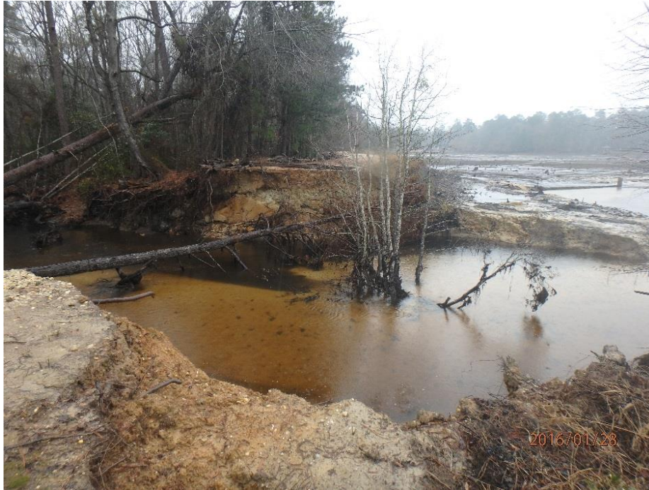
Figure 16: Structural Failure at Duffies Pond Dam (Source: FEMA 2016)
