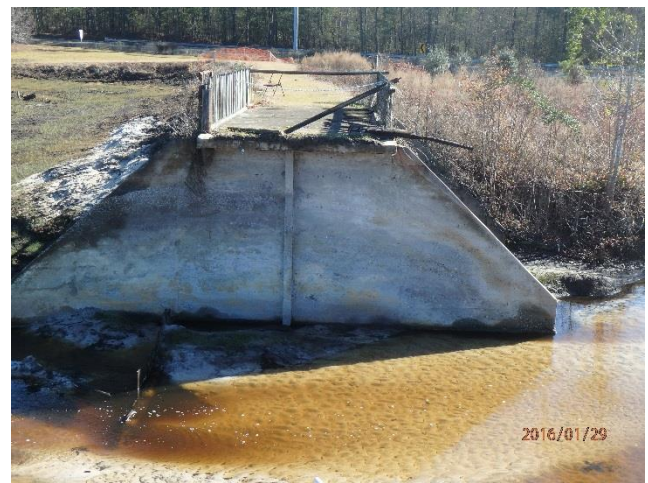
Figure 15. Example of Structural Failure at JW Smoaks Pond (Source: FEMA 2016)
