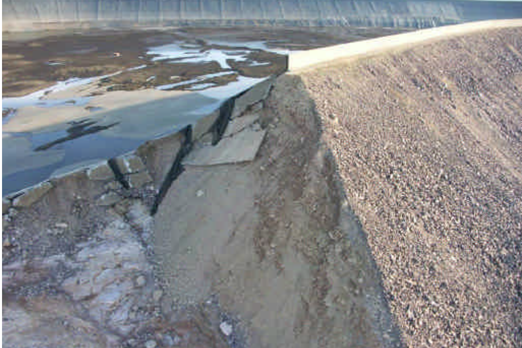
FIGURE 4-2 CLOSE UP VIEW OF WEST SIDE OF BREACH AREA
