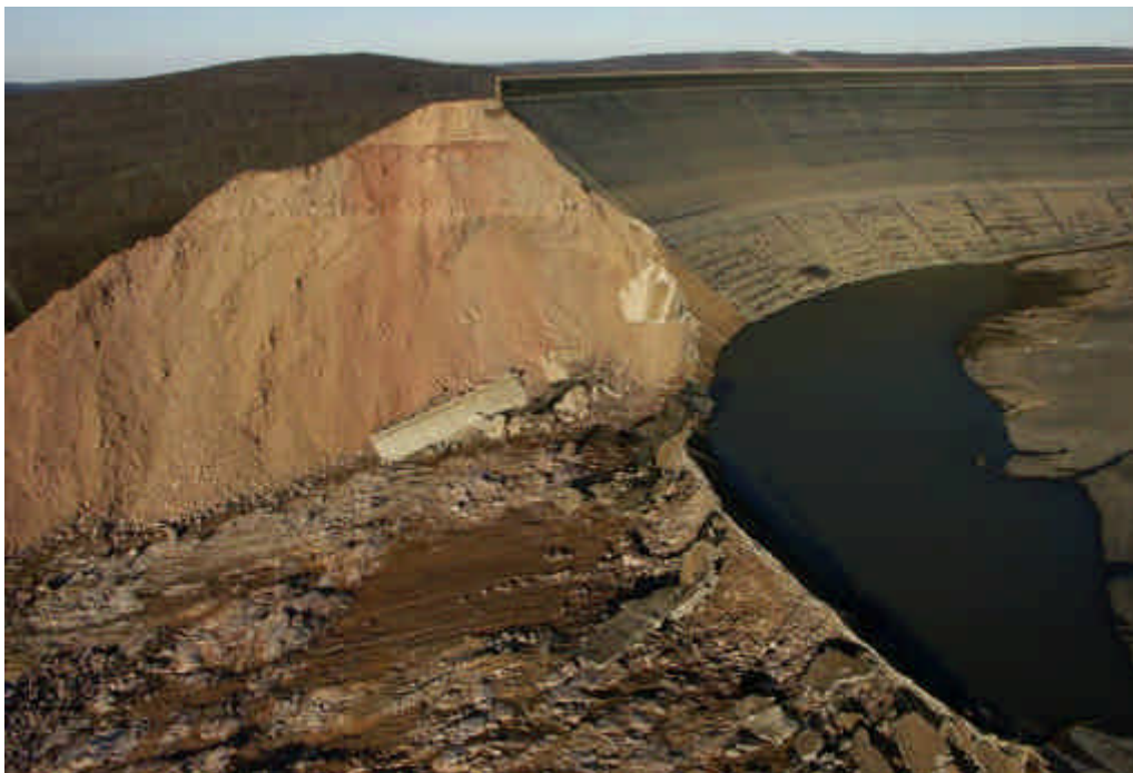
FIGURE 4-3 CLOSE UP VIEW OF EAST SIDE OF BREACH AREA
