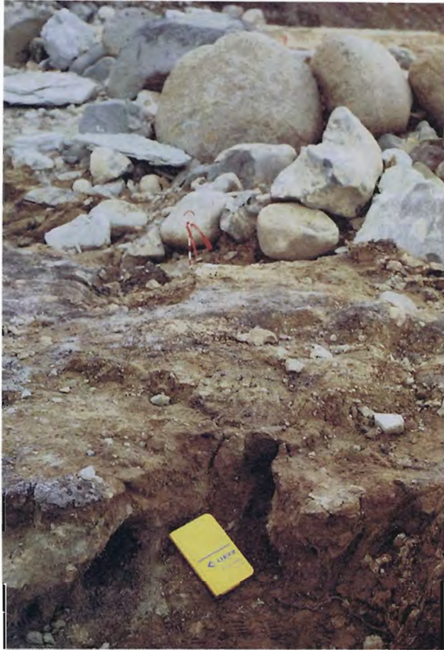
37. View of erosion channels upstream near station 5 + 50.
