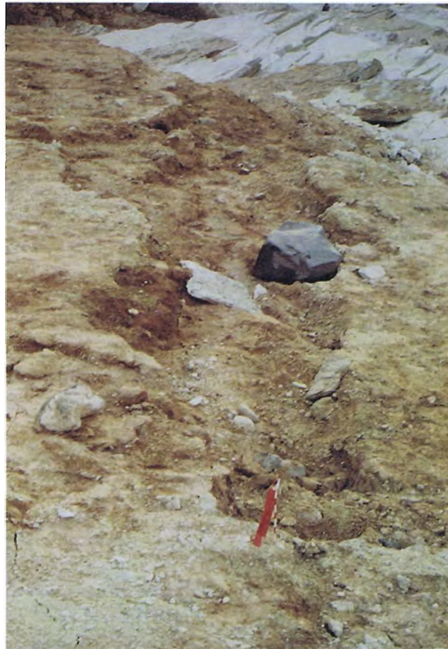
40. View of depression in remaining fill, upstream shell area.
