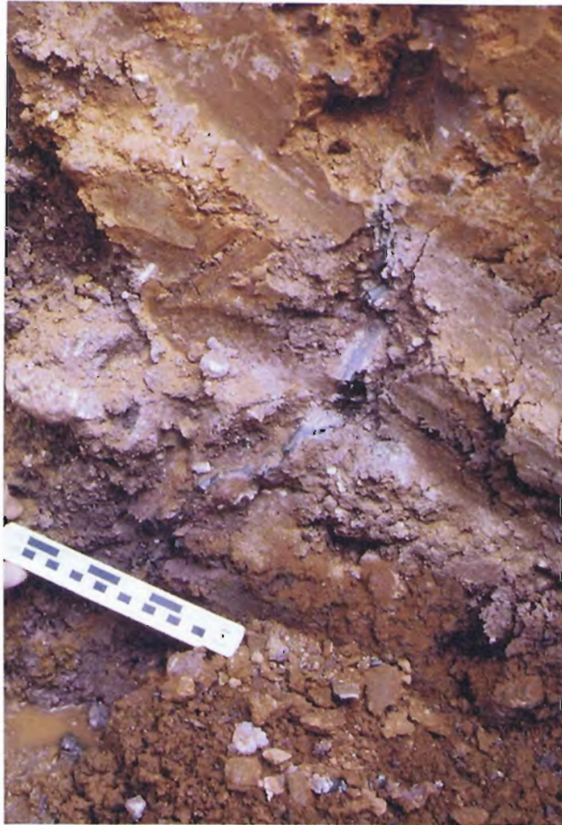
55. Grout intrusion through Zone II in cutoff trench on left side of breach.
