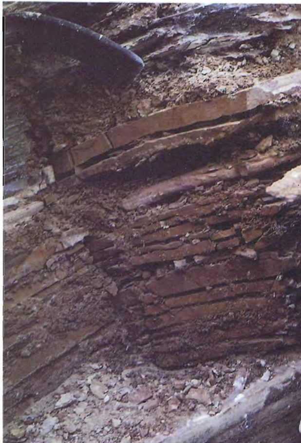
6. Weathered gypsiferous siltstone with open bedding planes; south wall of key trench, station 3 + 16, 10 feet below surface. (12-16-83)
