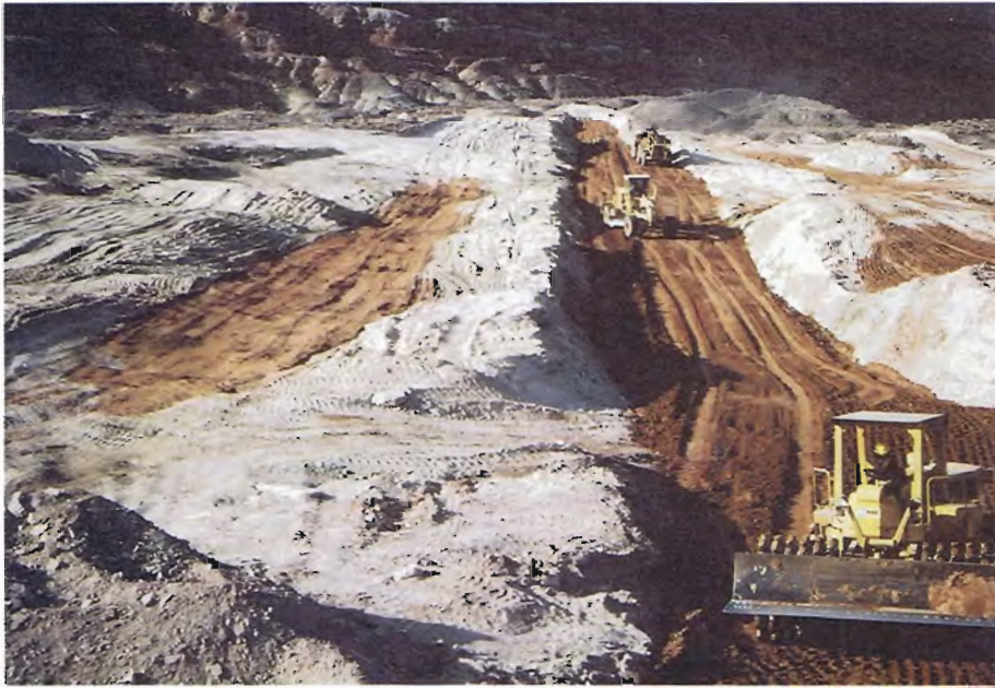
7. View west showing Zone I being placed in key trench and in hollows beside trench. (1-12-84)
