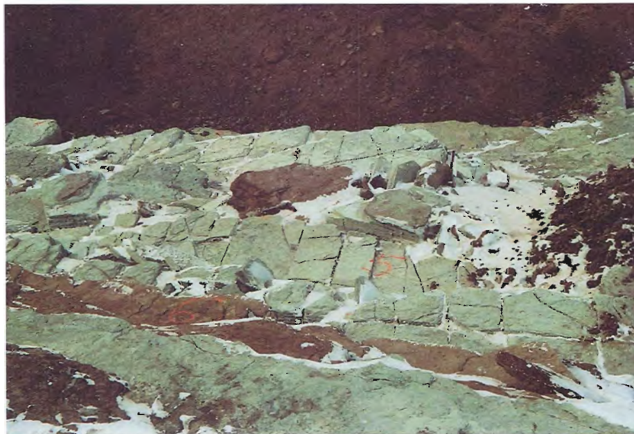
20. Joint pattern in breach area.
