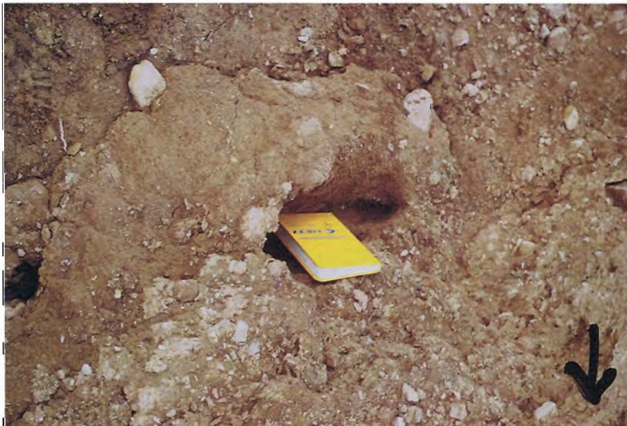
38. View of erosion channels upstream near station 5 + 50.
