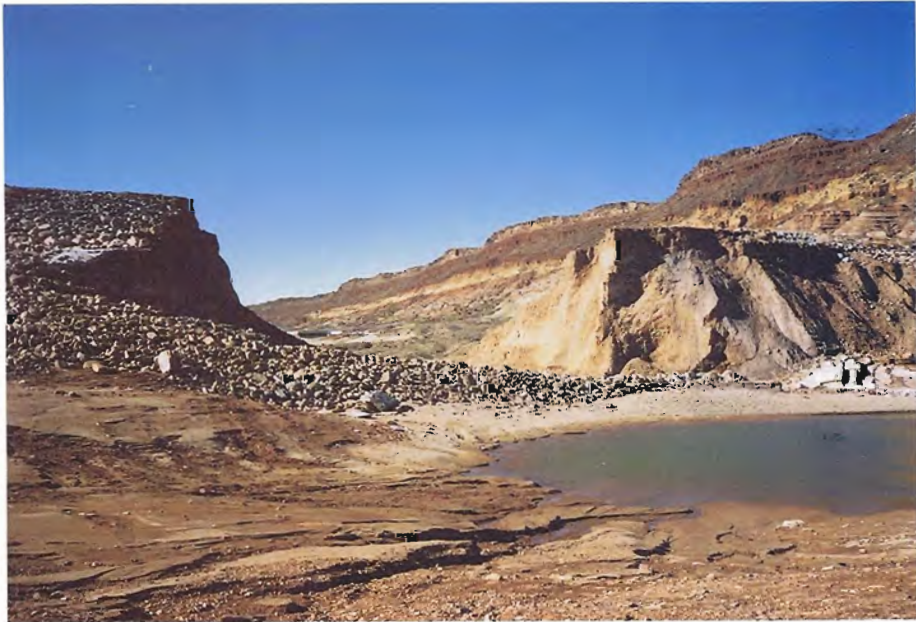
14. Breach from upstream.
