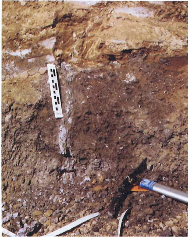
51. Grout extending through Zone I and Zone II on right side of breach at centerline of cutoff trench.
