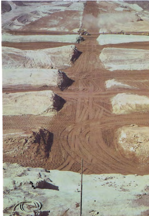
8. View west past grouting operation on left abutment showing placing of fill. (2-8-84)
