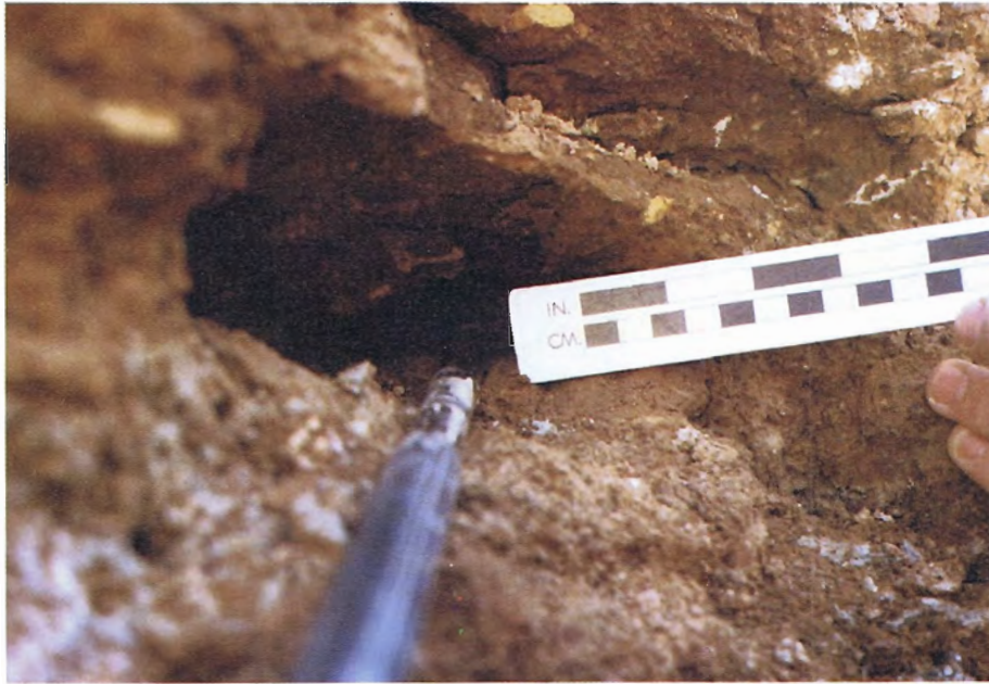
45. Piping channel found in exploratory trench upstream of dike centerline on left side of breach.
