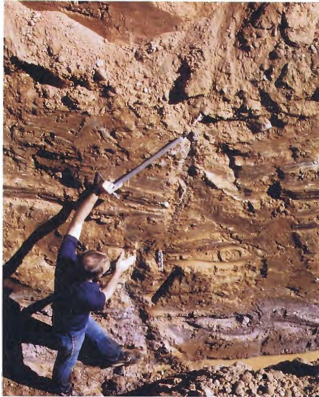
49. Grout filling crack noted in exploratory trench on centerline of cutoff on left side of breach.
