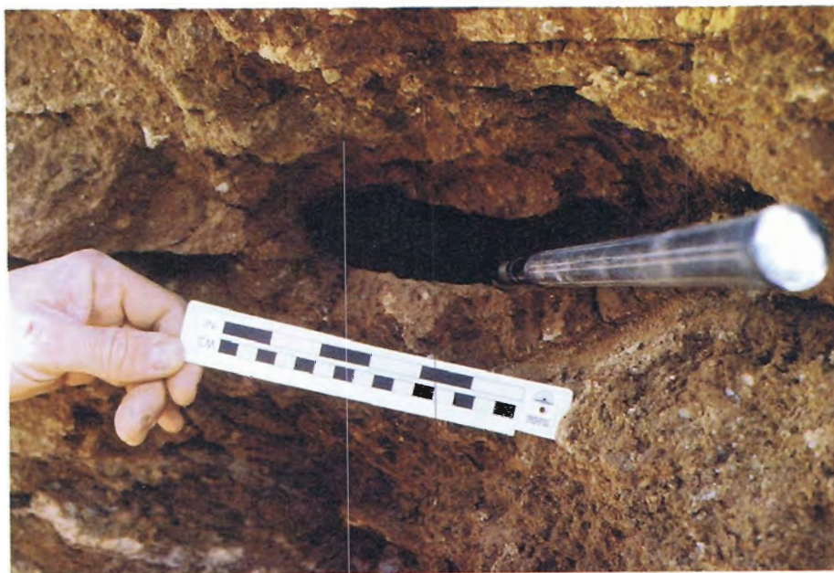
46. Piping channel found in exploratory trench upstream of dike centerline on left side of breach.
