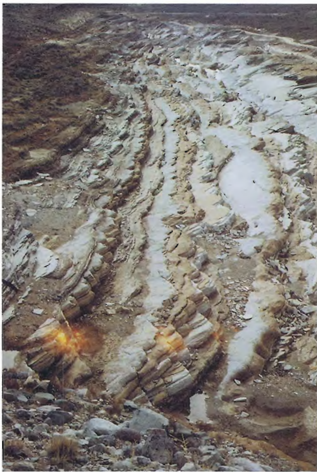
15. Erosion downstream of dam showing dip of beds into left abutment.
