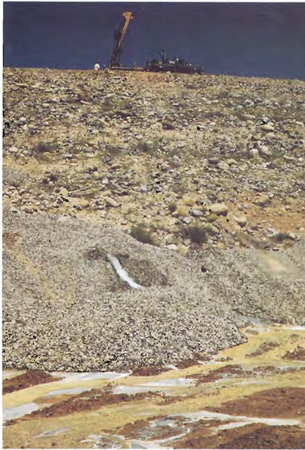
11. Sewer rock dumped on spring at toe of dike, somewhere between 7 + 00 and 8 + 00. (8-3-87)
