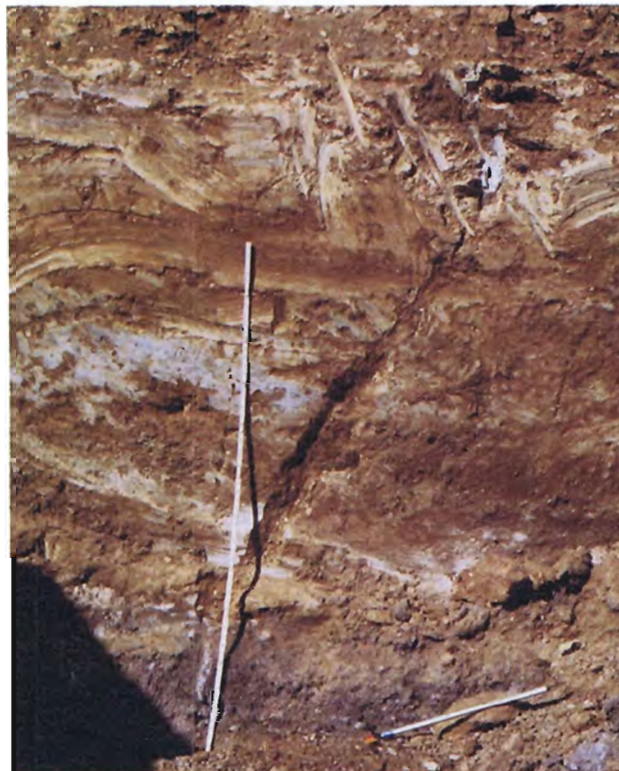
52. Grout intrusion through entire depth of cutoff trench on right side of breach.
