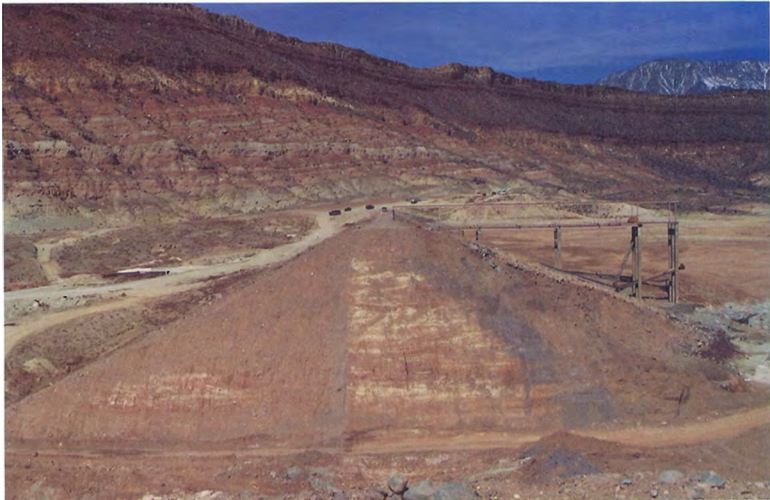
43. View of right embankment showing zoning remaining following sloping of breach side.
