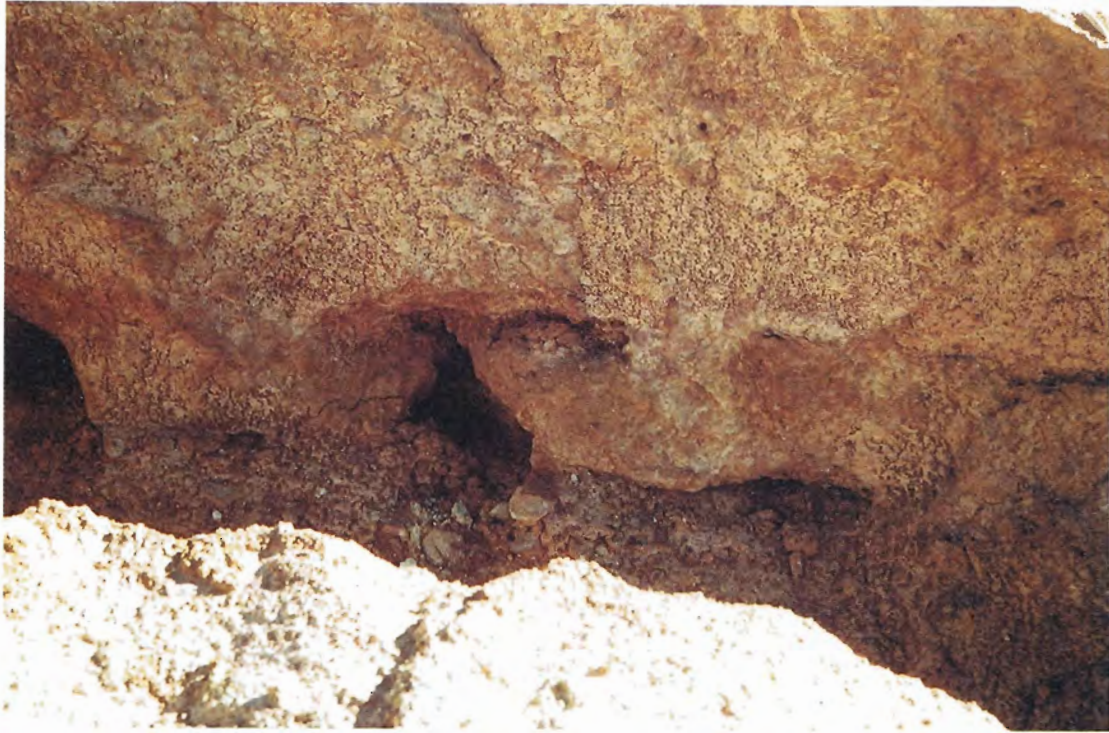
39. View of erosion channels upstream near station 5+50.
