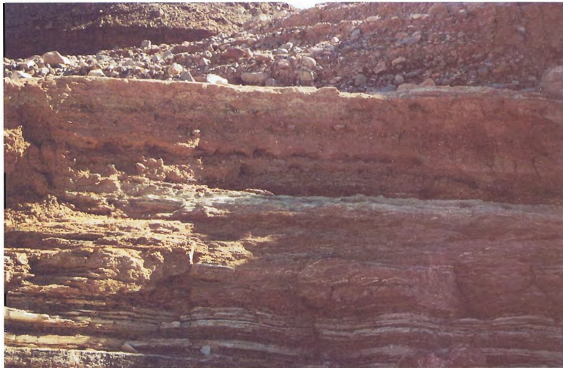
34. View of erosion channel near contact of dam and foundation downstream near station 4 + 50.
