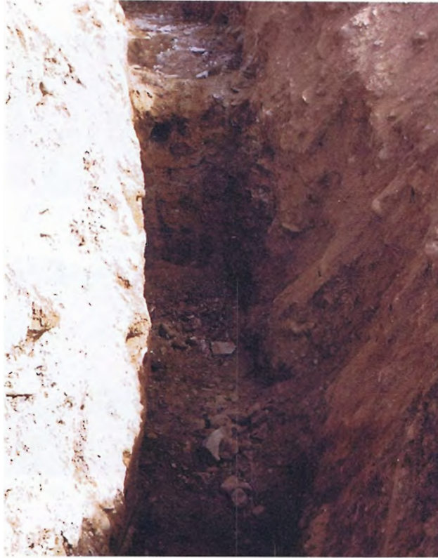
47. Drain pipe encountered in exploratory trench at original downstream toe of dam.
