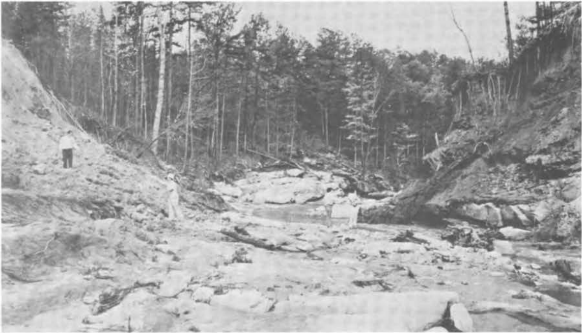
FIGURE 4a Dam looking downstream through breach
