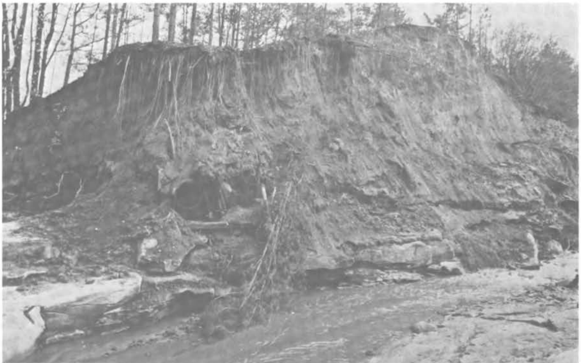
FIGURE 6 Face of breach on right side looking southwest, showing old penstock and remains of 1899 crib dam at downstream toe on left
