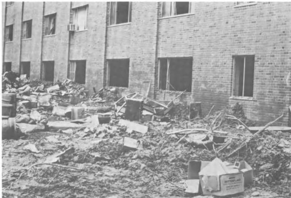
FIGURE 9b Dormitory looking at riverside face. High water line about top of windows, debris and mud shoveled from rooms looking for bodies
