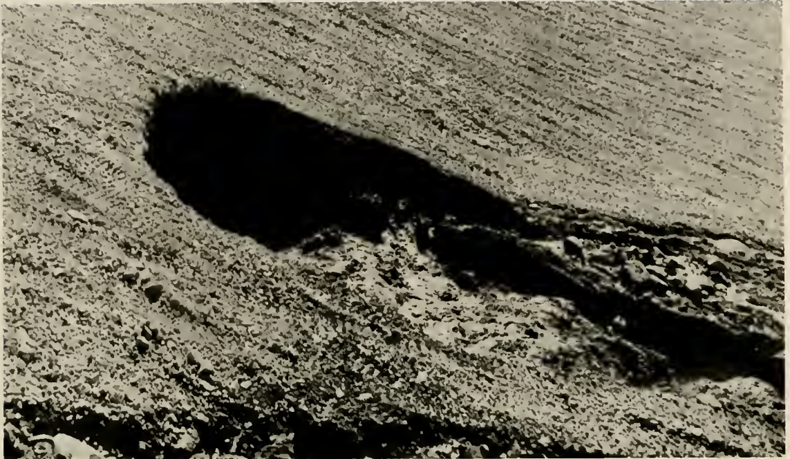
Figure 21.—Closeup of leak at El. 5200 near right abutment. About 10:30 a.m., June 5, 1976.
