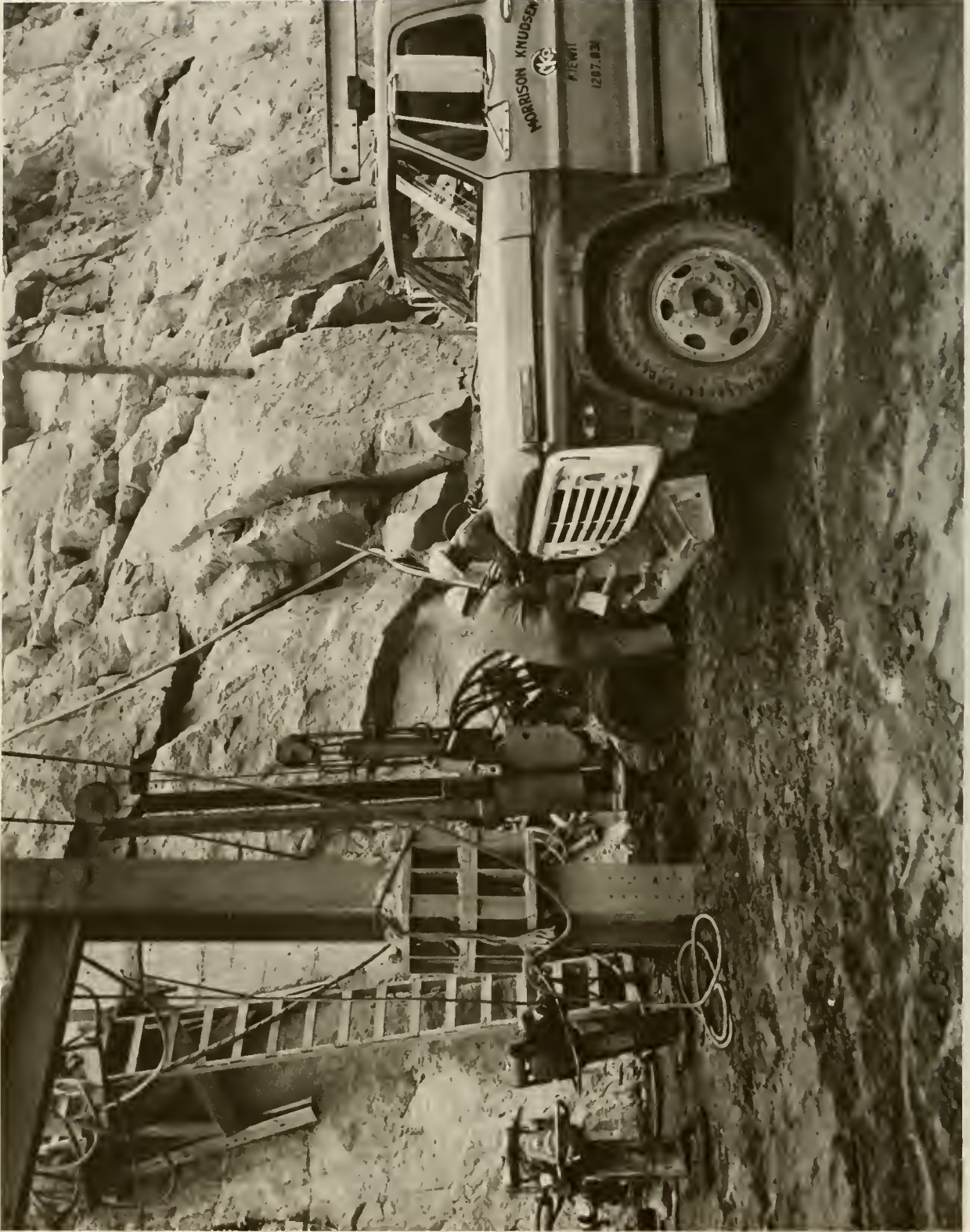
12.—Hydraulic hammer used for special compactor along abutment and around tower supports, 7/2/74; P549-147-4590 NA.
