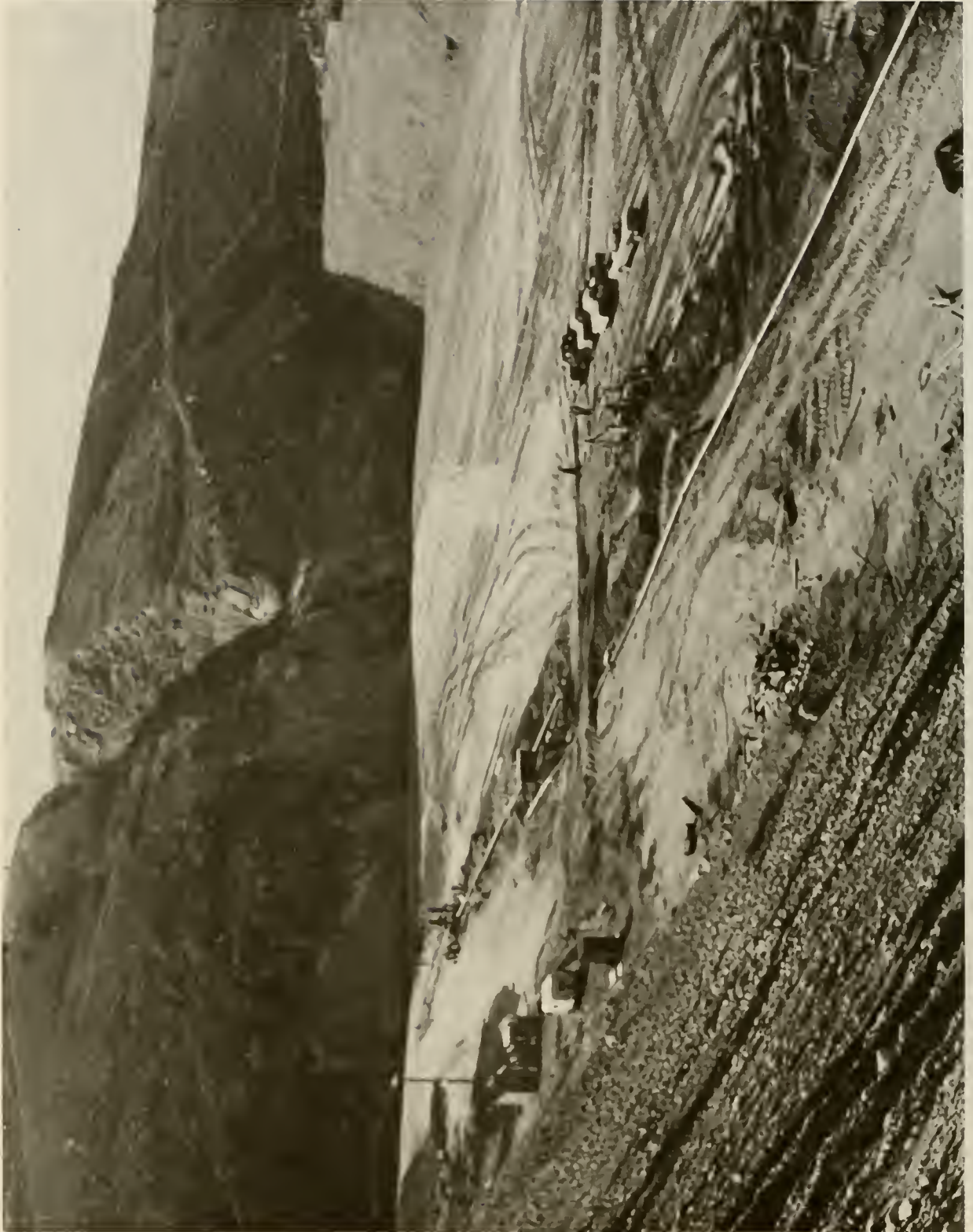
8.—Dewatering operations zone 1 cutoff trench to take care of seepage due to high water on the upstream side of the dam, 6/18/74; P549-147-4539 NA.
