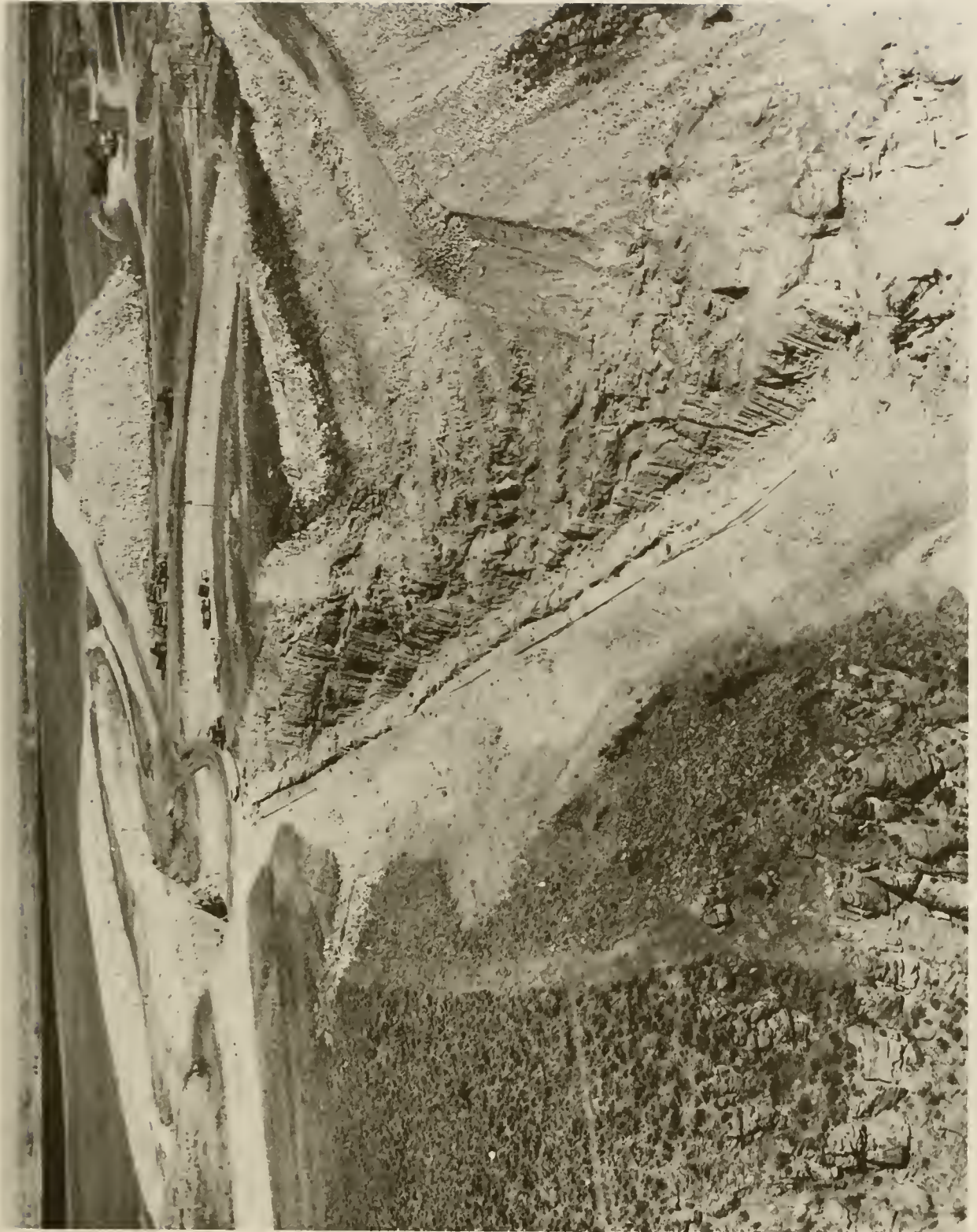
1.-View of right foundation keyway trench and zone 5 stockpile, also portion of spillway area, 7/19/73; P549-147-2912 NA. Note number of benches with adjacent steep faces.
