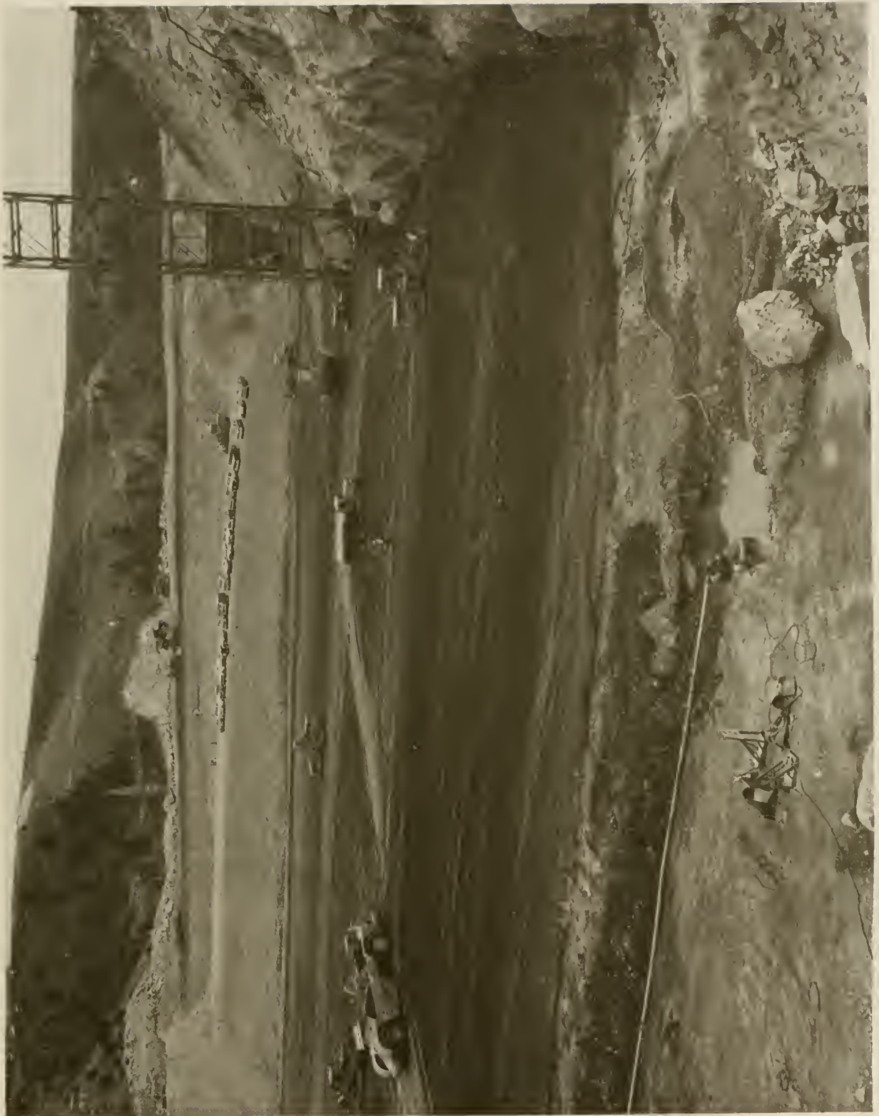
11.--Viewing zone 1 fill and preparation work. Taken from station 16+00, 550 feet upstream, 7/2/74; P549-147-4589 NA.
