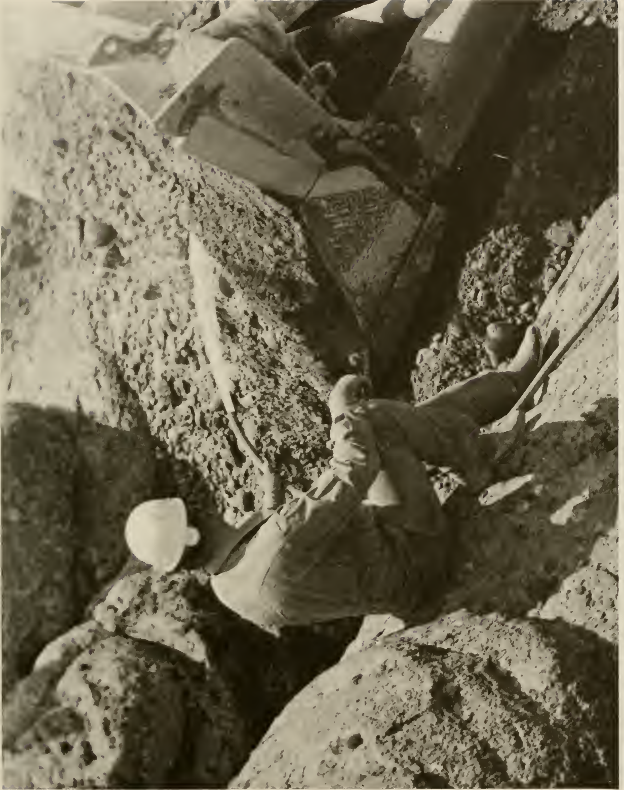
9.—View of sluicing operation on zone 2 blanket area. Material is sluced into cracks between rocks to insure all voids are filled. 7/19/72; CN549-147-140 NA.
