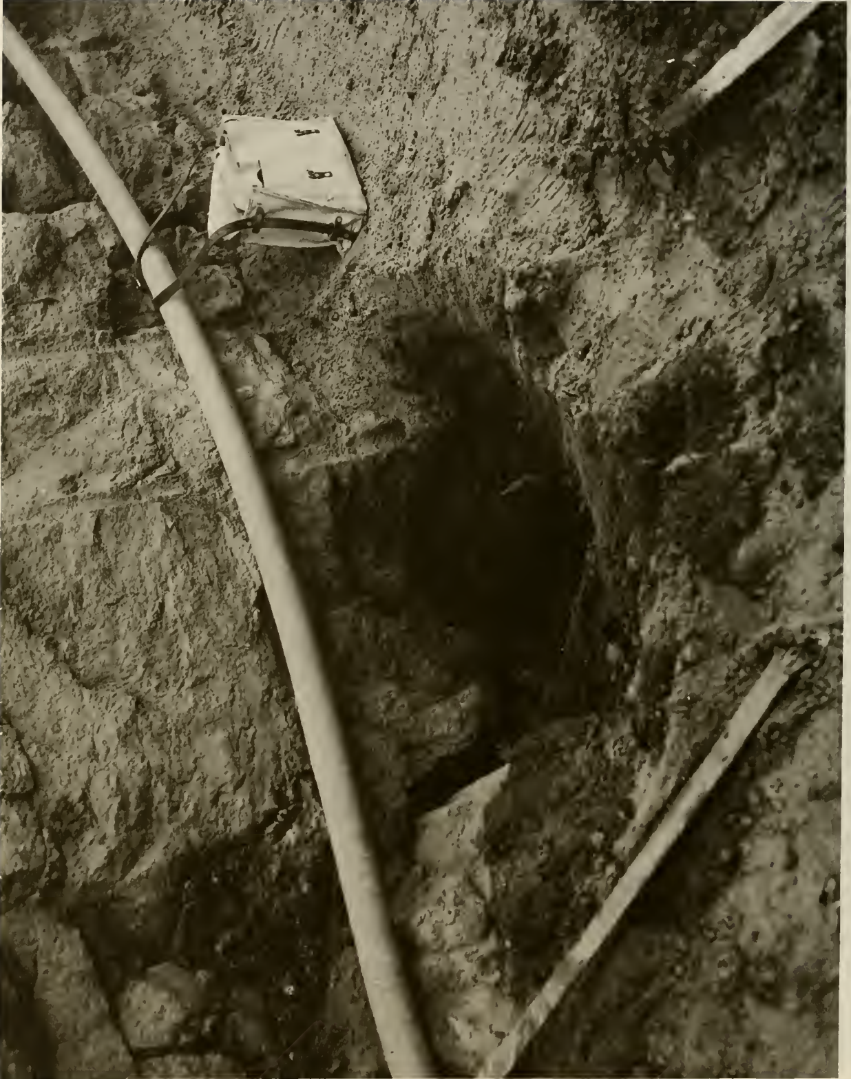
14.—View of open joint on the right abutment at elevation 5142, station 14+52, 90 feet upstream ready to be grouted, 11/14/74; P549-147-5216 NA.
