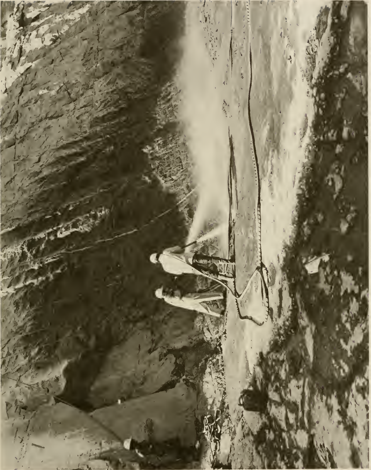
3.—View of workmen cleaning rhyolite in bottom of cutoff trench. Photo taken at station 18+10, 90 feet upstream from centerline of dam, 10/15/73; P549-147-3356 NA.
