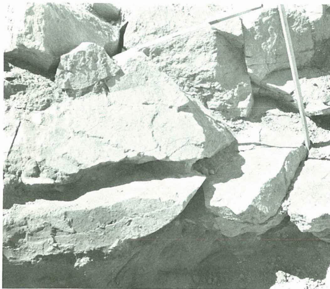
Fig. E-8 Intensively jointed ash-flow tuff in downstream face of right abutment key trench at El. 5290. (post-failure)
