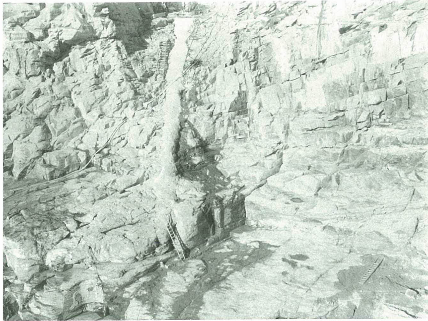
Fig. E-23 Joint system near missing segment of grout cap Sta. 14+00 behind ladder in lower center. (post-failure)
