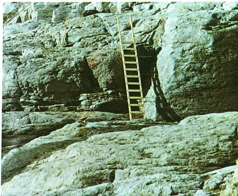
Fig. 3-10 Grout cap severed at Sta. 13+96 and missing to Sta. 14+26. Open fracture shown in Fig. 3-12 is behind the ladder
