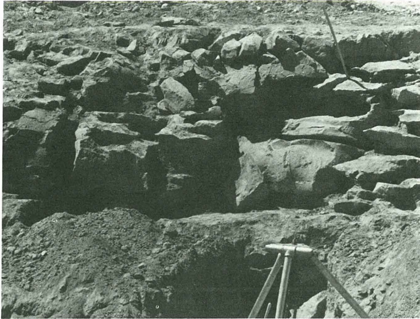
Fig. E-11 Downstream of wall of right abutment key trench. Elevation in center of photo is about 5290. (post-failure)
