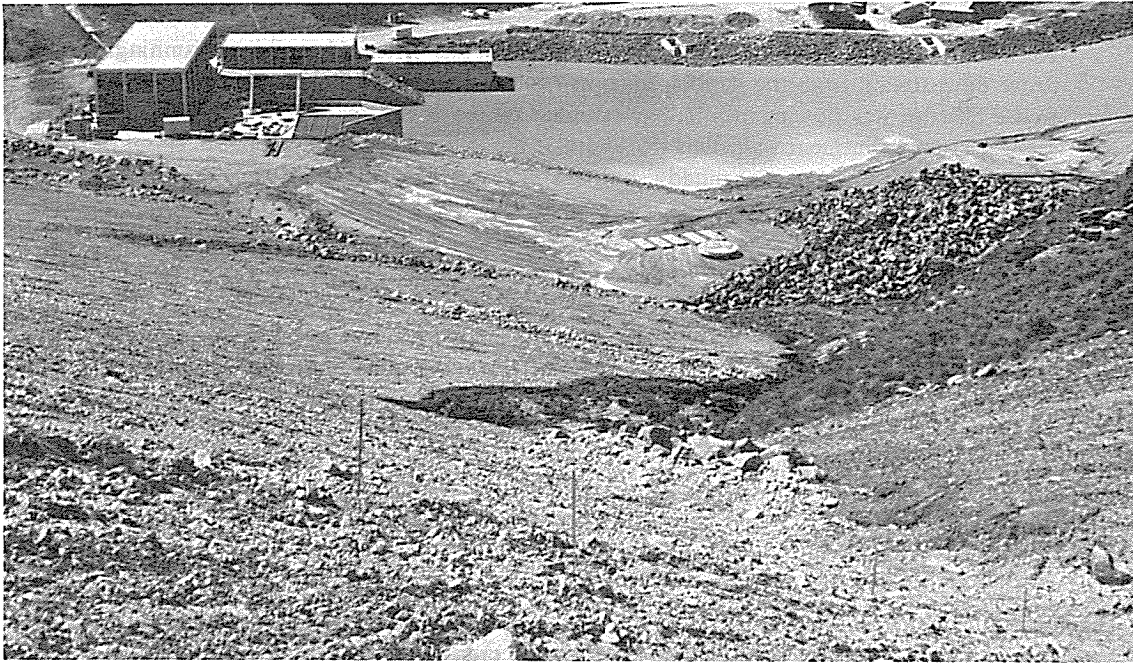
Fig. 2-7. View from top of embankment toward leak at El. 5200 near right abutment. Approximately 10:30 a.m. June 5, 1976.
