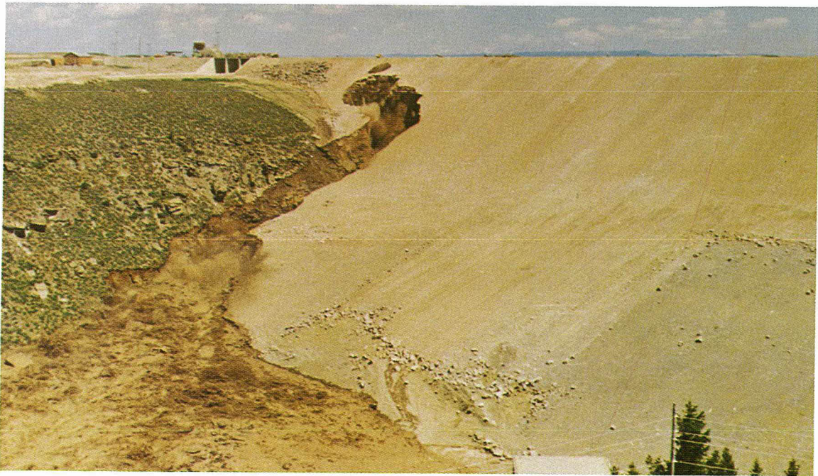
Fig. 2-12. Second hole in face of dam. A few minutes after 11:30 a.m. June 5, 1976.
