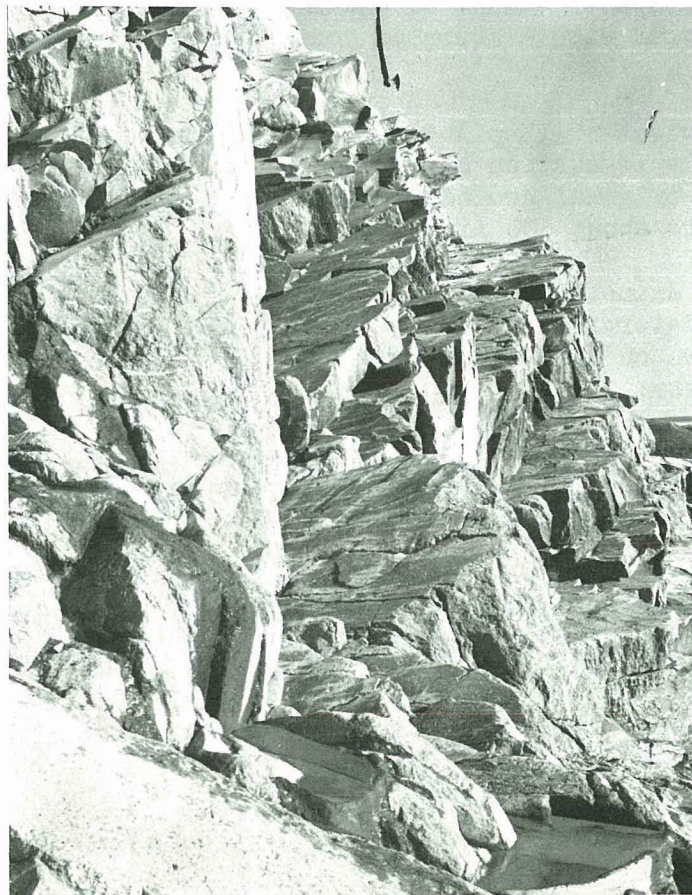
Fig. E-24 View across grout cap toward prominent joint near Sta. 13+30. (post-failure)
