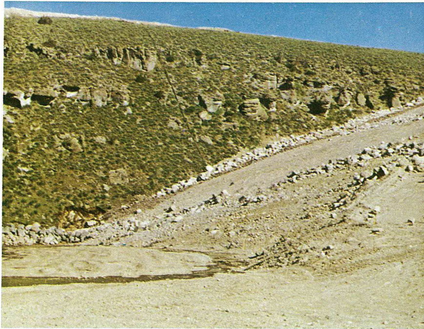
Fig. 2-5. Muddy flow at about El. 5045 at right downstream toe estimated 20 to 30 cfs (9,000 to 13,500 gpm) 8:30 a.m. June 5, 1976.
