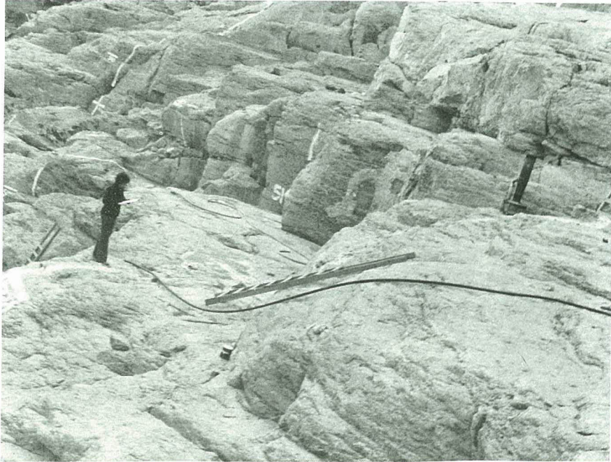
Fig. E-21 Prominent rock joints in vicinity of missing grout cap segment — bottom of photo. (post-failure)
