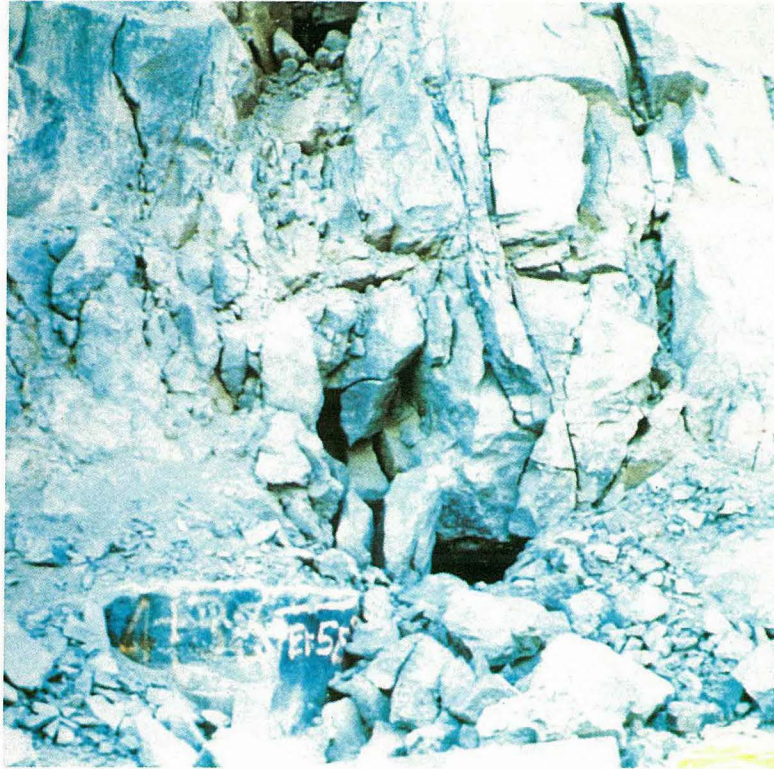
Fig. 5-17 Rock fissure near Sta. 4+34 discovered during excavation of key axis trench of the dam. Crevice extends through axis of dam for nearly 100 ft both upstream and downstream. (1974)
