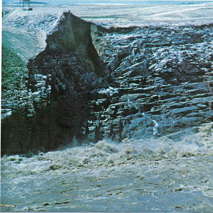
Fig. 5-8 Showing prevalent horizontal joints upstream and dominating vertical joint system downstream of dam in right wall of canyon (post-failure photo)
