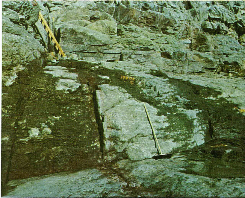
Fig. 3-11 Three vertical joints crossing alignment where grout cap is missing between Stas. 13+96 and 14+26
