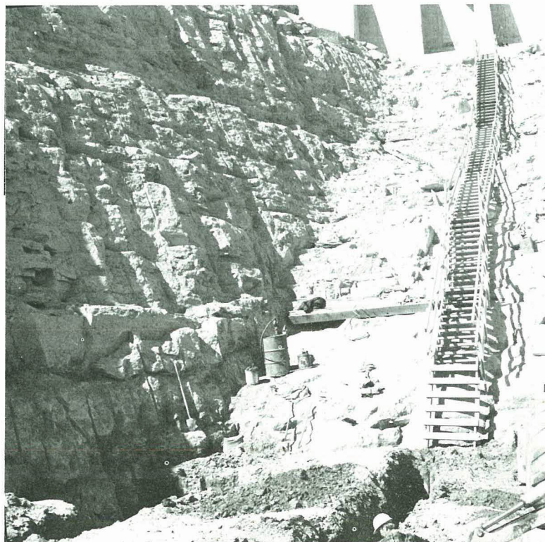
Fig. E-16 Downstream wall of right abutment key trench. (post-failure)
