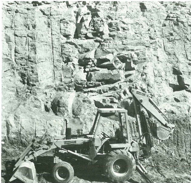
Fig. E-14 Upstream face of right abutment key trench at Sta. 12+70. Fill at El. 5240. (post-failure)
