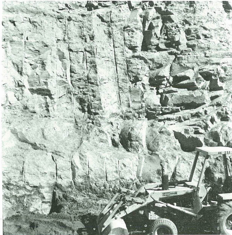
Fig. E-15 Upstream wall right abutment key trench at Sta. 12+65. Elevation of fill is 5240. (post-failure)
