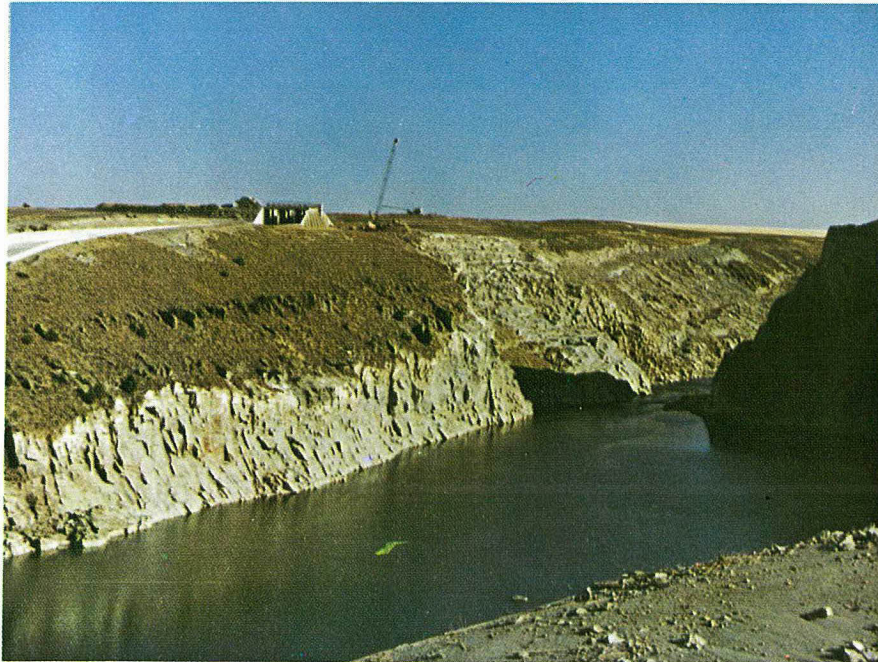
Fig. 5-12 Prominent vertical joints in right wall of canyon downstream of the axis of the dam. (post-failure photo)
