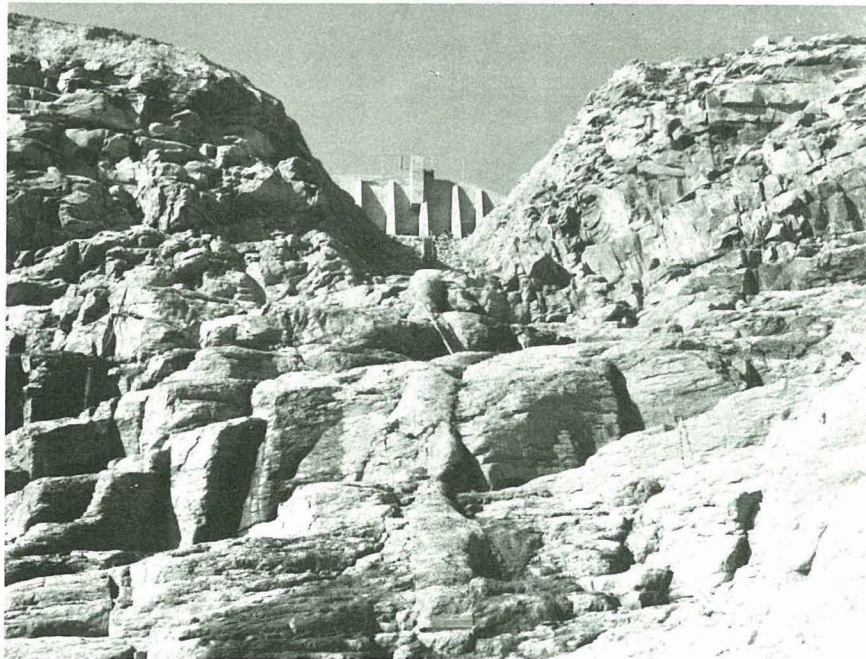
Fig. E-12 View along grout cap; key trench, and spillway in background. (post-failure)
