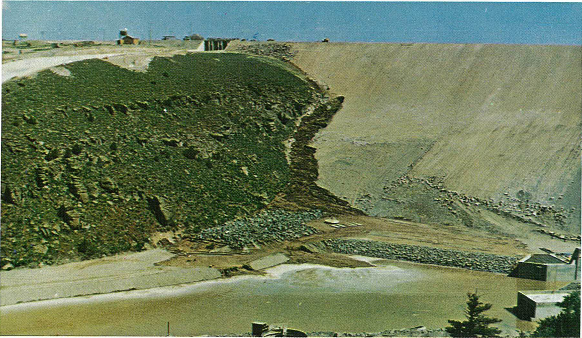
Fig. 2-9. Flow increasing. Dozers sent to fill hole at El. 5200. About 10:45 a.m. June 5, 1976.
