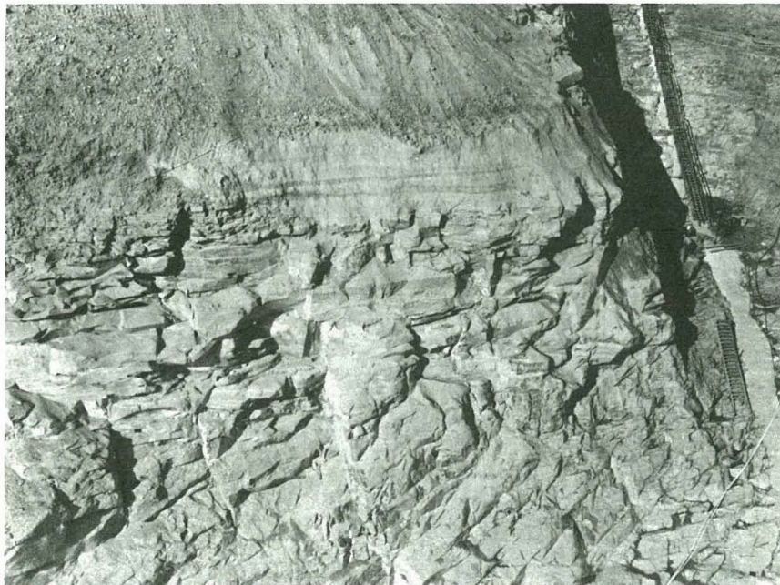
Fig. E-18 Right abutment of dam immediately downstream from grout cap. (post-failure)
