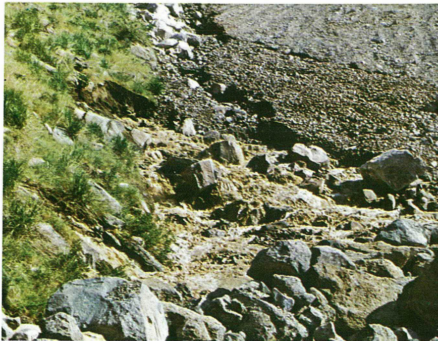
Fig. 2-6. Close-up of leak shown in Fig. 2-5. Muddy flow through rock on right abutment at about El. 5045. 8:30 a.m. June 5, 1976.
