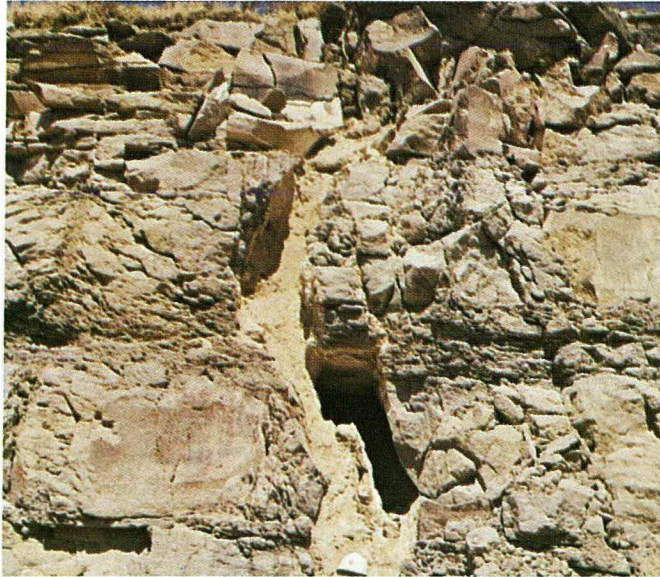
Fig. 5-19 Opening in upper right wall of Teton Canyon 1/8 to 1/4 mile upstream from dam. (post-failure photo)
