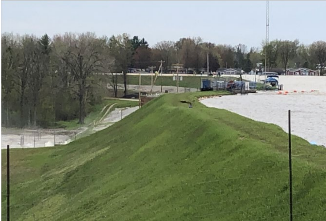
Figure 7: Photograph showing the downstream side of the Edenville left embankment at 5:31 p.m., Tuesday, May 19, 2020
