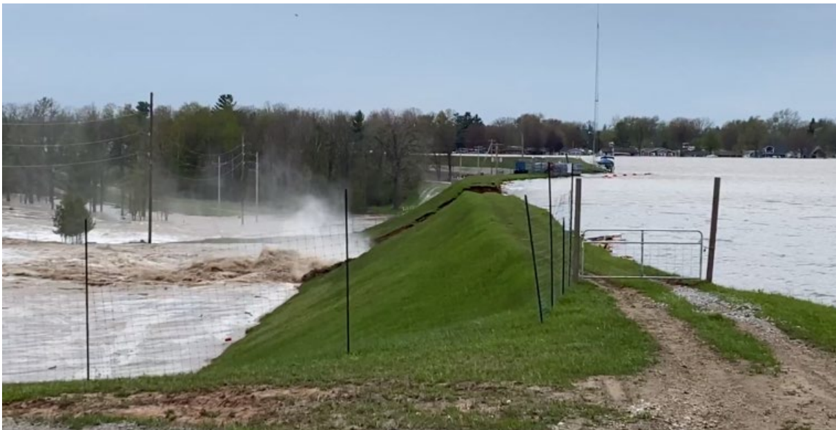
Figure 17: Enlarged still image from dam failure video at 36 seconds
