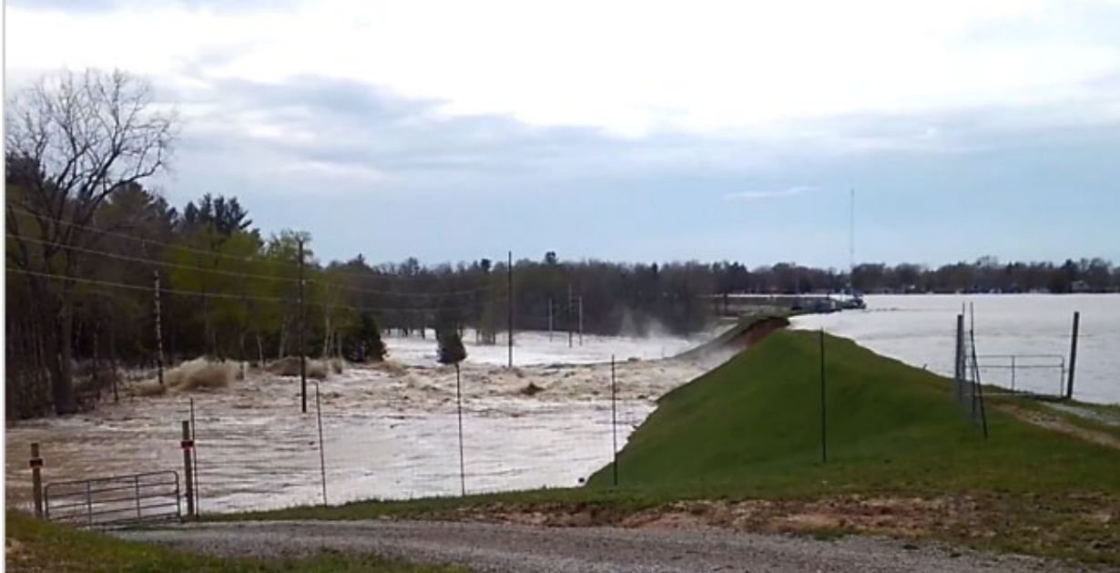
Figure 18: Edenville left embankment breach at 6:00 p.m. on Tuesday, May 19, 2020
