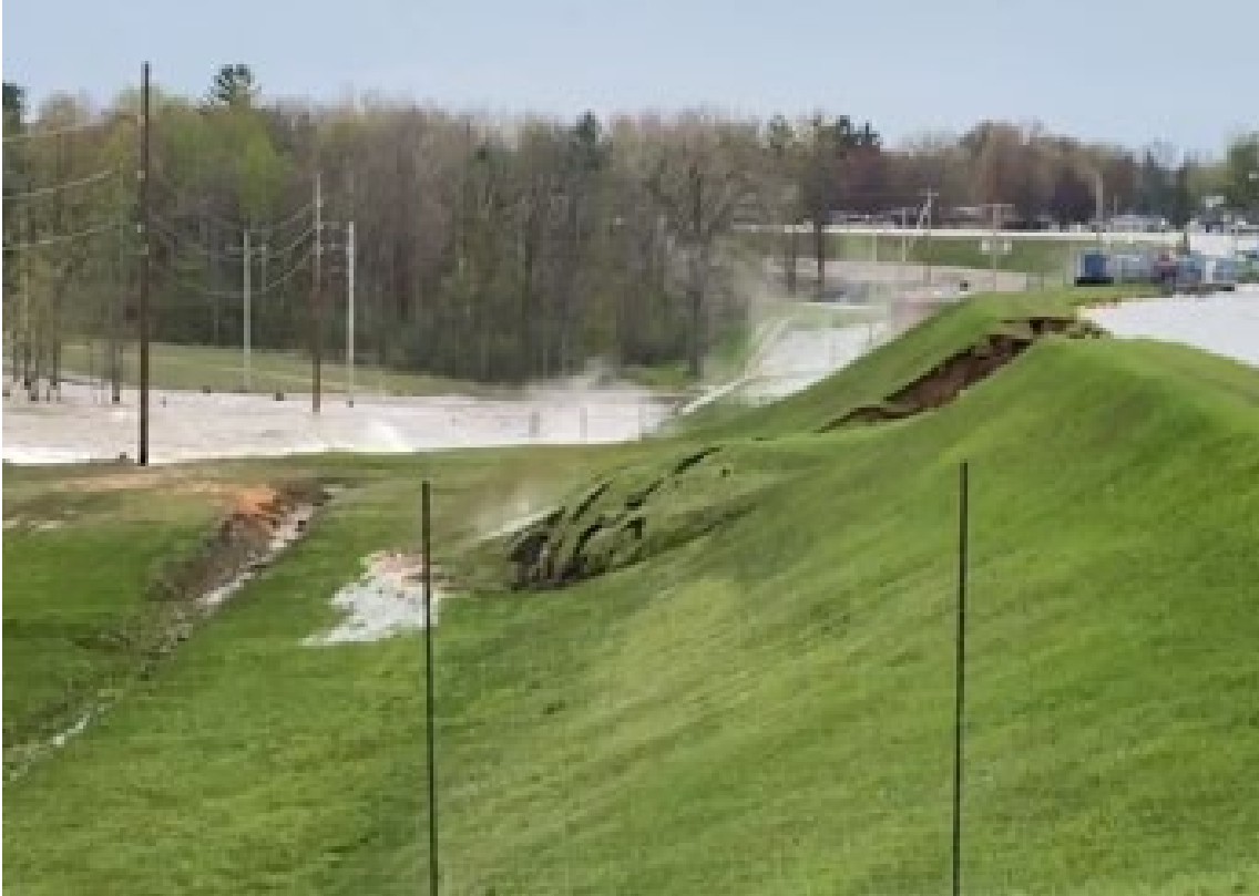
Figure 12: Enlarged still image from dam failure video at 7 seconds
