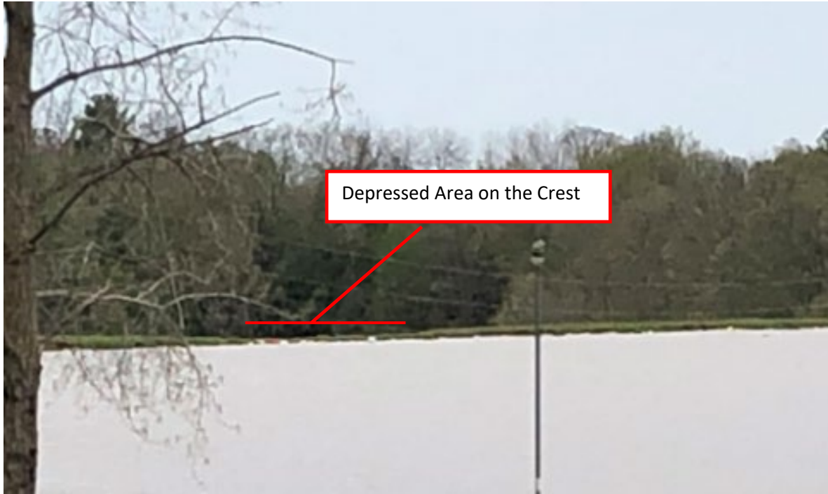
Figure 5: Photograph showing depression in the crest of the Edenville left embankment at 5:20 p.m., Tuesday, May 19, 2020
