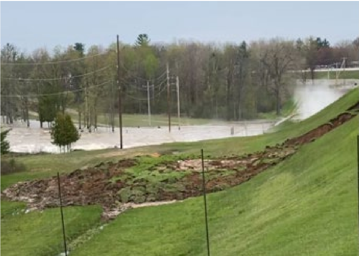
Figure 15: Enlarged still image from dam failure video at 15 seconds
