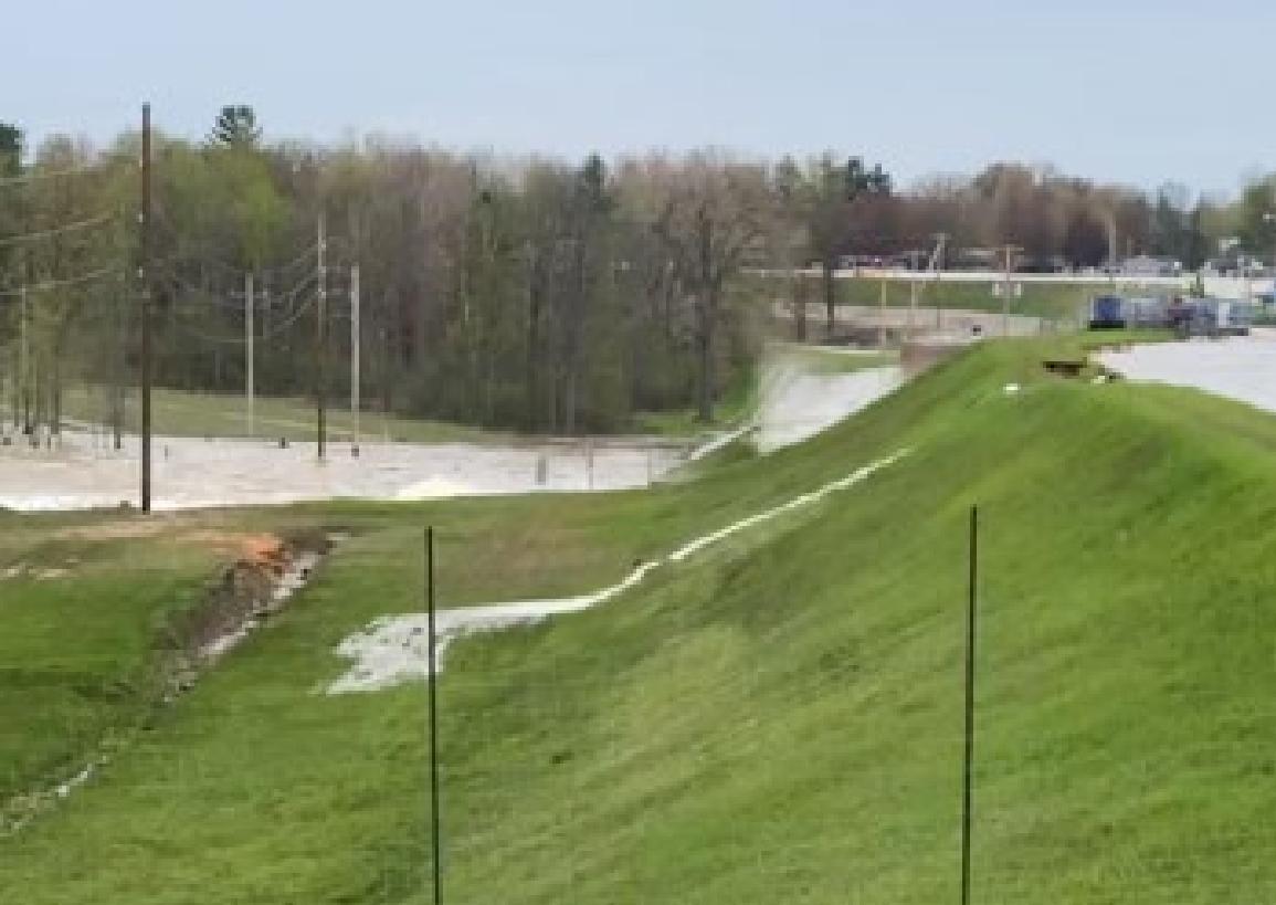
Figure 10: Enlarged still image from dam failure video at 4 seconds
