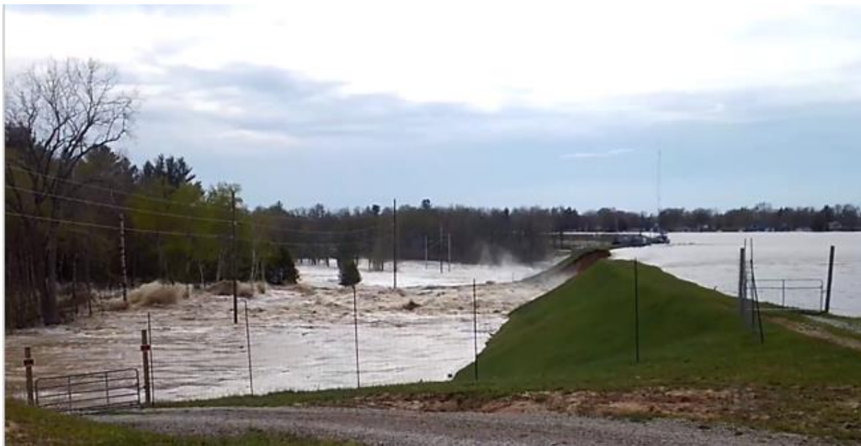
Figure 3-15: Edenville Left Embankment Breach at 6:00 P.M. on Tuesday, May 19, 2020
