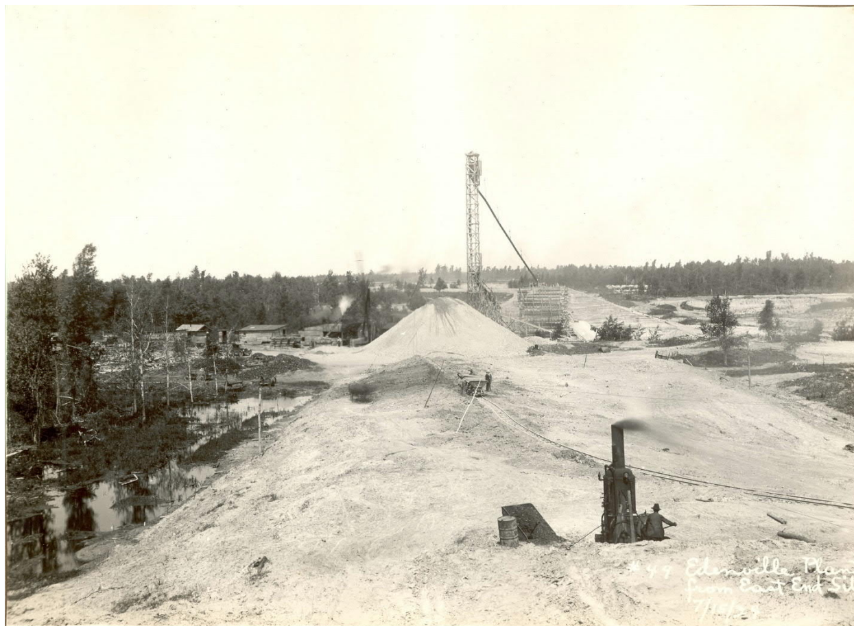
Fill placed in lower portion of Edenville east (left) embankment. Note material in background being stockpiled in downstream portion of the embankment. Note in this photo the rail car from the east is placing fill in the downstream area and the apparent color variation in that area. (July 1924)
