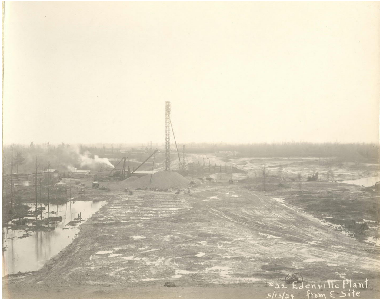
Fill placed near the foundation level of Edenville east (left) embankment. Note stockpile of material in background in downstream portion of the embankment and what appears to be linear alignments of foundation drains. (May 1924)
