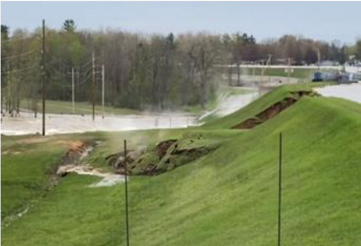
Figure 3-10: Enlarged Still Image from Dam Failure Video at 8 Seconds
