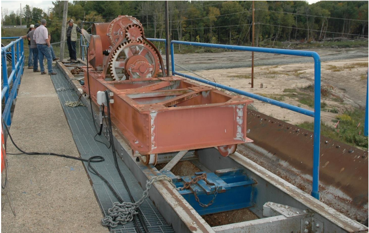
Figure 2-4: Electric Hoist at Edenville
