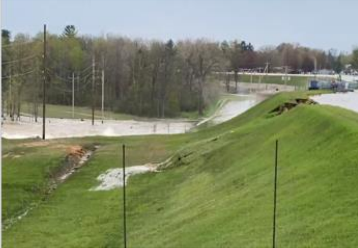
Figure 3-8: Enlarged Still Image from Dam Failure Video at 6 Seconds
