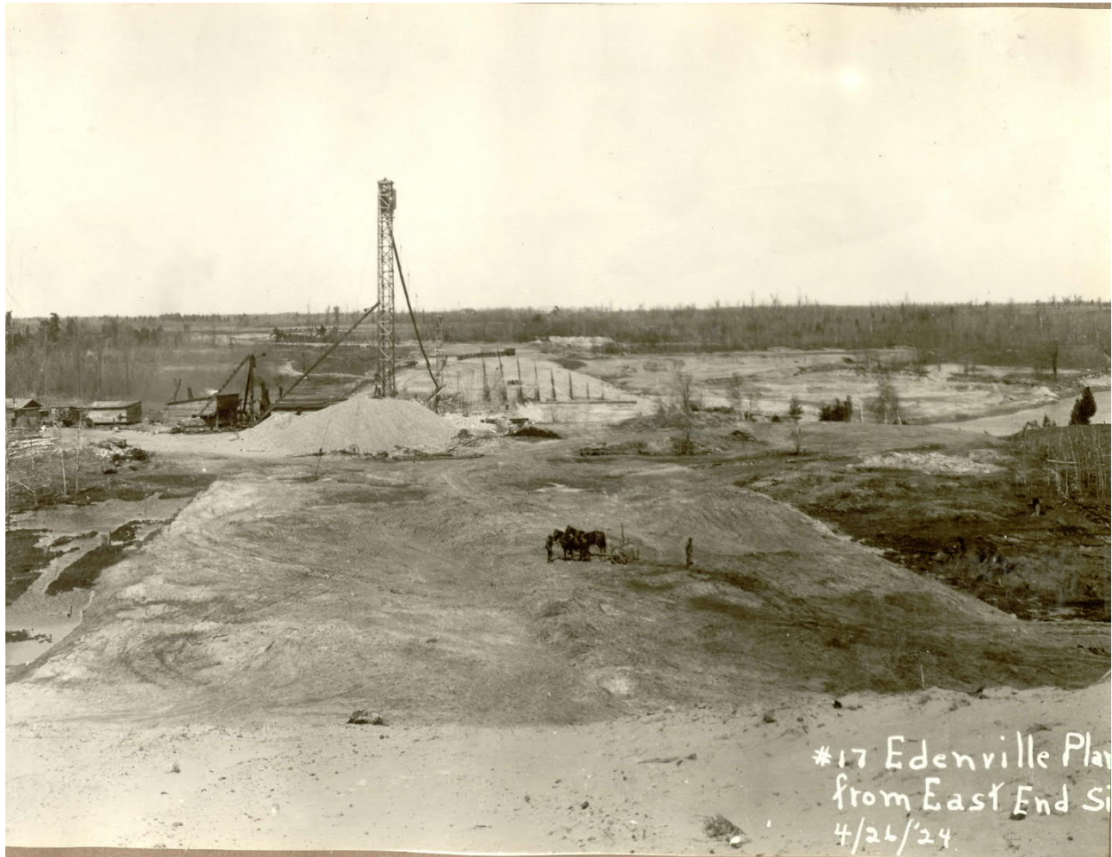
Fill placed near the foundation level of Edenville east (left) embankment. Note stockpile of material in background in downstream portion of the embankment. (April 1924)
