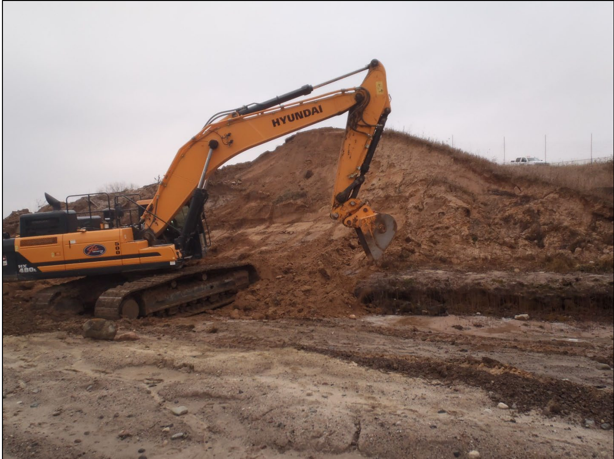
Figure E-4: Excavator Removing Loose Fill and Debris from the Face of the Left Breach Remnant
