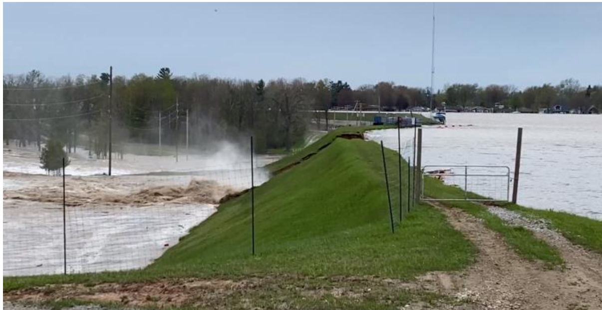
Figure 3-14: Enlarged Still Image from Dam Failure Video at 36 Seconds
