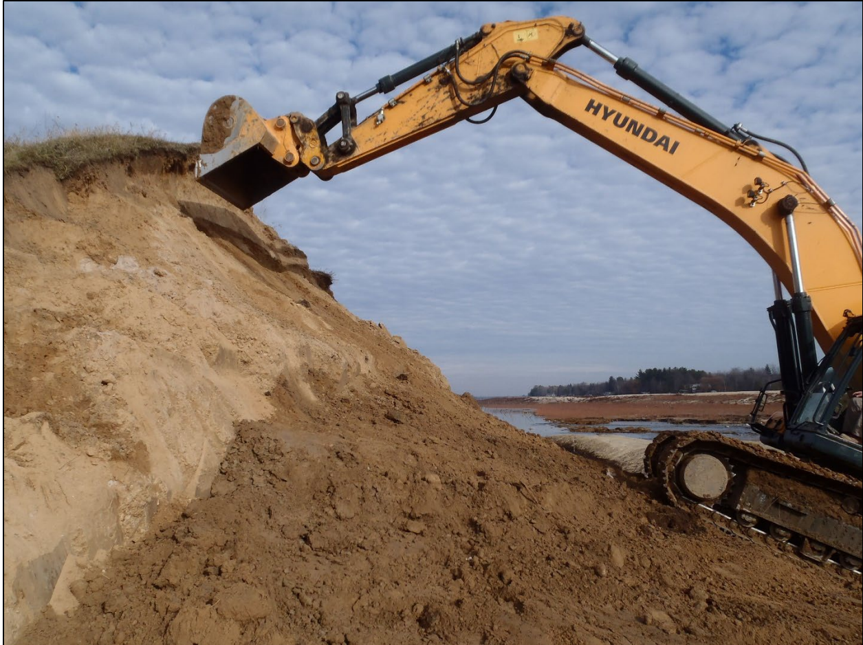
Figure E-5: Excavator Removing Loose Fill from the Face of the Right Breach Remnant, near the Crest
