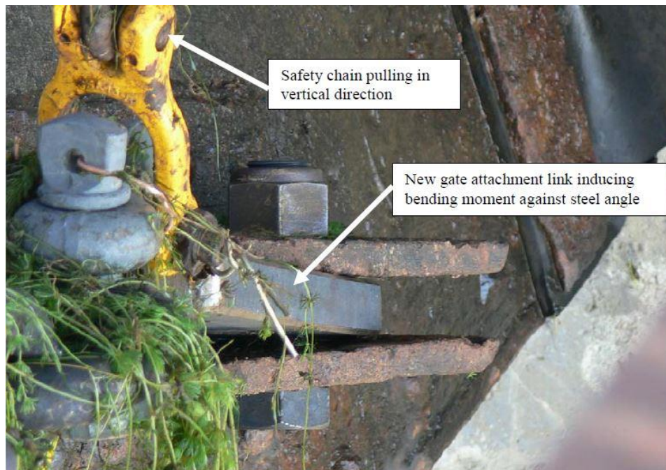
Figure 2-9: A-Frame Induced Bending at Connection to Gate (Spicer 2019)
