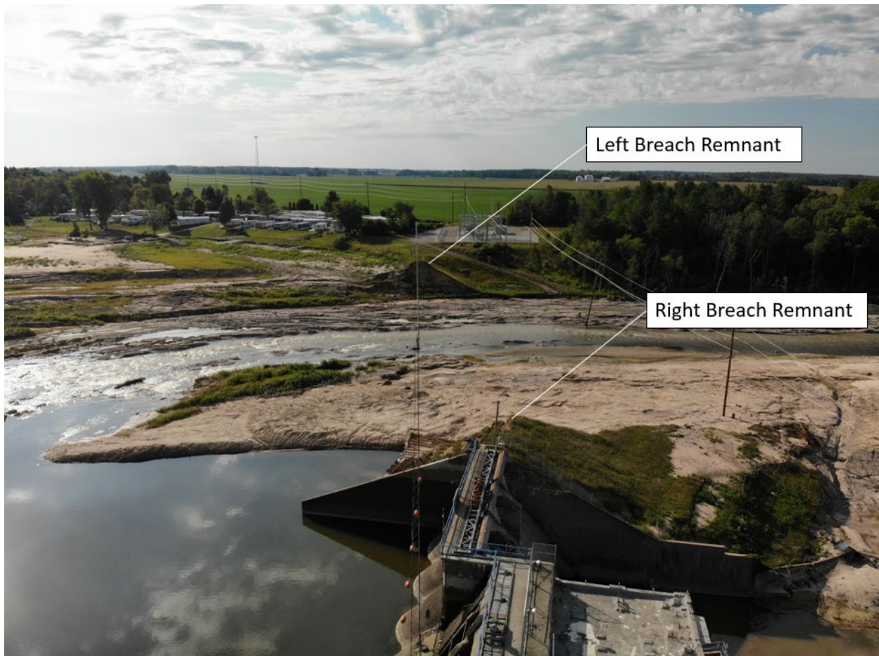
Figure E-1: View of Edenville Left Embankment, Post Failure (photo courtesy of EGLE)
