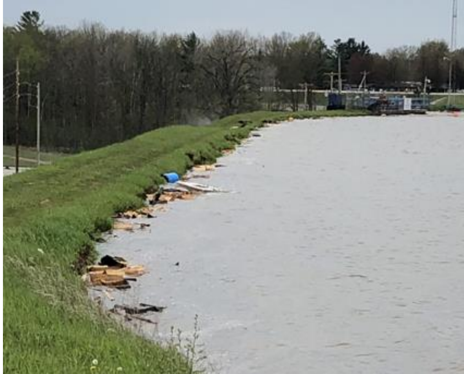
Figure 3-5: Enlarged Photograph Showing the Upstream Side of the Edenville Left Embankment at 5:31 P.M., Tuesday, May 19, 2020
