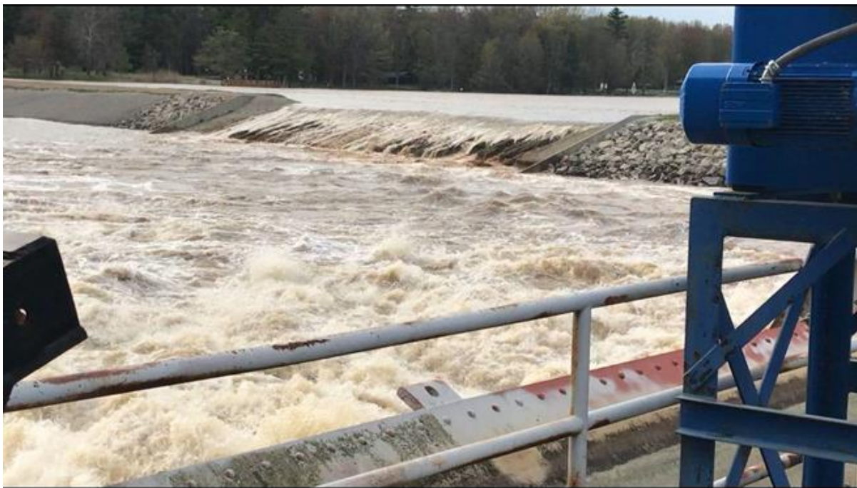
Figure 3-22: Erosion of Fuse Plug Embankment and Head Cutting at about 7:25 P.M. (photo courtesy of EGLE)
