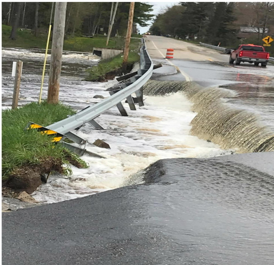
Figure F1-25: Local Roadway Upstream of Secord Dam on May 18, 2020
