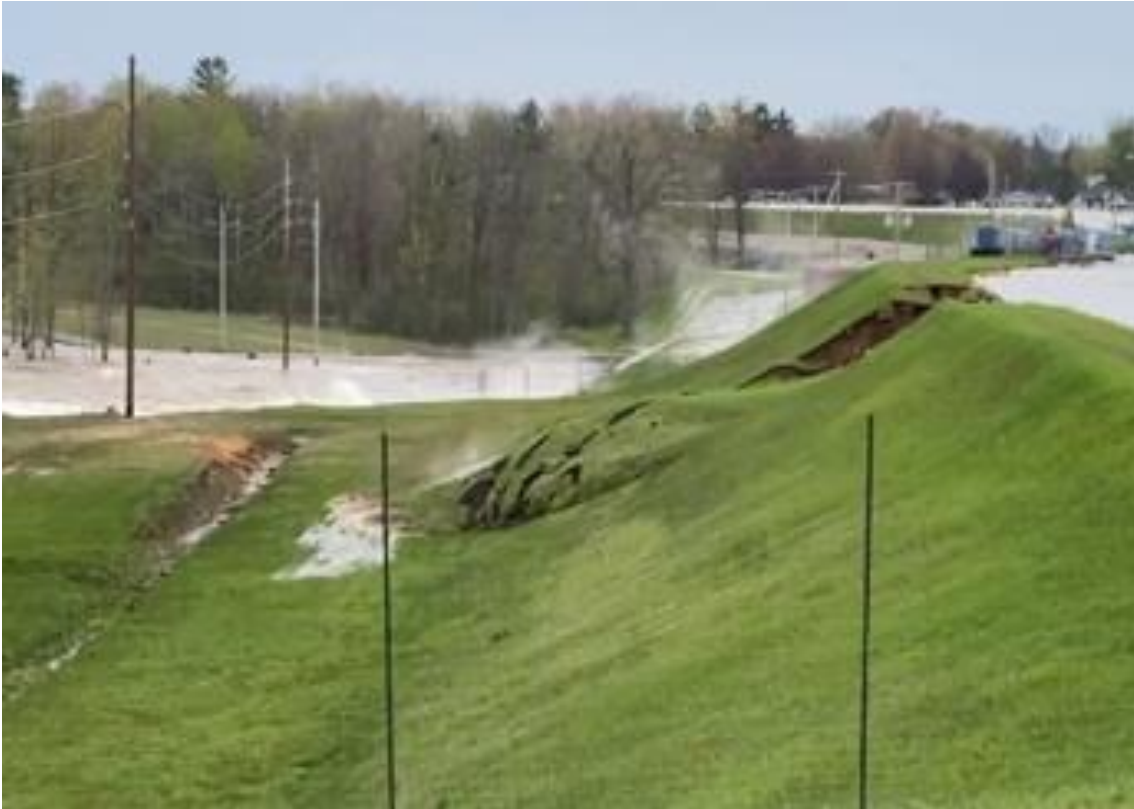
Figure 3-9: Enlarged Still Image from Dam Failure Video at 7 Seconds
