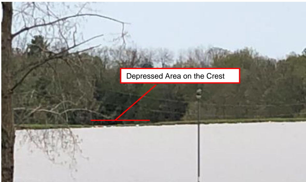
Figure 3-2: Photograph Showing Depression in the Crest of the Edenville Left Embankment at 5:20 P.M., Tuesday, May 19, 2020
