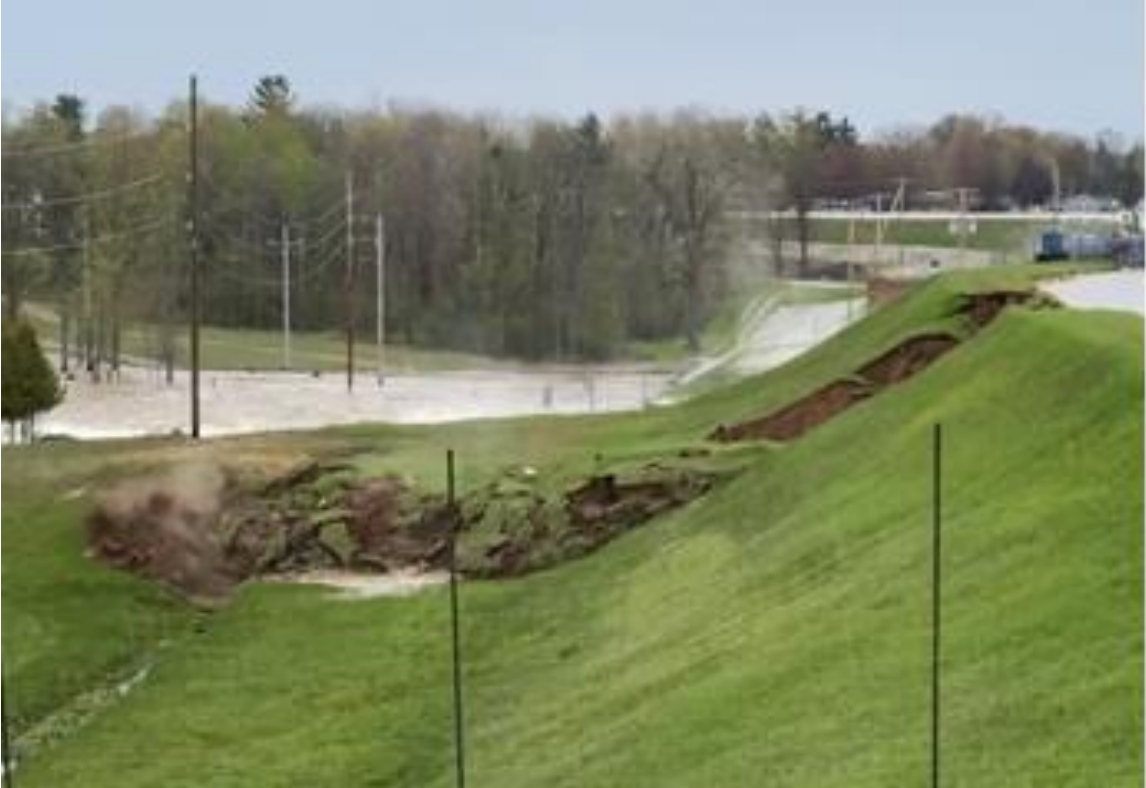
Figure 3-11: Enlarged Still Image from Dam Failure Video at 10 Seconds
