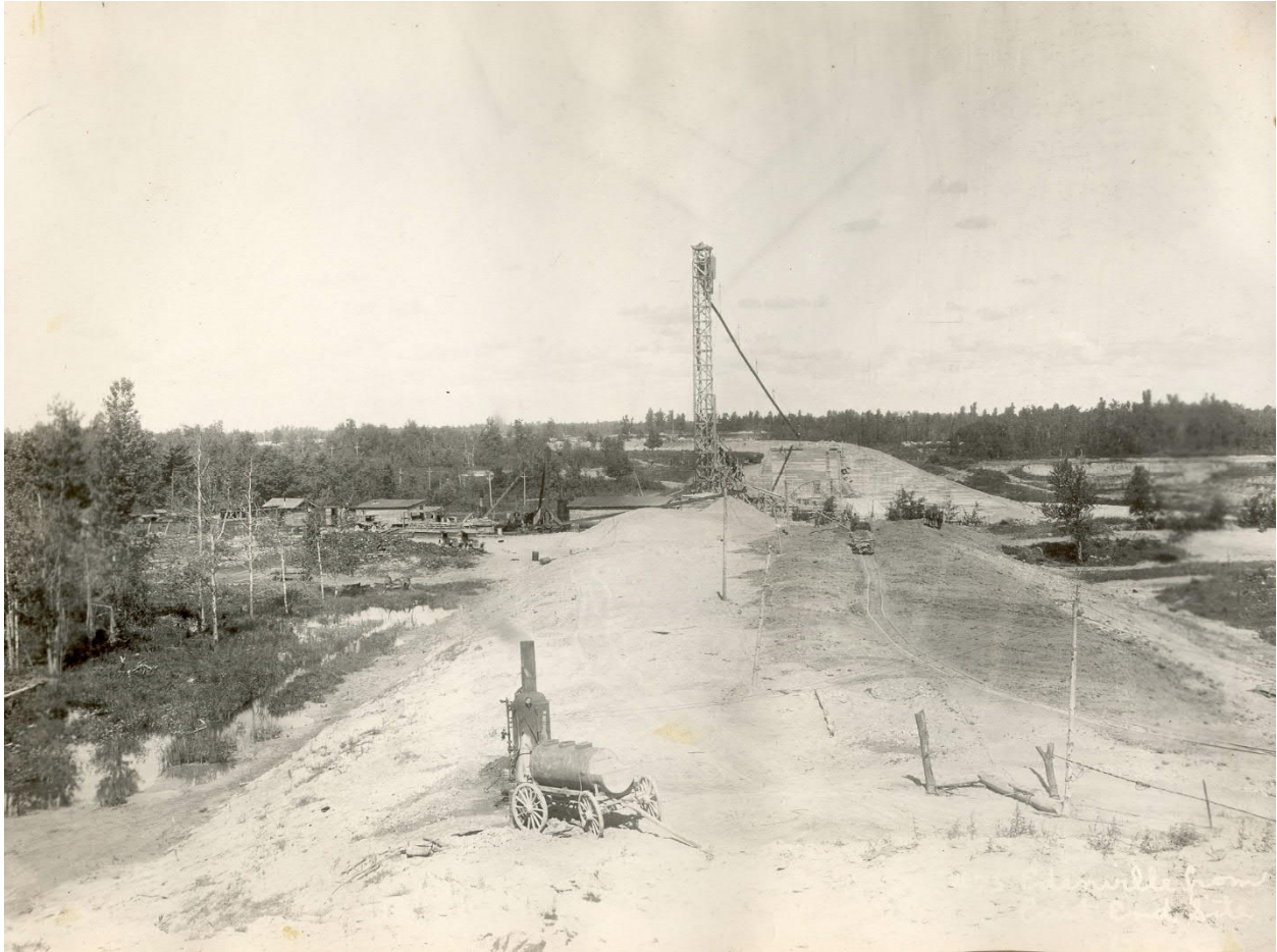
Fill placed in lower portion of Edenville east (left) embankment. Note material in background stockpiled in downstream portion of the embankment. Note the apparent color variation between upstream and downstream areas of the embankment. (no date)
