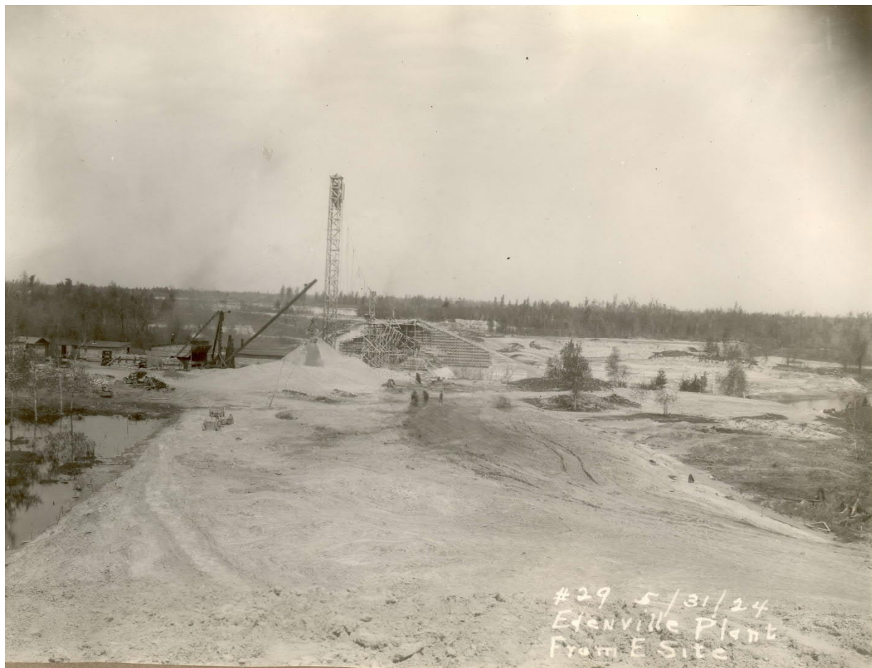
Fill placed in lower portion of Edenville east (left) embankment. Note material in background being stockpiled with clam-shell bucket in downstream portion of the embankment. Foundation drain pipes are visible along the downstream toe. Note the apparent color variation between upstream and downstream areas of the embankment. (May 1924)
