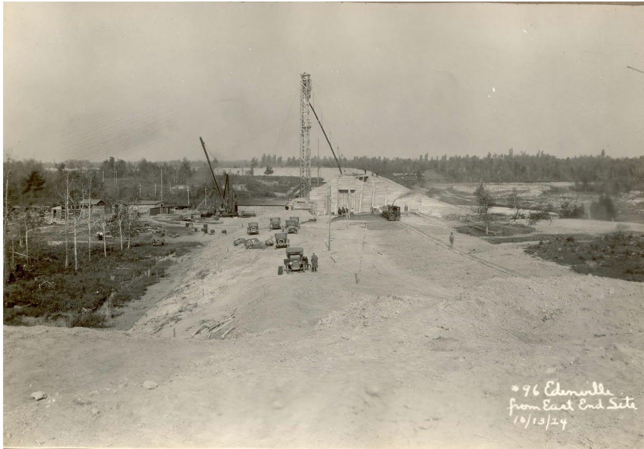
Fill placed in Edenville east (left) embankment. Note the apparent color variation between upstream and downstream areas of the embankment. (October 1924)
