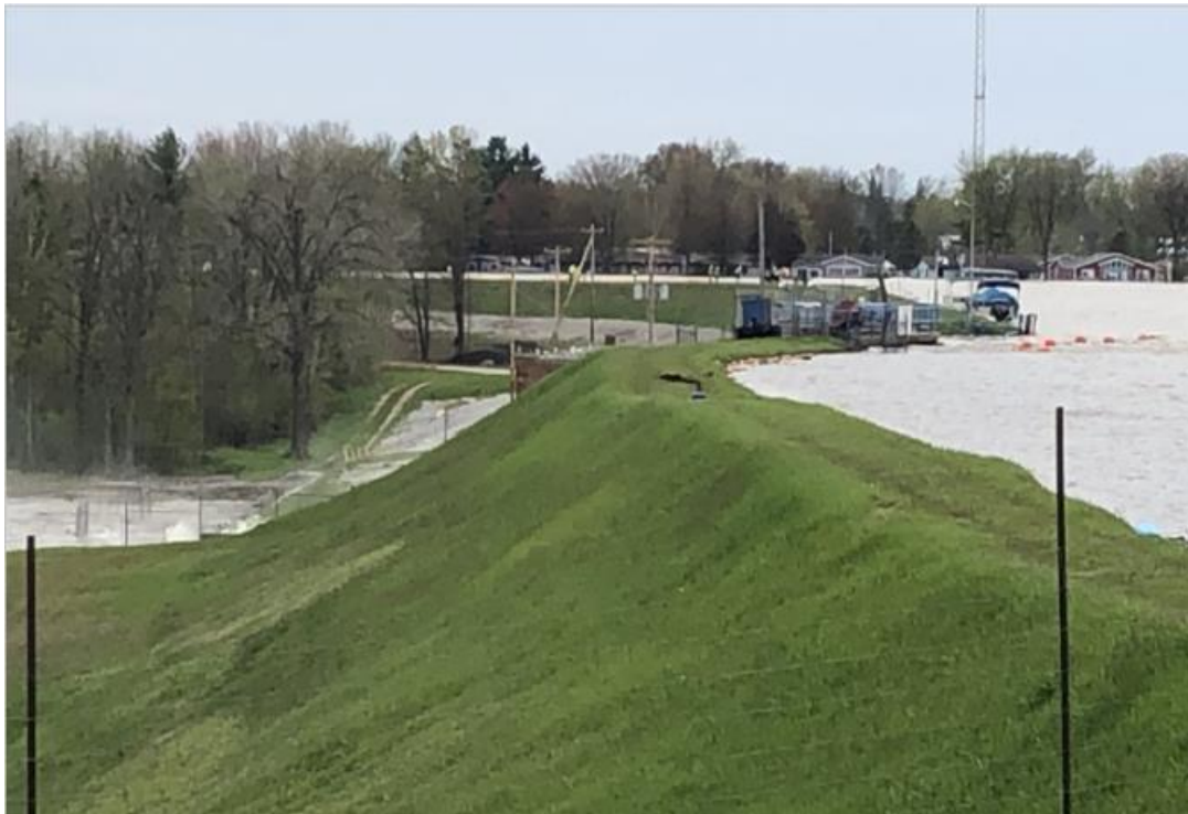
Figure 3-4: Photograph Showing the Downstream Side of the Edenville Left Embankment at 5:31 P.M., Tuesday, May 19, 2020
