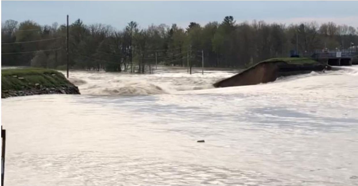
Figure 3-17: Edenville Left Embankment Breach at 7:13 P.M. on Tuesday, May 19, 2020
