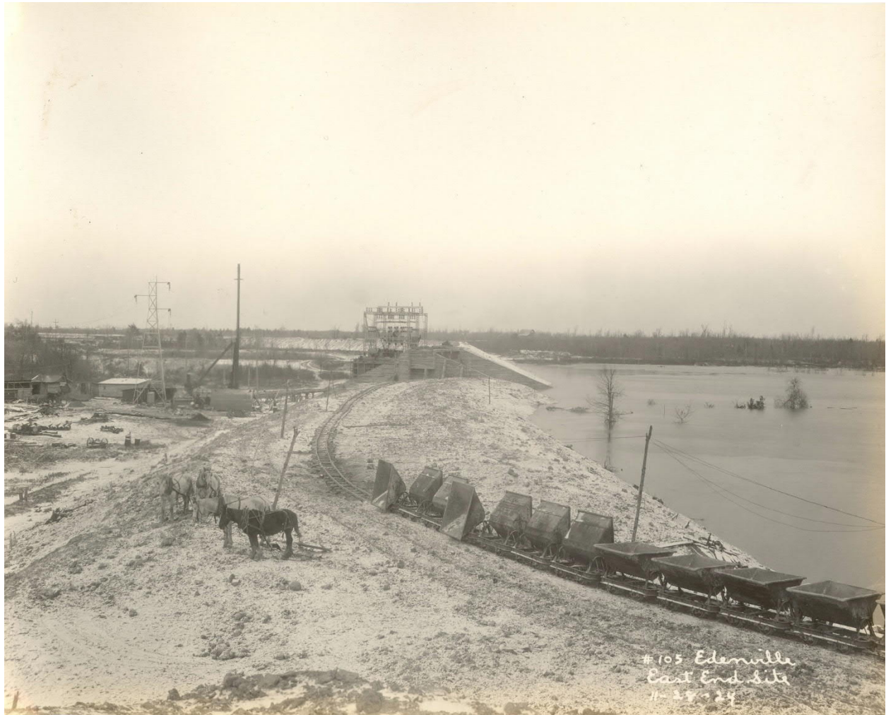
Fill placed in Edenville east (left) embankment. Note material previously stockpiled in the background is no longer visibly present. Note cold-weather fill placement on snow-covered ground. Note rising lake level in comparison to earlier photo. (November 1924)
