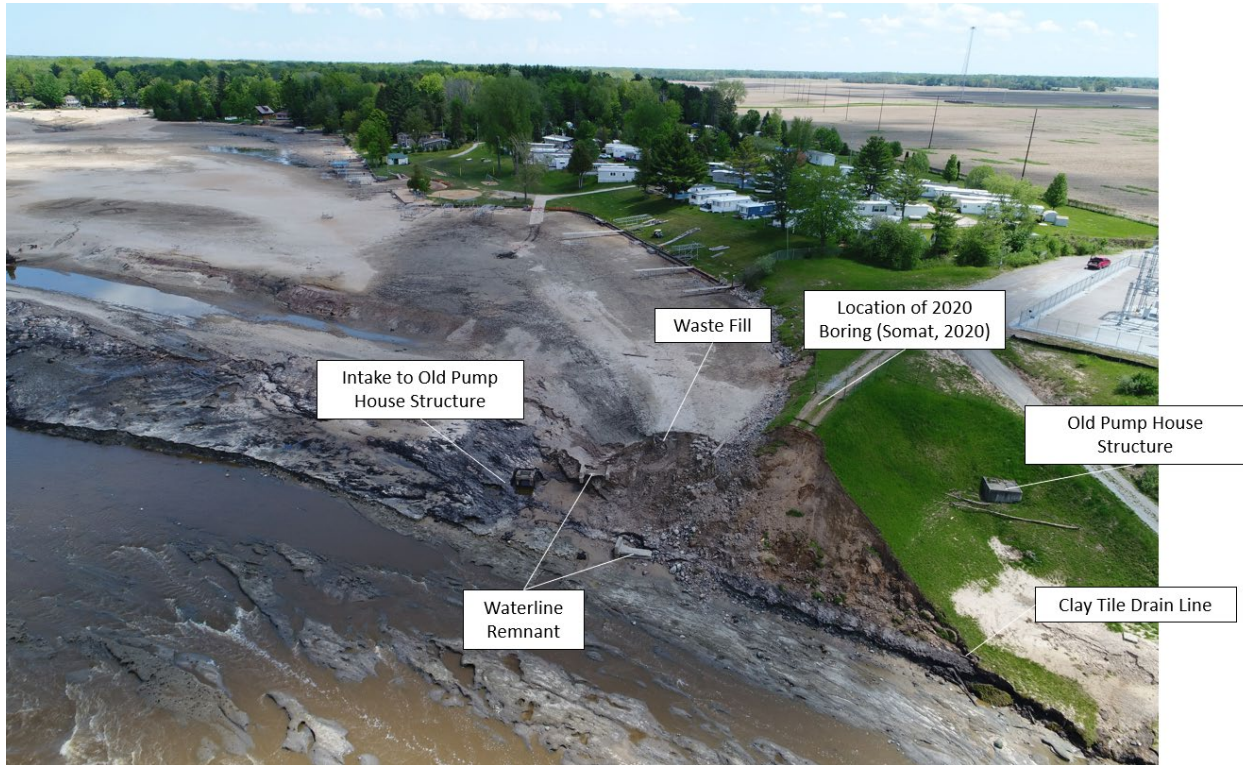
Figure E-2: Aerial View of Left Breach Remnant (photo courtesy of EGLE)
