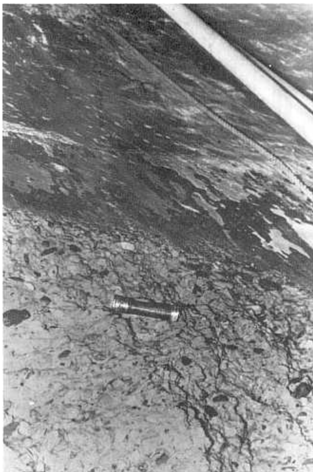
FIGURE 7-8.—Hoover Dam, Arizona tunnel spillway — misalignment that caused major damage.
