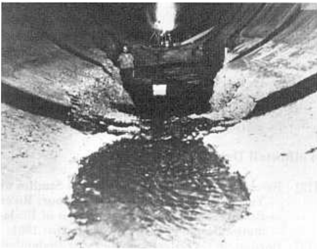
FIGURE 7-13.— Yellowtail Dam, tunnel spillway — major damage downstream of elbow.
