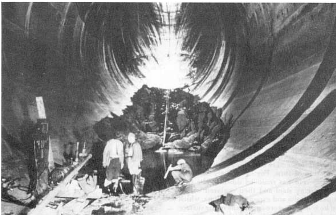
FIGURE 7-7.—Hoover Dam, Arizona tunnel spillway — major damage (1942).
