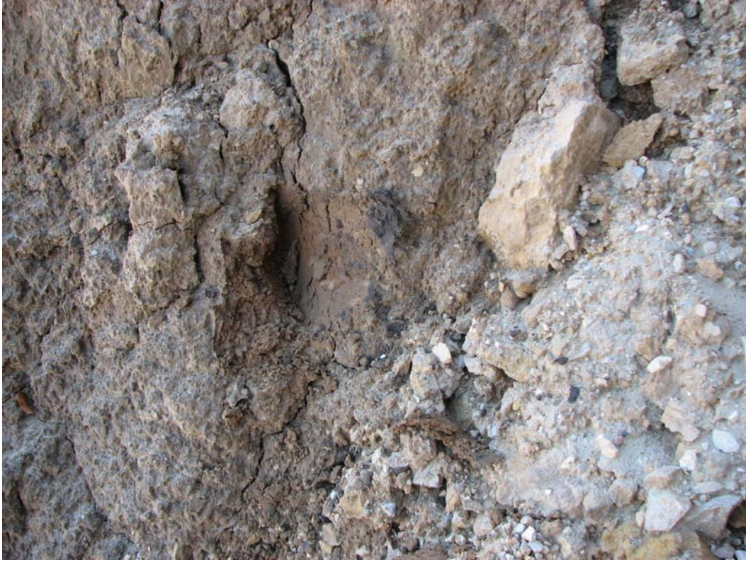
Photo IV-3 Close up of exposed embankment material.
