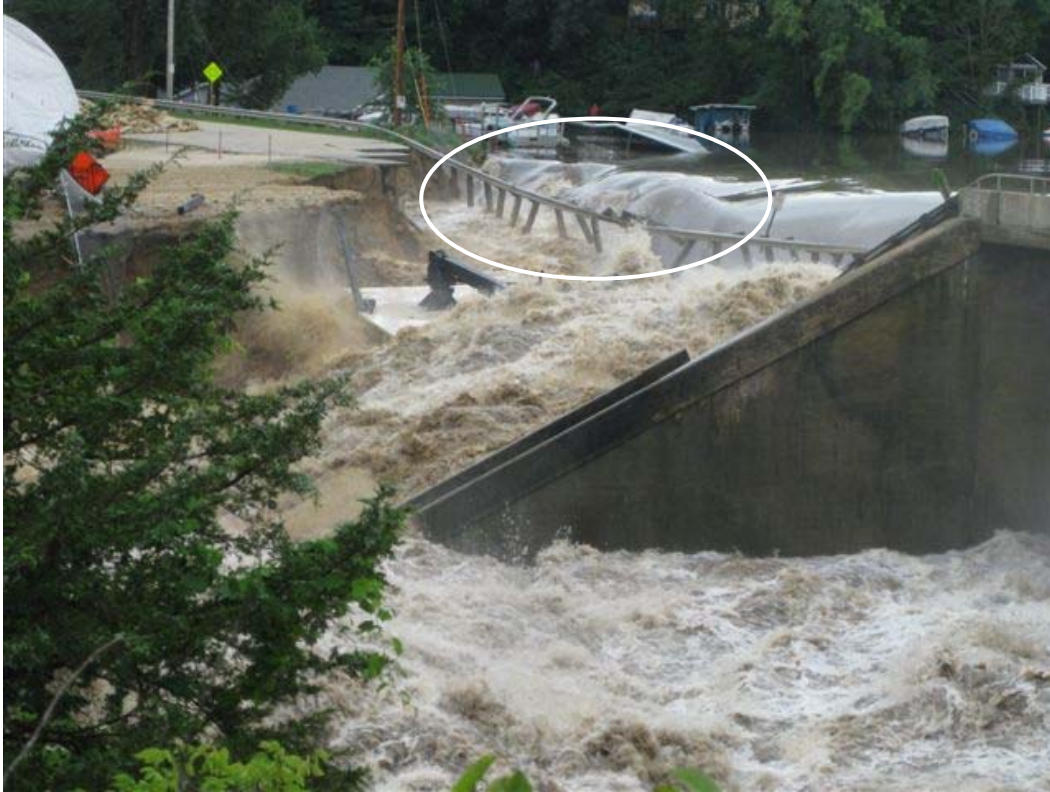
Photo IV-19 Continued breach development showing expected core wall location Note advancing erosion in original embankment section (photo by T. McCarthy).
