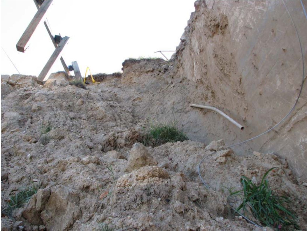
Photo IV-10 Fill material downstream of core wall at breach. Note coarser fill material above top of core wall.
