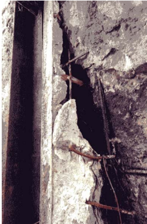
Photo III-5 Damage to spillway pier adjacent to Gate 3 left side guide [Stanley 2010]
