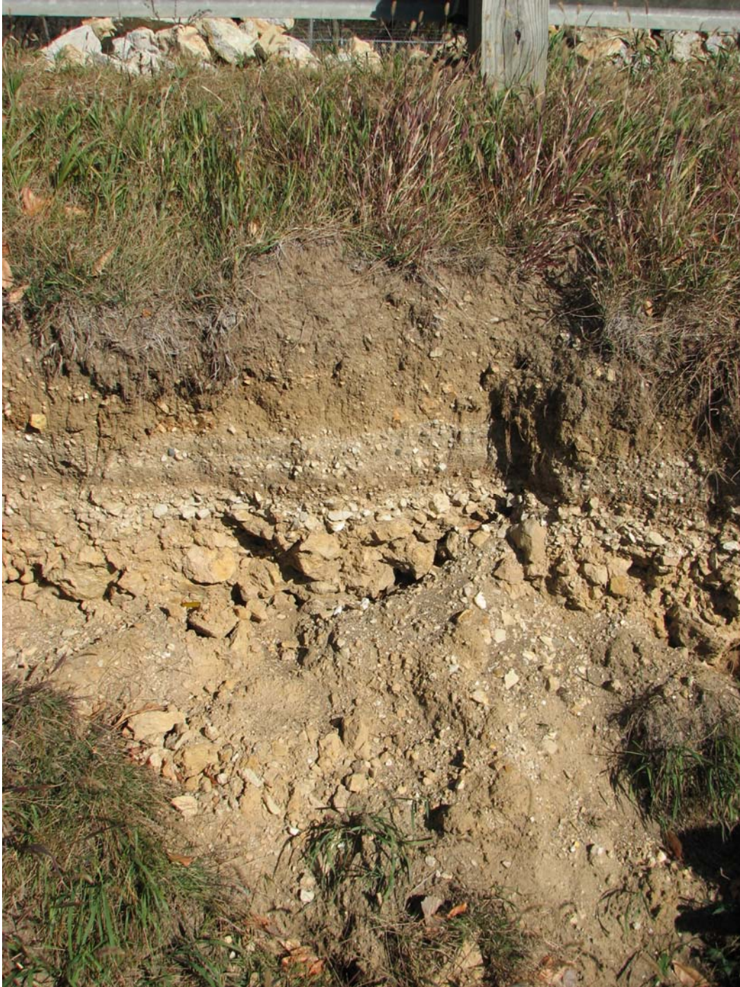
Photo IV-11 Coarse material observed above the top of core wall at the remaining sinkhole
