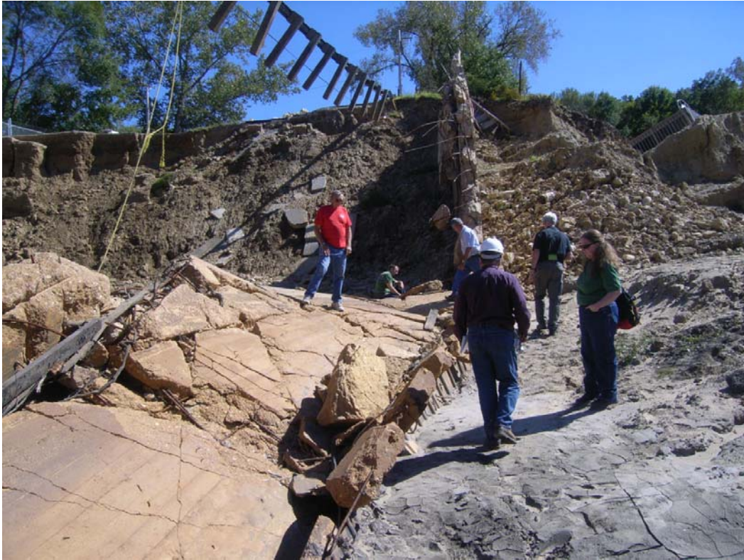
Photo IV-2. Exposed embankment material post-breach.
