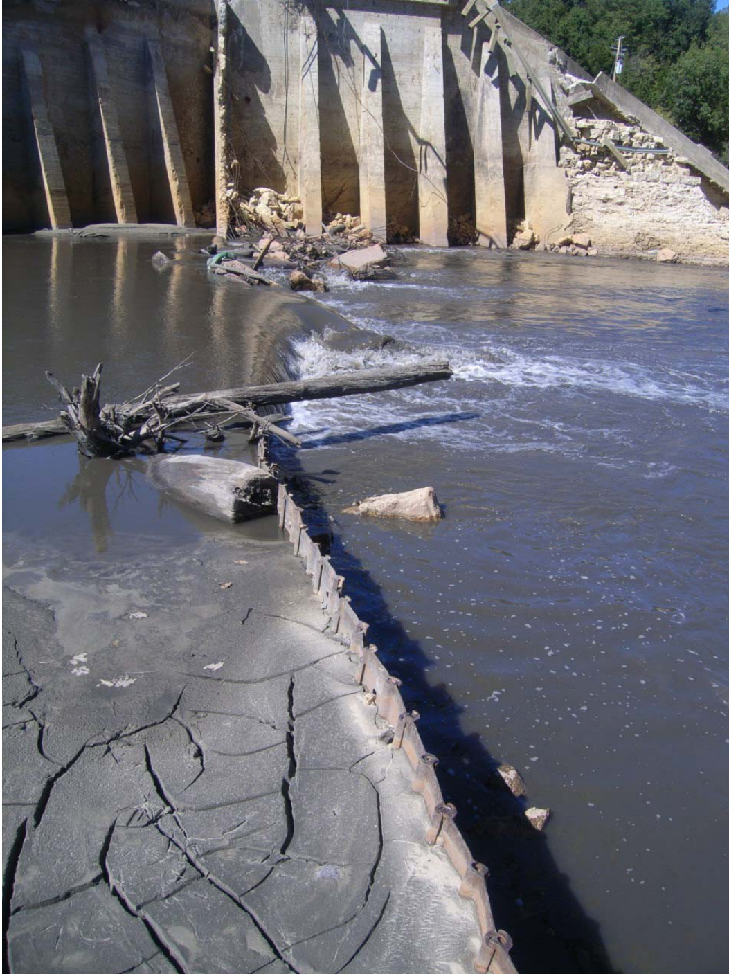
Photo II-3. Breach area Note Embankment core wall remnant at gated spillway and sheet pile.
