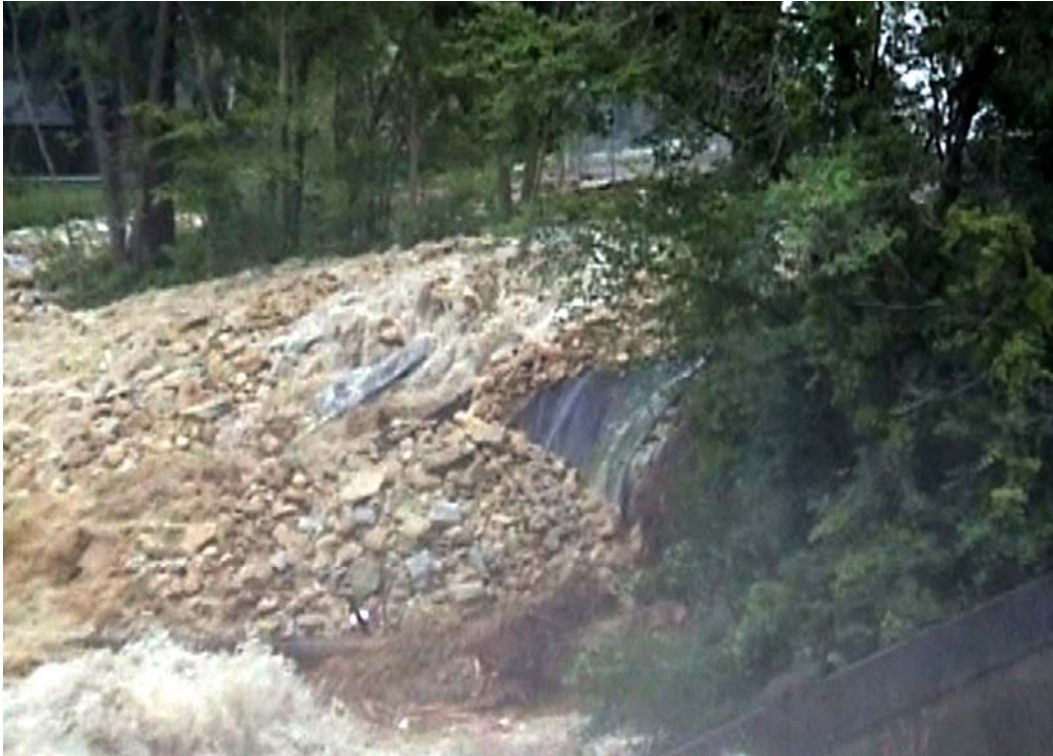
Photo IV-8 Overtopping flow and discolored discharge from beneath geotextile (still photo captured from amateur video).
