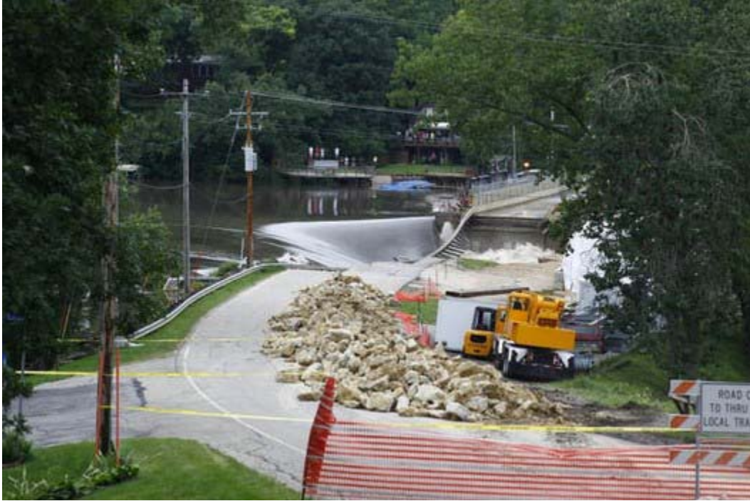
Photo IV-20. Breach expanding in width with loss of core wall (photo from DesMoinesRegister.com).
