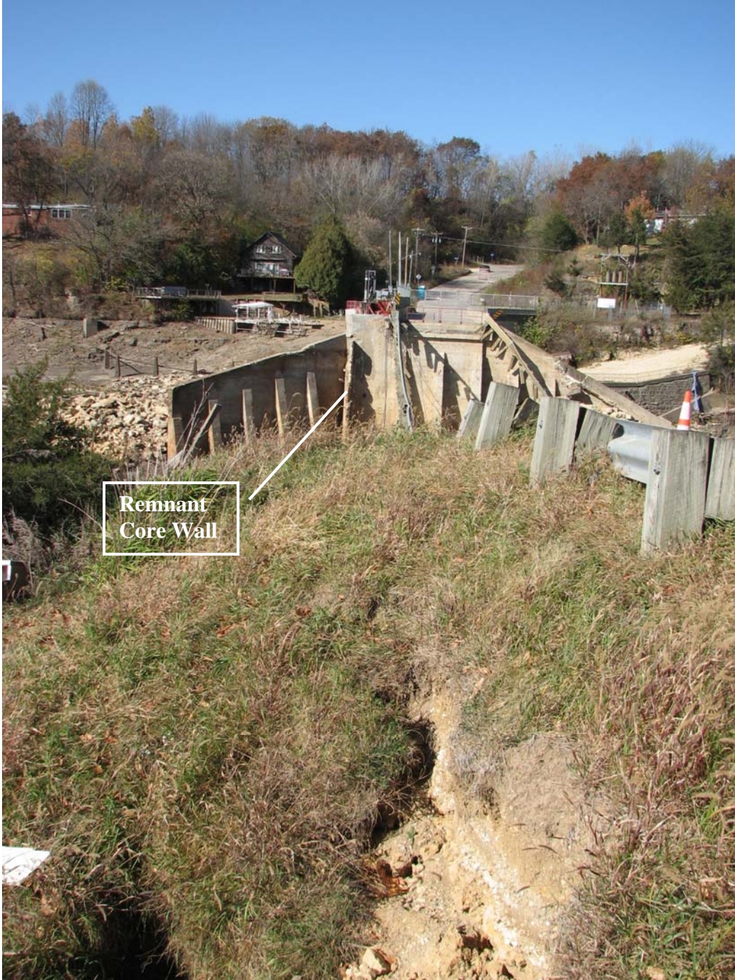
Photo IV-13 Developing sinkhole location in line with remnant core wall.
