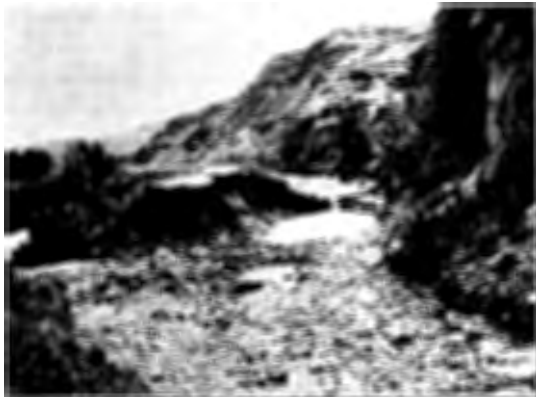
LEFT: One of the major breaks on the main Two Medicine canal. This photo was taken shortly after the flood of June 8, 1964.
