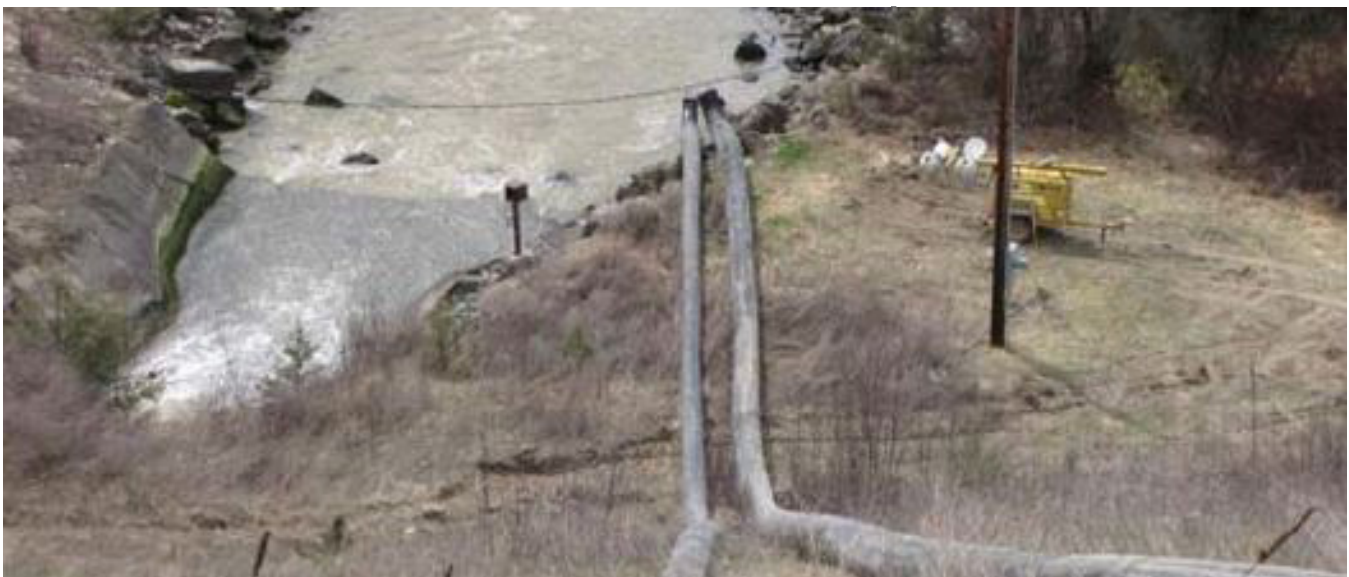
Figure 11: Pump Outlet Piping Along the Downstream Slope of Dam and Discharge Location
