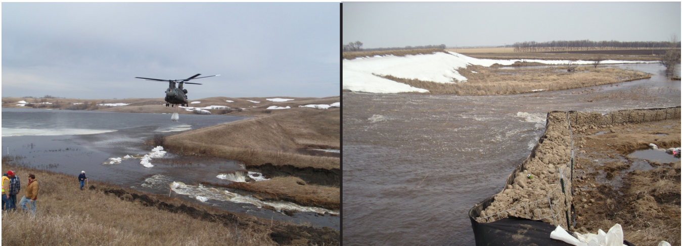
Figure 28: Photographs showing examples of the use of sandbags and rock filled gabions to divert flows in eroding auxiliary spillways.
