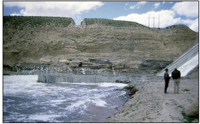
Figure 2B. A photo of the abutment downstream of the spillway. The seepage pattern illustrates the permeability and layering in the foundation.
