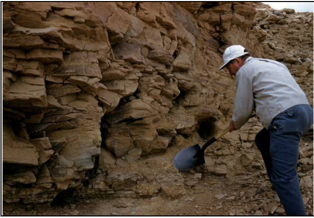
Figure 2A. A photo from right abutment site exploration in the 1950's showing the fractured nature of the foundation.
