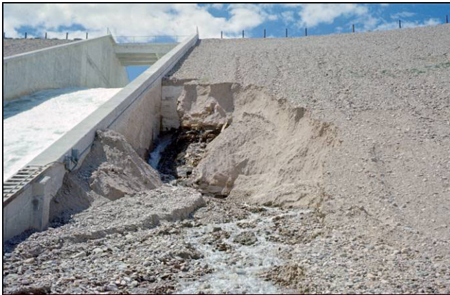
Figure 7A. Seepage emerging from the shale formation along the left side of the spillway chute, July 28, 1965.
