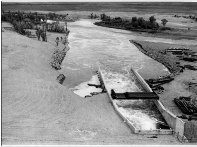
Figure 6A. Failure of the backfill on the left side of the river outlet stilling basin, May 30, 1964
