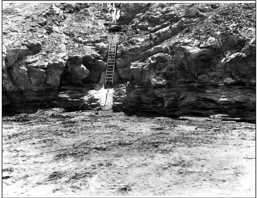
Figure 4B. A photo showing embankment construction along the right abutment. Note the steepness of the foundation and the narrowness of the grout cap under the ladder.
