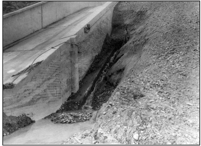
Figure 6B. Seepage emerging from the shale formation along the left side of the spillway chute, May 21, 1965.
