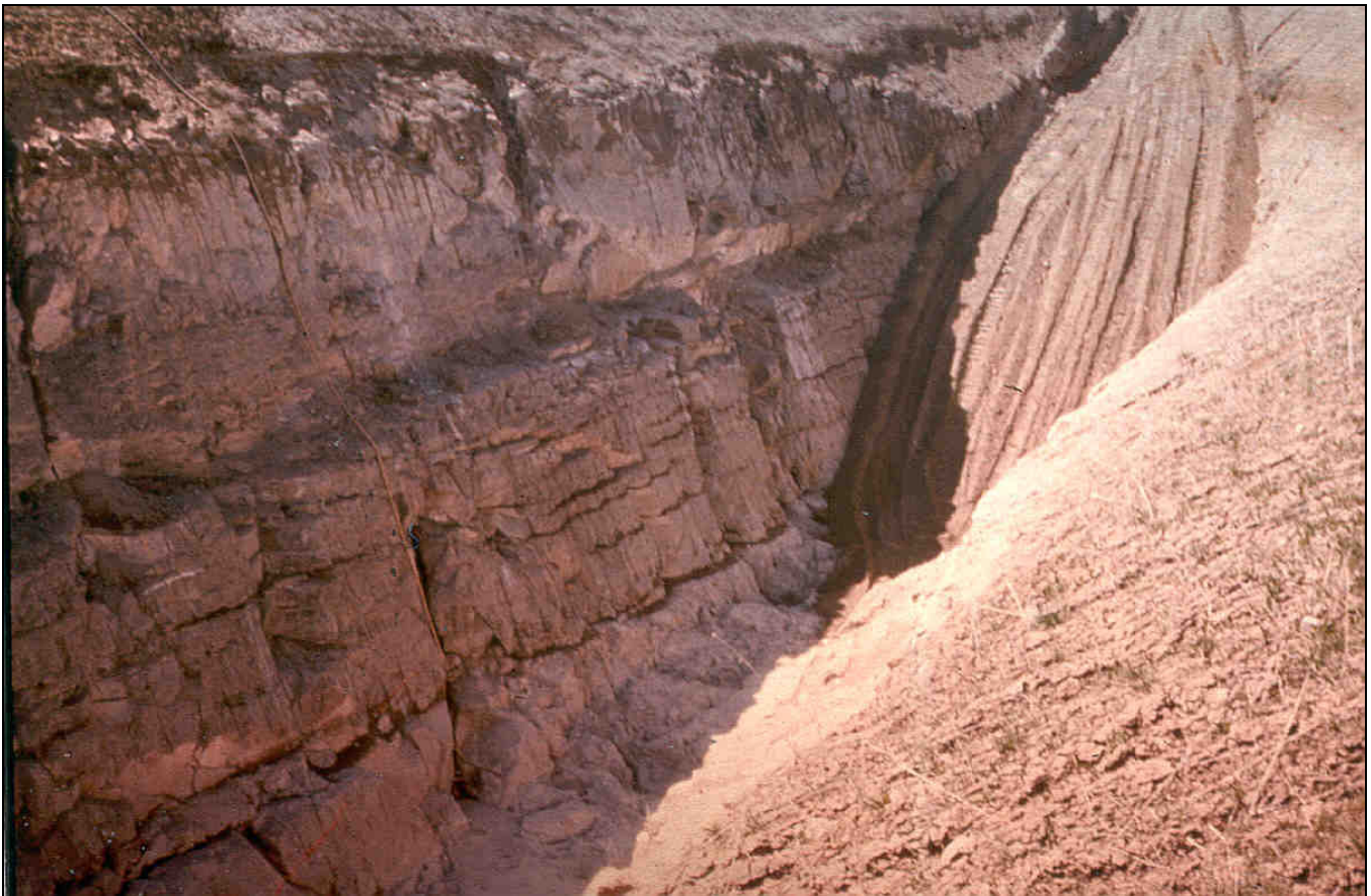
Figure 16. A view of the right abutment key trench showing the jointed nature of the foundation
