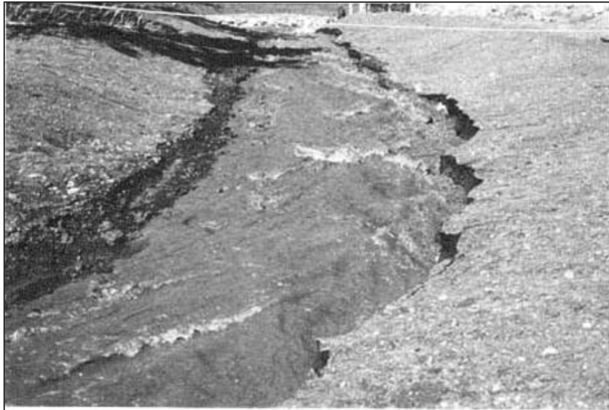
Figure Cottonwood-13.—Flow in the membrane-lined channel during operation. View looking upstream towards the crest with the flat bottom eroded to the edges of the 2:1 side slopes (Reclamation figure republished in Timblin et al., 1988).
