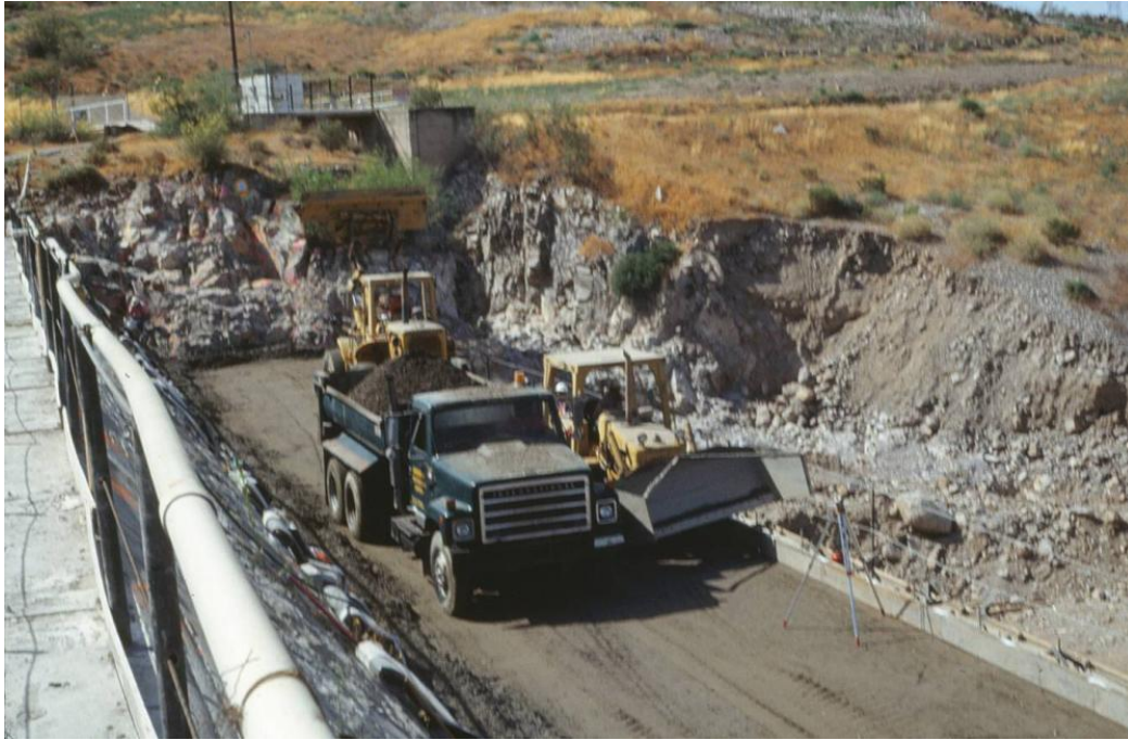
Figure 12-7.—RCC buttress being constructed at downstream face of Camp Dyer Diversion Dam. Width of RCC placement is sufficient for passing construction equipment. Note flat drains on contact surface between dam and buttress. (Reclamation)
