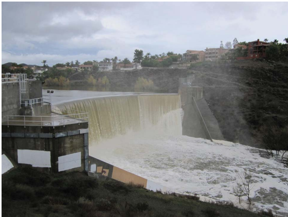
Figure Railroad Canyon-1.—Railroad Canyon Dam during flood event in 2010 (Courtesy of Elsinore Valley Municipal Water District).
