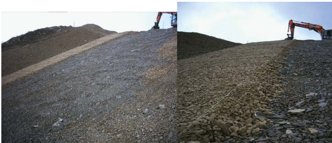
Figure Barriga-8.—Views of the two filter-compatible gravel layers beneath the block system, (a) top bedding layer (left) and (b) bottom drainage layer (right) (courtesy of Morán and Toledo, 2006, all rights reserved).
