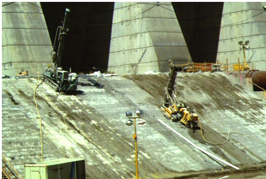
Figure 12-6.—Mechanical anchors being installed through the RCC toe block into the foundation for Pueblo Dam spillway, to improve sliding resistance (Reclamation).
