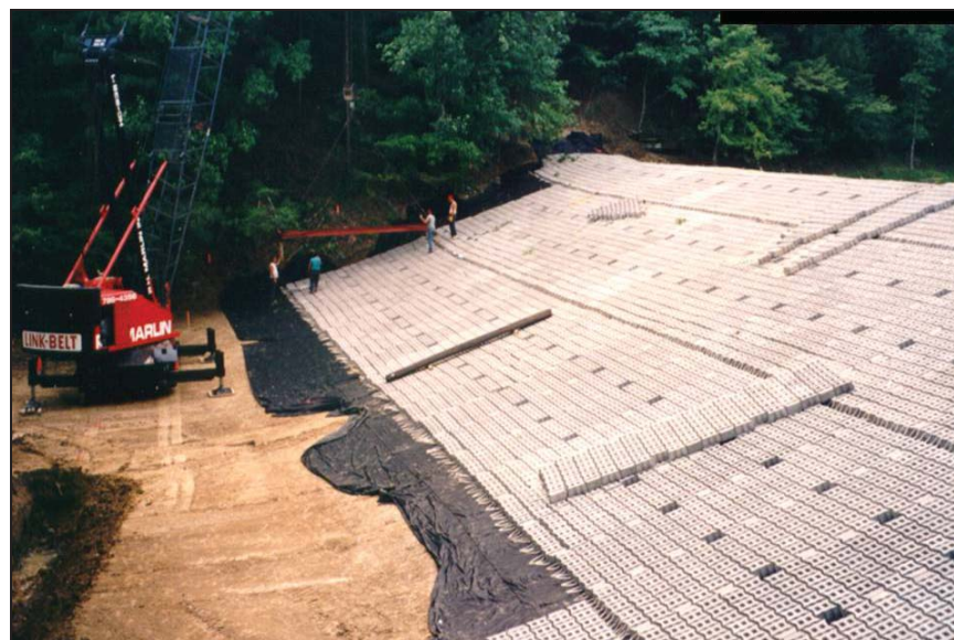
Figure Strahl-2.—Placement of the cable-tied mats over a geotextile on the downstream face of Strahl Lake Dam (Courtesy of Contech Engineering Solutions, all rights reserved).
