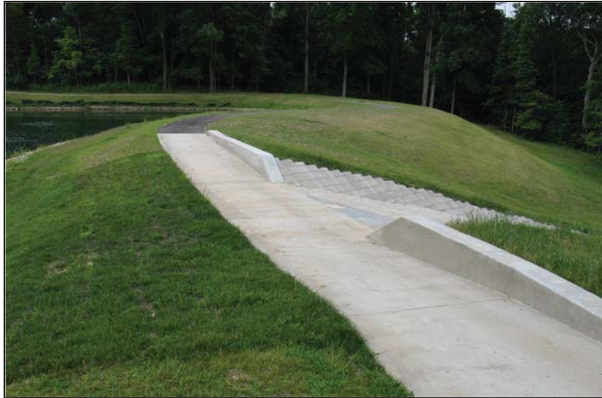
Figure Friendship Village-3.—Finished crest forming a sidewalk for the lake and the top of the ArmorWedge block spillway (courtesy of Contech Engineering Solutions, all rights reserved).
