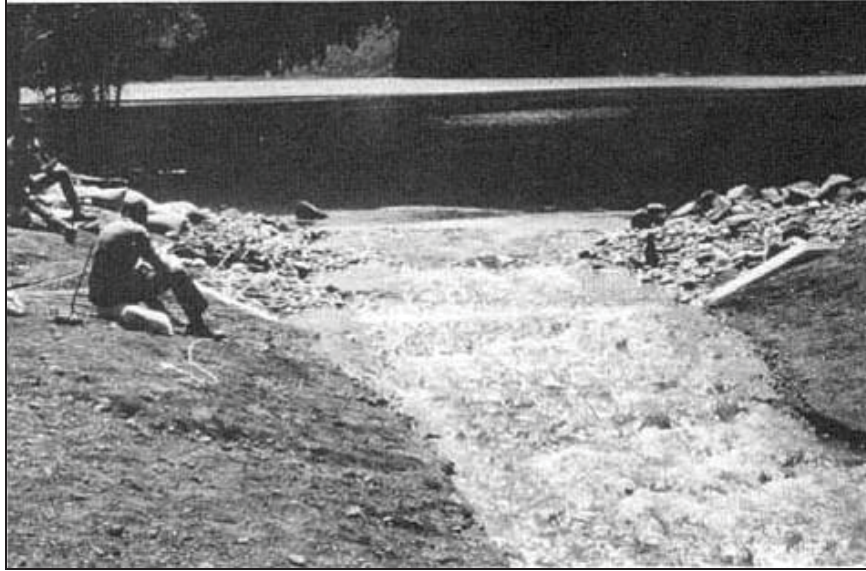
Figure Cottonwood-12.—Flow over spillway crest during operational test. The flow was estimated to be 21 to 25 ft 3 /s at a maximum velocity of 19 to 26 ft/s (Reclamation figure republished in Timblin et al., 1988).
