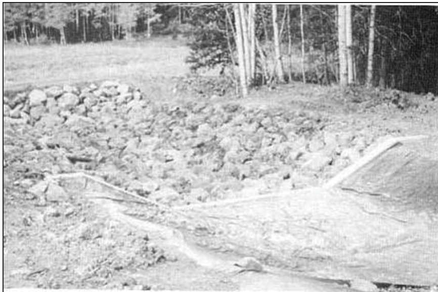
Figure Cottonwood-7.—Downstream end of geomembrane-lined spillway. Note concrete cutoff wall (Reclamation figure republished in Timblin et al., 1988).
