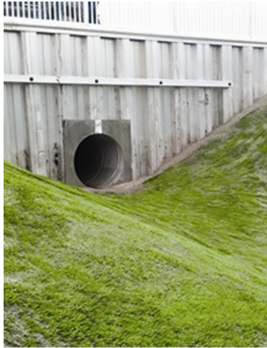
Figure 6.1.—HydroTurf™ Outfall Structure with St. Johns River Water Management District in Florida (Courtesy of Watershed Geo, all rights reserved).
