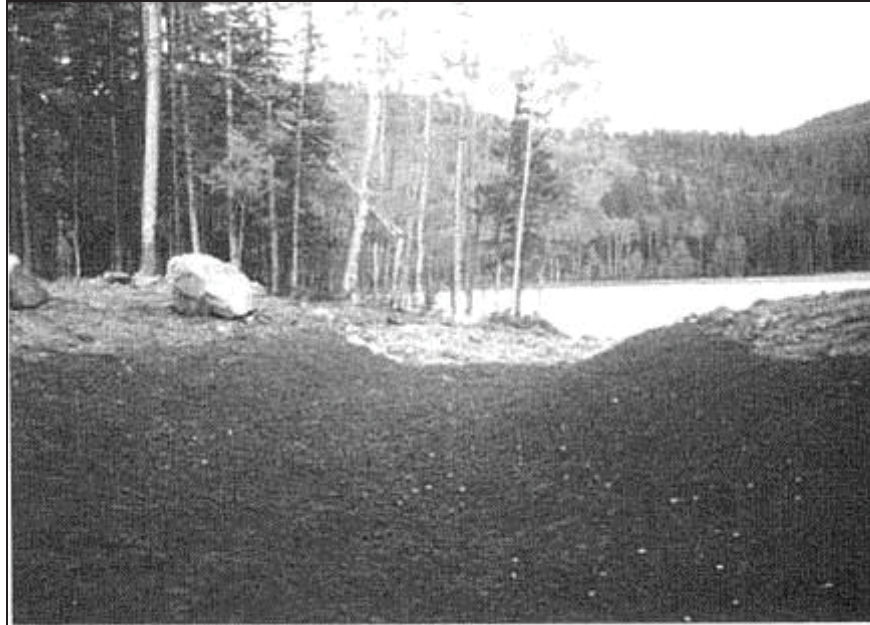
Figure Cottonwood-10.—Completed spillway looking upstream into the reservoir (Reclamation figure republished in Timblin et al., 1988).
