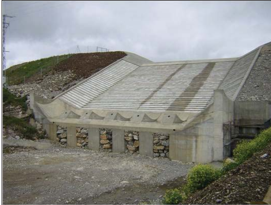
Figure Barriga-14.—Completed spillway prior to operation (courtesy of Morán and Toledo, 2006, all rights reserved).
