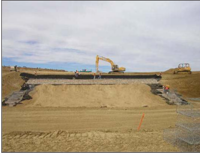
Figure West Cornfield-2.—Dam beginning construction (Courtesy of Maccaferri, Inc., all rights reserved).
