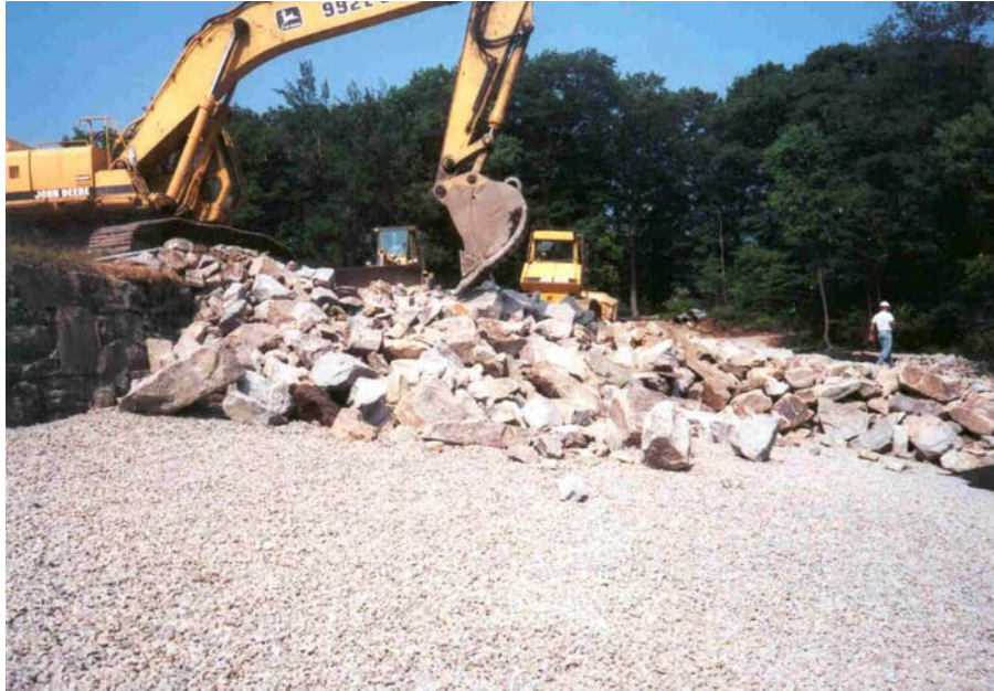
Figure 8-1.— Dumped riprap placement on 6-inch bedding layer for Upper Stoneville Reservoir Dam, Massachusetts (Wooten and Wood, 2002, Courtesy of ASDSO and GEI Consultants, all rights reserved).
