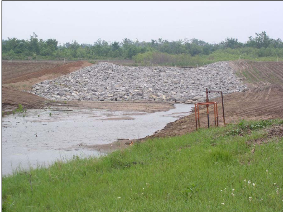
Figure 8-2.—Rock chute spillway on Little Washita Site 13 in Grady County, Oklahoma. This chute was installed in 2010 to convey flows over the remnants of the decommissioned dam (USDA-NRCS, Courtesy of Chris Stoner).
