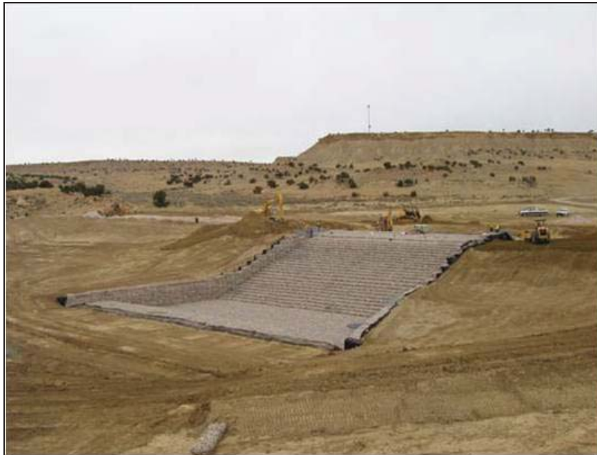
Figure West Cornfield-5.—Construction nearing completion (Courtesy of Maccaferri, Inc., all rights reserved).
