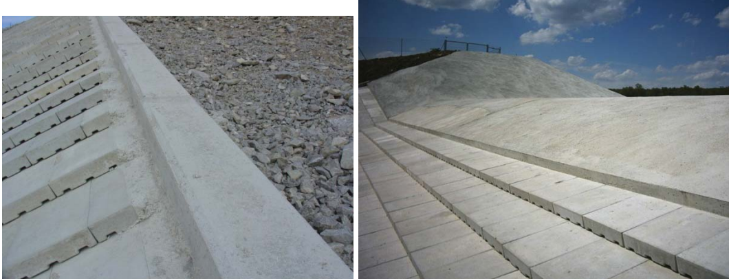
Figure Barriga-13.—View of top caps for the side slope blocks on left and of the completed crest cap on right (courtesy of Morán and Toledo, 2006, all rights reserved).
