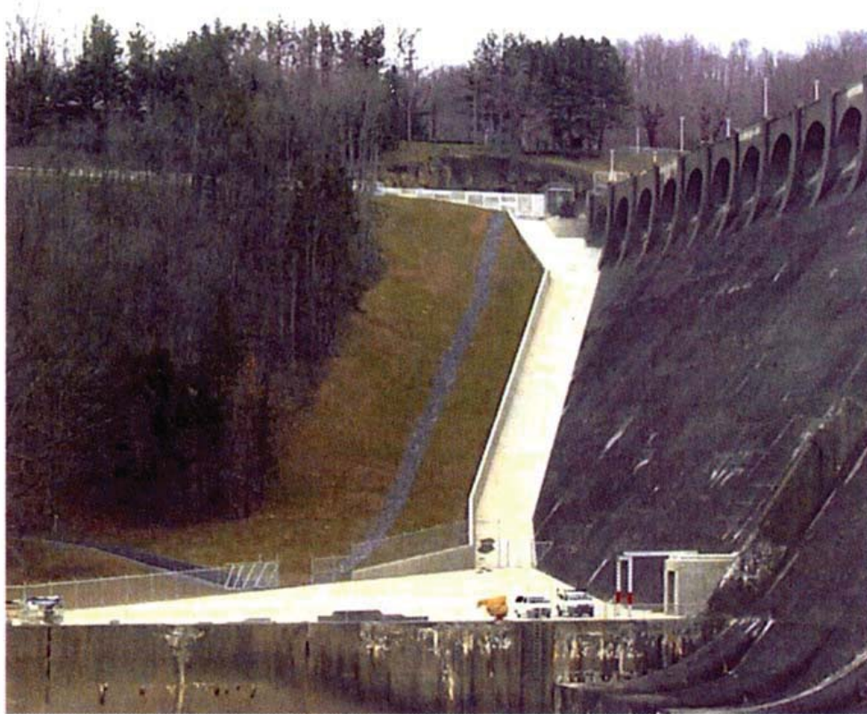
Figure Tygart-1.—Concrete Paving and Channel Along Downstream Right Abutment (Courtesy of USACE).
