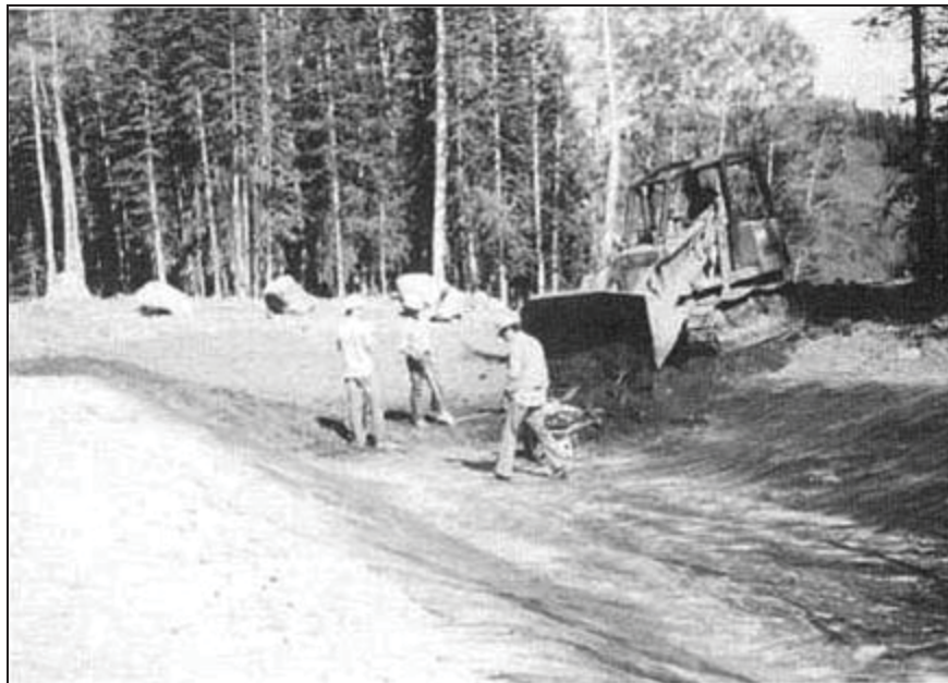
Figure Cottonwood-9.—Placement of soil cover to protect geomembrane liner from the elements and mechanical damage (Reclamation figure republished in Timblin et al., 1988).
