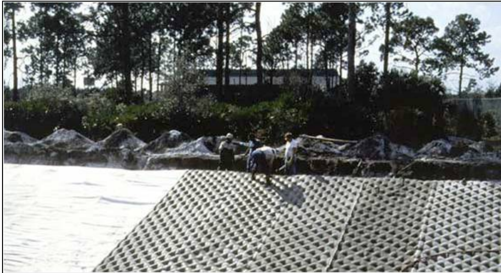
Figure 9-7.—Fabric forms being filled with fine aggregate concrete. (Courtesy of Donnelly Fabricators, all rights reserved).
