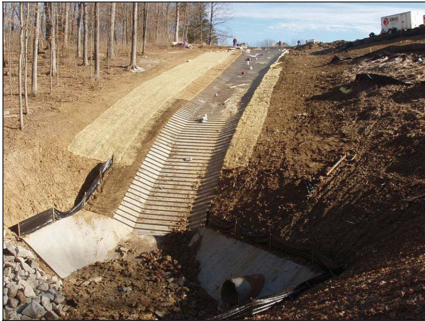
Figure Friendship Village-1. —Overall view of the ArmorWedge auxiliary spillway for the Friendship Village Project nearing completion. The spillway is converging near the top, with three slope changes. The flow will enter an energy dissipating basin shared with the service spillway pipe located to the right in the photo (courtesy of Contech Engineering Solutions, all rights reserved).
