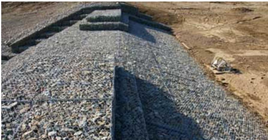
Figure 5-4.—Example of gabion spillway crest structure. (Courtesy of Concrib, all rights reserved)
