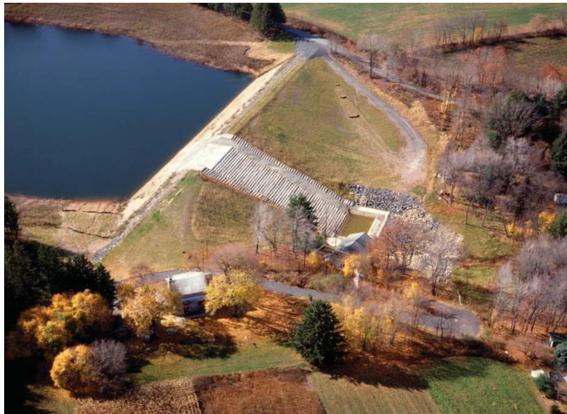
Figure Ringtown-1.—Ringtown Dam and Reservoir (Courtesy of Gannett Fleming, Inc., all rights reserved).
