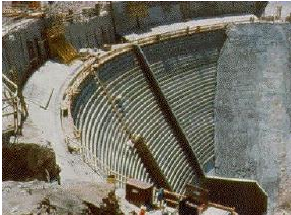
Figure 12-8.—RCC placements followed curvature of existing arch dam, Santa Cruz Dam (Reclamation).
