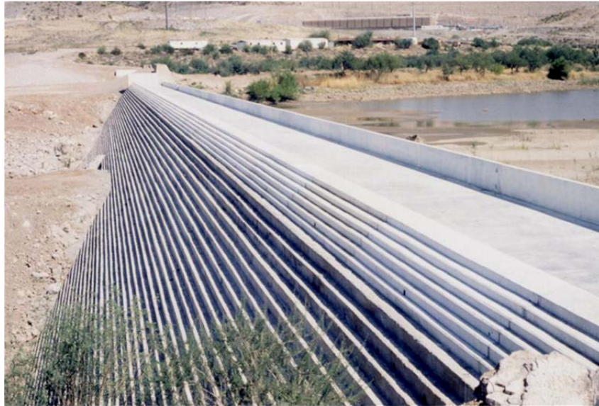
Figure 12-1.—Completed RCC buttress at downstream face of Camp Dyer Diversion Dam in Arizona. Conventional concrete was used for the overflow crest and approach apron. The stepped surface provides energy dissipation for overtopping flows (Reclamation).
