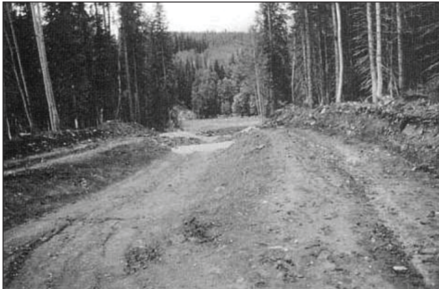
Figure Cottonwood-5.—Preparation of subgrade before geomembrane liner installation in spillway (Reclamation figure republished in Timblin et al., 1988).
