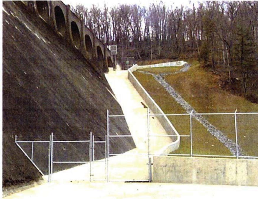
Figure Tygart-2.—Concrete Paving and Channel Along Downstream Left Abutment (Courtesy of USACE)
