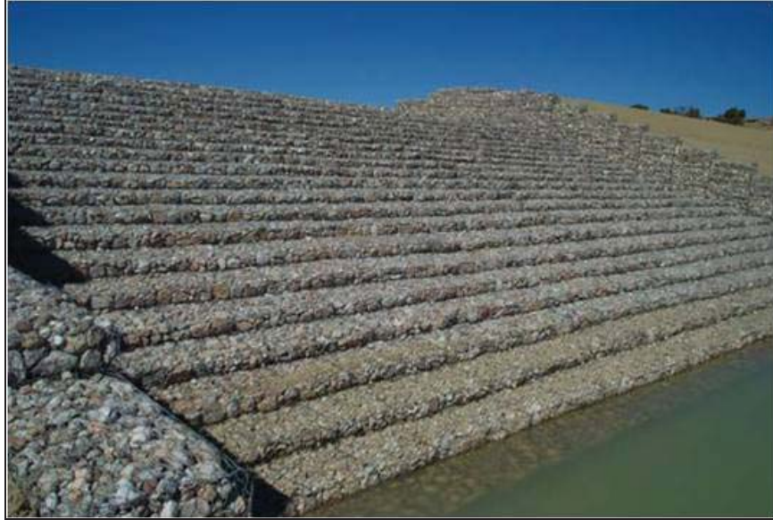
Figure West Cornfield-6.—Completed gabion spillway in 2003 (Courtesy of Maccaferri, Inc., all rights reserved).
