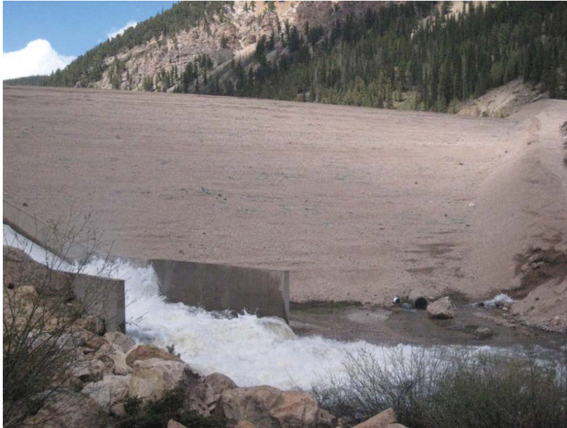
Figure Spring Creek-1.—RCC overtopping protection placed on downstream face of Spring Creek Dam between left abutment groin and right abutment service spillway (shown operating in foreground). (Courtesy of Colorado Department of Natural Resources)
