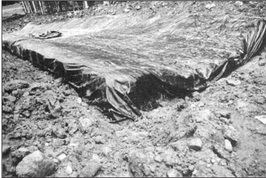
Figure Cottonwood-6.—Section of geomembrane liner installed in spillway before backfilling and compacting anchor trenches (Reclamation figure republished in Timblin et al., 1988).
