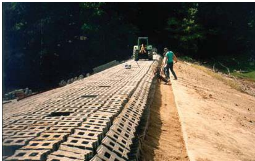
Figure Strahl-5.—View of the upstream trench used to anchor the system at the crest (Courtesy of Contech Engineering Solutions, all rights reserved).
