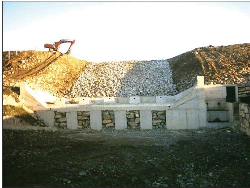
Figure Barriga-7.—Completed flip bucket toe block and drainage with initial grading for block spillway (courtesy of Morán and Toledo, 2006, all rights reserved).
