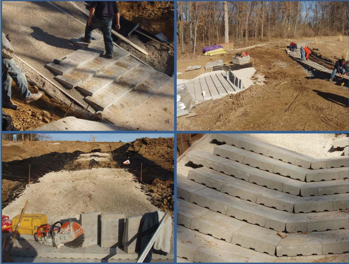
Figure Friendship Village-2. — Top left photo is of ArmorWedge block placement over graded bedding material near toe
