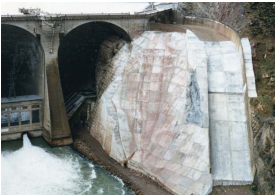
Figure Coolidge-9.—Photo showing finished left spillway concrete overlay and overtopping protection on lower left abutment of dam (Reclamation).
