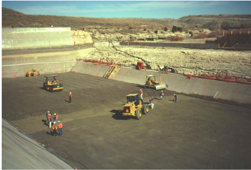
Figure 12-5.—RCC buttress construction within the original spillway plunge pool for Pueblo Dam in Colorado (Reclamation).
