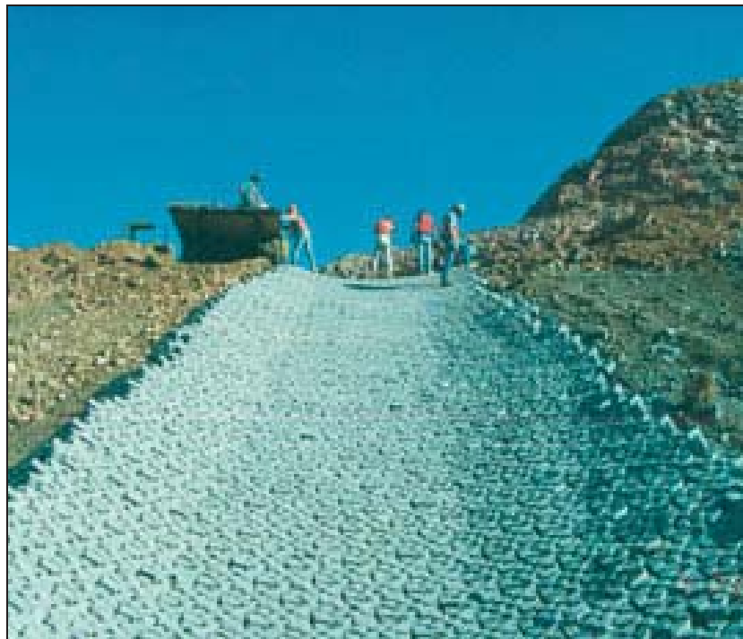
Figure Richmond Hill-5.—Nearly completed downchute constructed of interlocking ACBs. The upstream end of the Tri-lock mat was not anchored as it would be in today's installations. The sides of the mat were anchored into the overburden stockpile cover material (Courtesy of Jacobs et al., 2004, all rights reserved).
