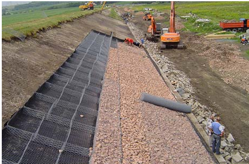
Figure 5-6.—Gabion erosion protection on slope of embankment. Zamoly Reservoir, Hungary (Courtesy of Pannon Gabion Kft, all rights reserved).
