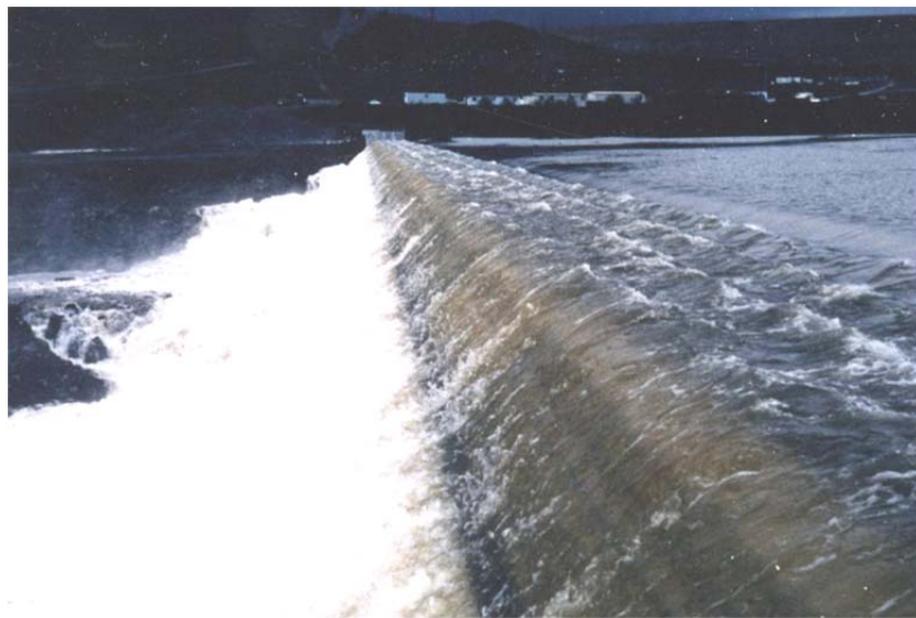
Figure 12-2.—RCC buttress for Camp Dyer Diversion Dam during overtopping in January 1993 (Reclamation).
