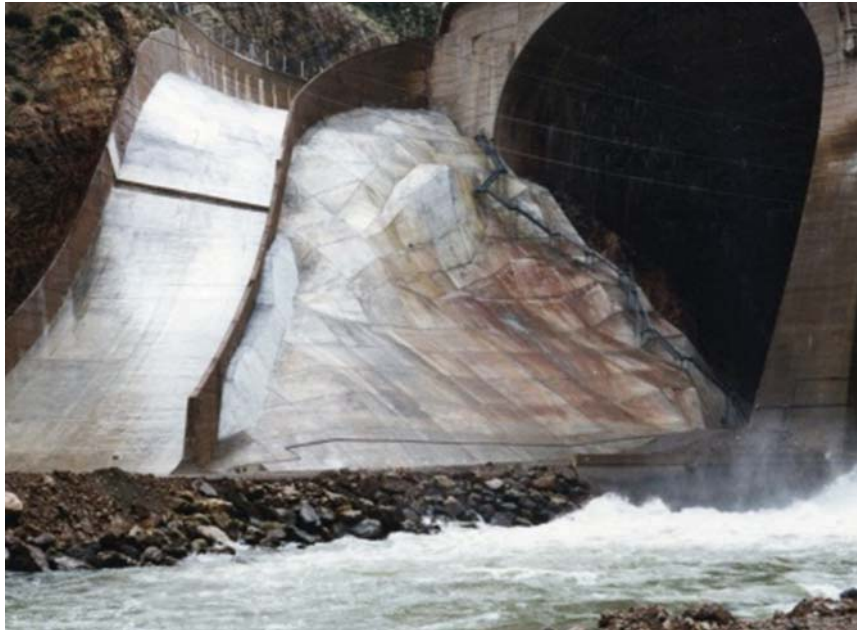
Figure Coolidge-8.—Photo showing finished right spillway concrete overlay and overtopping protection on lower right abutment of dam (Reclamation).
