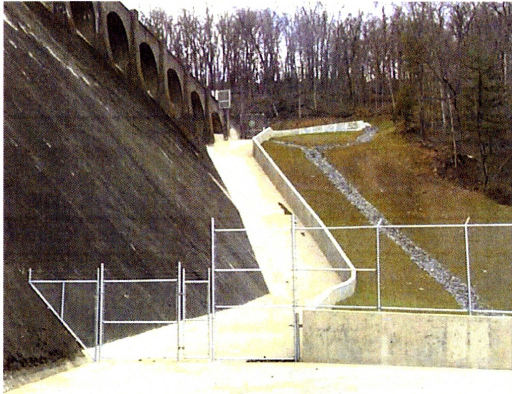
Figure 13-5.—Concrete channel using guide wall to convey overtopping flows (USACE republished in Zaitsoff, 2003).
