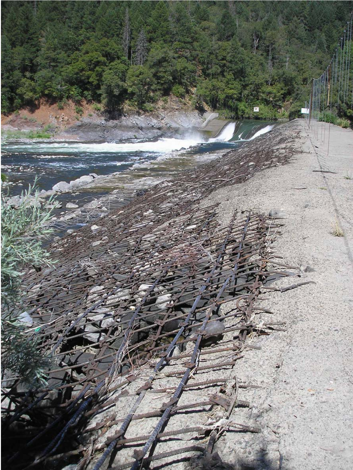
Figure 7-2.—Pit No. 7 Afterbay Dam, looking at downstream face, toward right abutment spillway. Dam crest has been capped with concrete. (Reclamation, 2007, courtesy of Jared Vauk).
