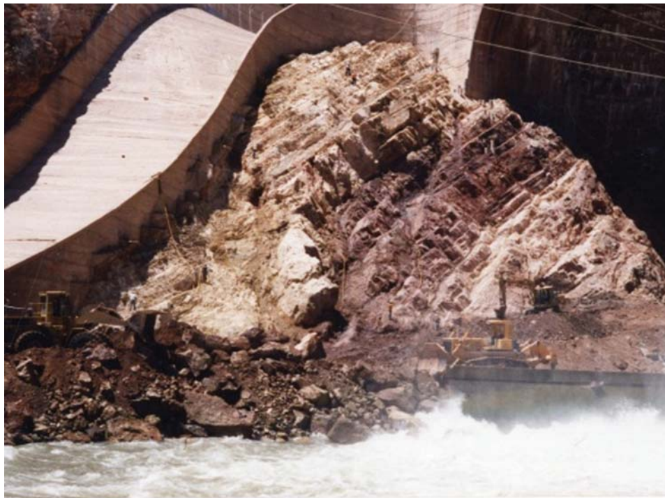
Figure Coolidge-7. —Photo of lower right abutment of dam and right spillway chute. Right abutment overtopping and excavation and cleanup in progress (Reclamation).
