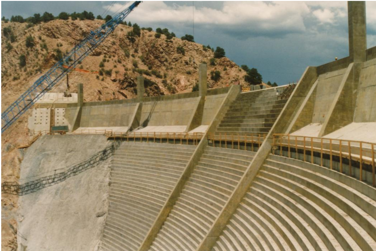
Figure 12-3.—Concrete overtopping protection for Santa Cruz Dam in New Mexico. Splitter piers were provided for overtopping of the entire dam crest (Reclamation).
