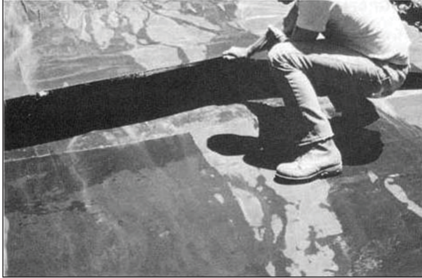
Figure Cottonwood-18.—The overlapped seams were inspected after the test. The geomembrane liner and the earthen materials were all dry under the overlapped areas (Reclamation figure republished in Timblin et al., 1988).
