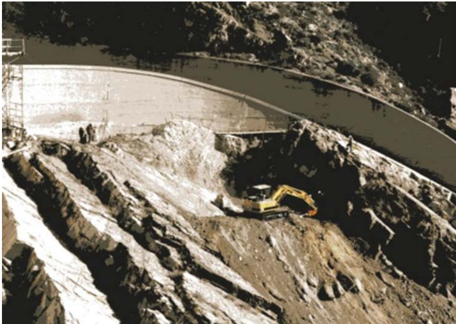
Figure Coolidge- . —Photo of left abutment before any material was excavated or vegetation removed (Reclamation).
