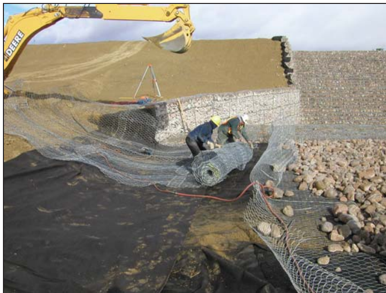
Figure West Cornfield-3.—Unrolling gabion mats in stilling basin (Courtesy of Maccaferri, Inc., all rights reserved).
