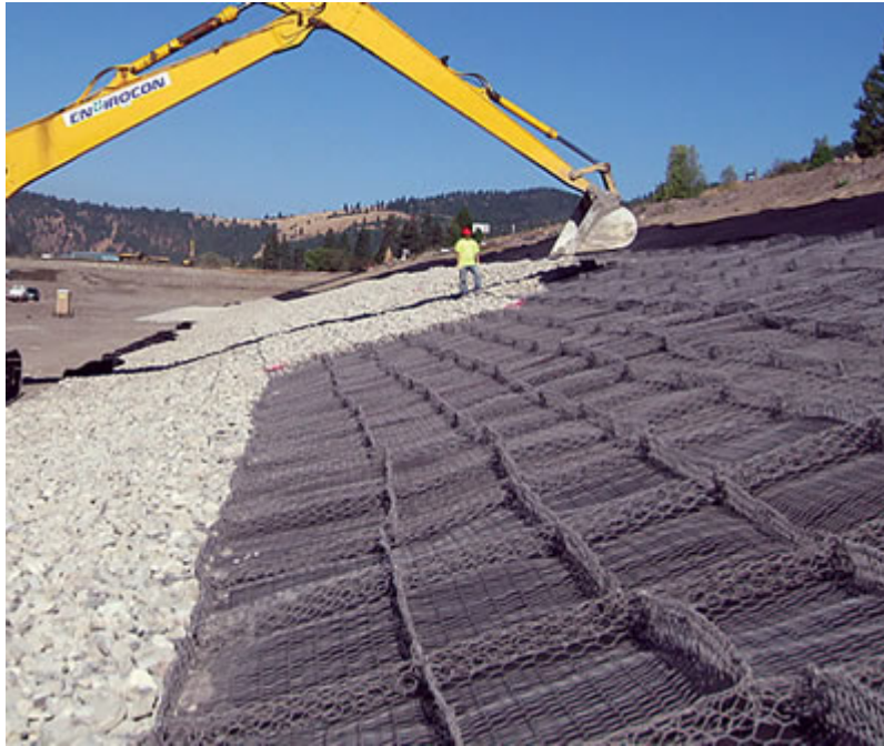
Figure 5-13.—Gabion baskets on slope being filled with rock, Milltown Dam Removal project in Milltown, Montana (Courtesy of Envirocon, all rights reserved).
