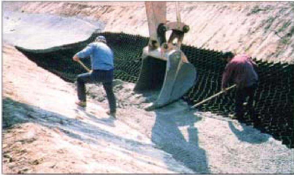
Figure Empire-1– Installation of the GeoWeb CCS with concrete infill for Empire Landfill (courtesy of Presto Geosystems, all rights reserved).
