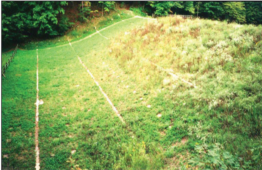
Figure Strahl-7.—Vegetative cover on Strahl Lake Dam overtopping protection (Courtesy of Contech Engineering Solutions, all rights reserved).
