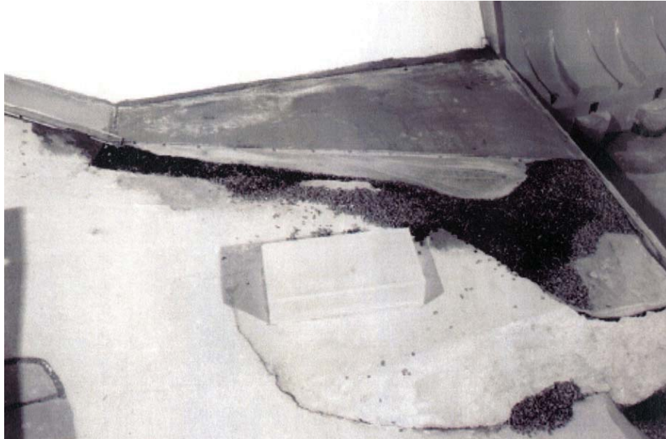
Figure Tygart-3.—Type 2 design, damage resulting from PMF flow for 1 hour (Courtesy of USACE, 1999).
