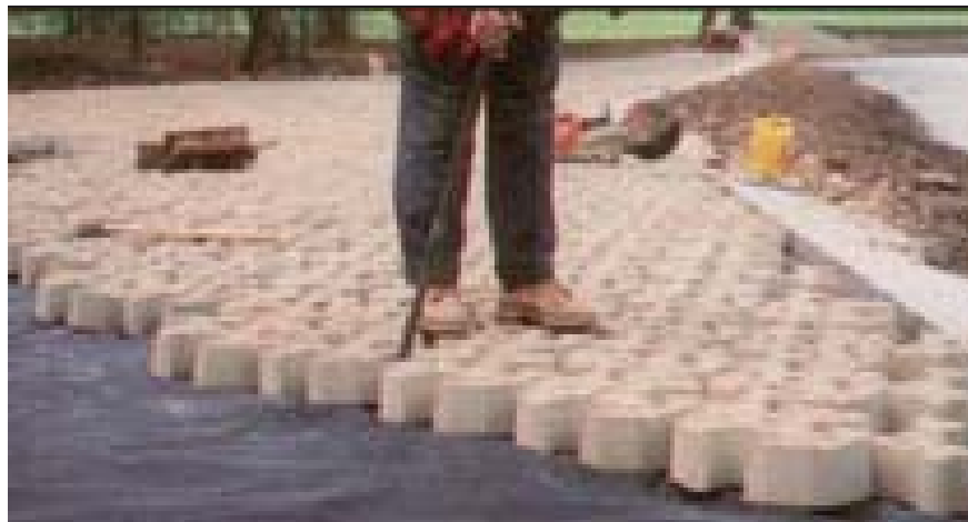
Figure Richmond Hill-3.—Installation of the 40-in-thick ACBs directly over the geotextile prior to backfilling the open space between blocks with topsoil (Courtesy of Jacobs et al., 2004, all rights reserved).
