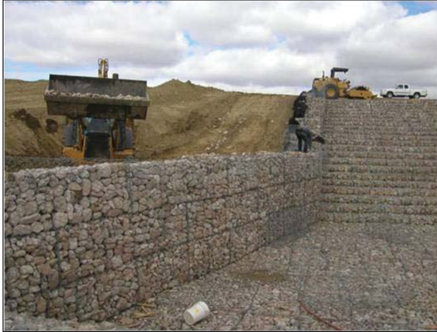
Figure West Cornfield-4.—Constructing stilling basin retaining walls (Courtesy of Maccaferri, Inc., all rights reserved).
