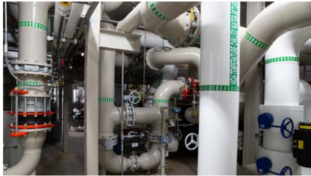
Cooling pipes at an Intel data center in Hillsboro, Oregon.
